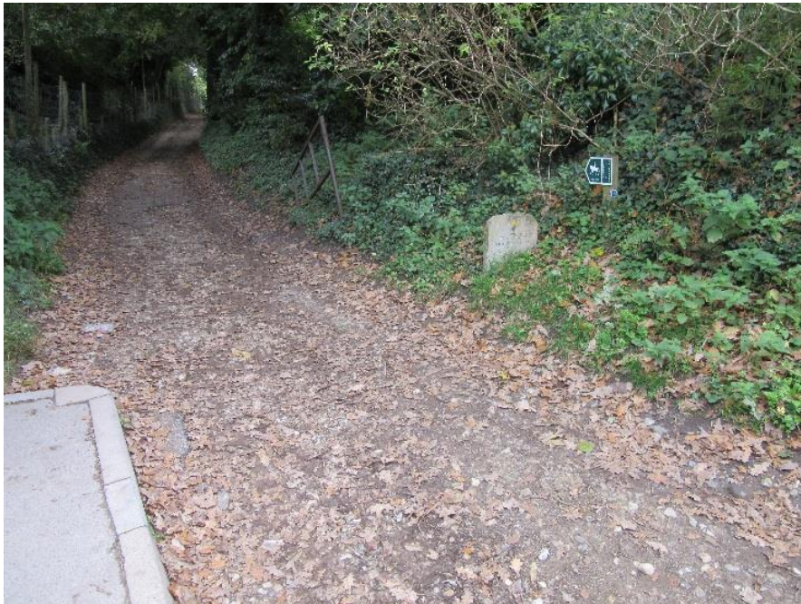
Photo 5. Loose gravel at bottom of LCH-4-S012 BW (29 Sept 2017)
