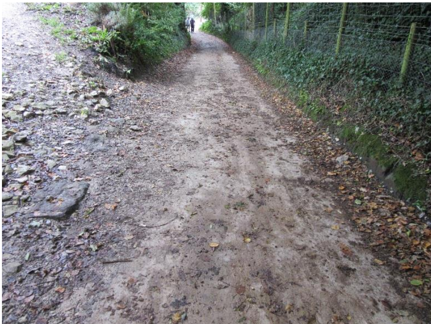
Photo 6. Run-off from adjoining drive-way onto concrete surface (LCH-4-S012 BW) (29 Sept 2017)
