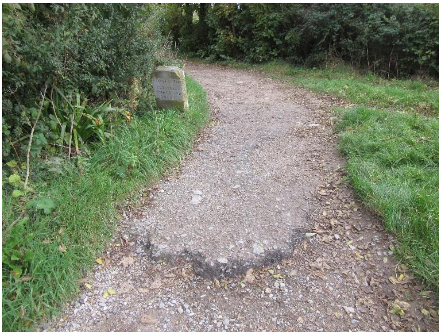
Photo 8. Route section LCH-4-S011 BW – broken tarmac edge (29 Sept 2017)
