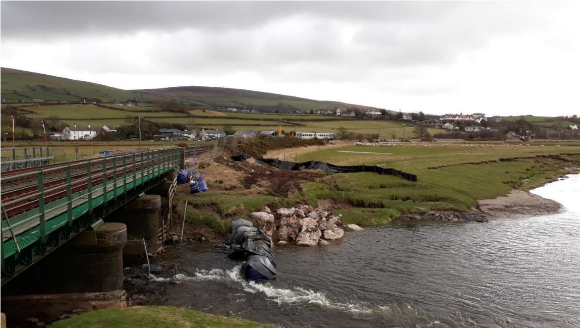
2. Existing rock armour needs work to allow improved footpath access.
