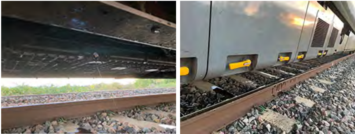
Figure 10: The oil leak under the second vehicle and oil contamination on the rail (left image courtesy of Hitachi Rail and right image courtesy of Network Rail)
