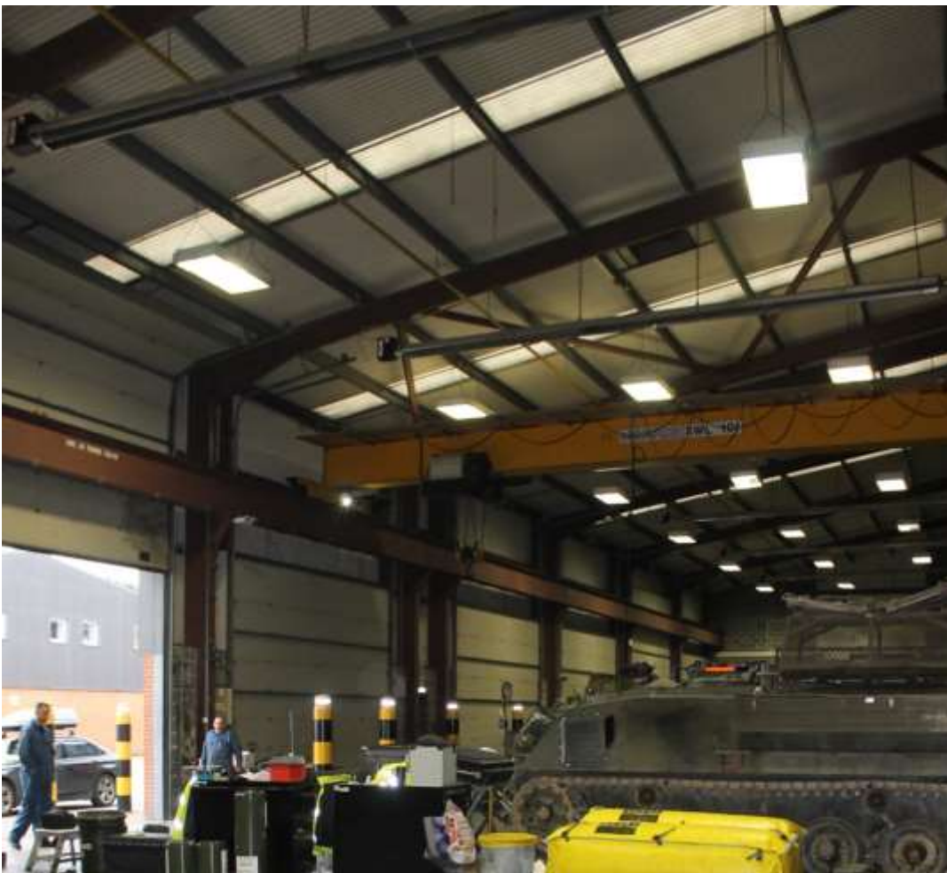
Photograph B. Examples of luminaires suspended and centrally where the luminaire fell.
