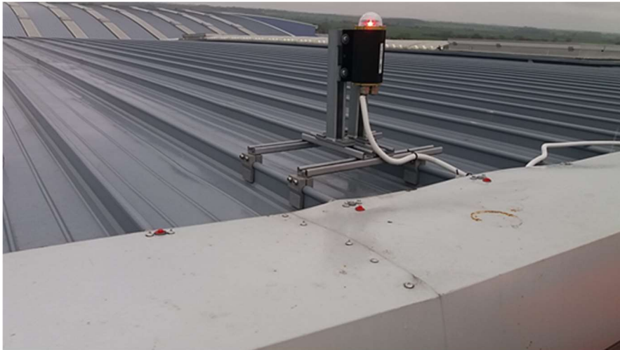
Figure 2: The fixings for the grey cladding are not visible to an inspector
