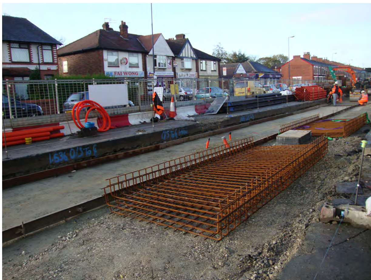
Figure 14: Construction work on Droylsden Road in November 2011. The location of the accident is at the right of the image (courtesy of TfGM)
