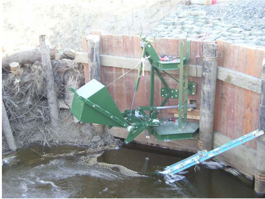
Figure 7.7: Float mechanism for an MTR gate at Schneider Creek, Washington State, US. Photograph courtesy of Tom Slocum, Washington Conservation District's North West Region Engineering Program.
