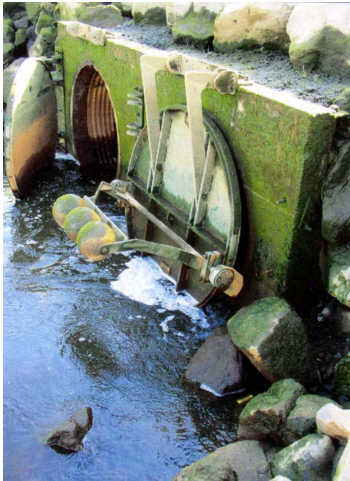
Figure 6.16. The nearer flap is fitted with a mitigator fish passage device, which holds the door ajar until the rising tide lifts the floats. The further culvert has a side-hinged gate, converted from a top-hinged flap – the remains of the flap hinges can be seen on top of the concrete bulkhead. Photograph courtesy of Guillermo Giannico, Oregon State University.
