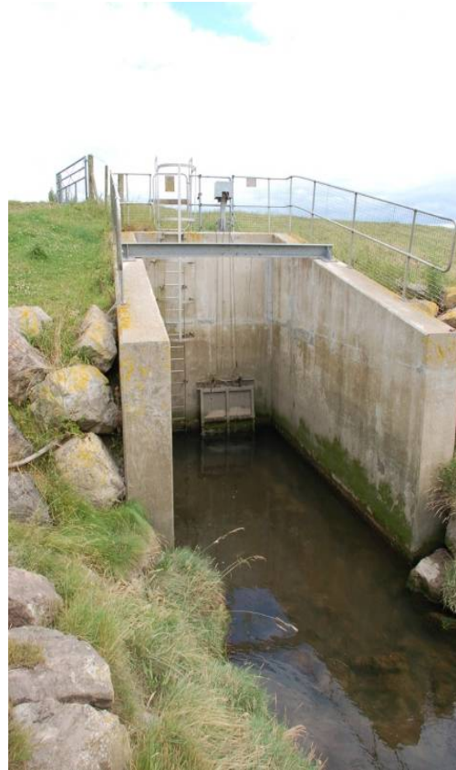
Figure 7.20: A flap gate at Warth Brook, Gloucestershire. The gate's correct invert level allows continuous opportunity for fish passage.
