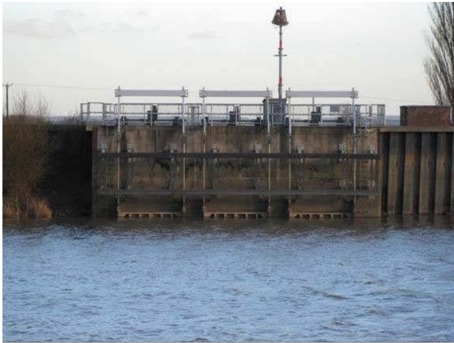
Figure 7.26: Counter-balanced gates on the Bottesford Beck, Scunthorpe.
