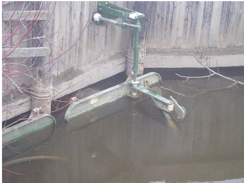
Figure 7.8: Gate actuating mechanism for an MTR gate at Schneider Creek, Washington State, US. The door is being held open. Photograph courtesy of Tom Slocum, Washington Conservation District's North West Region Engineering Program.
