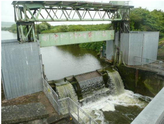
F. Penning weir (door down)
