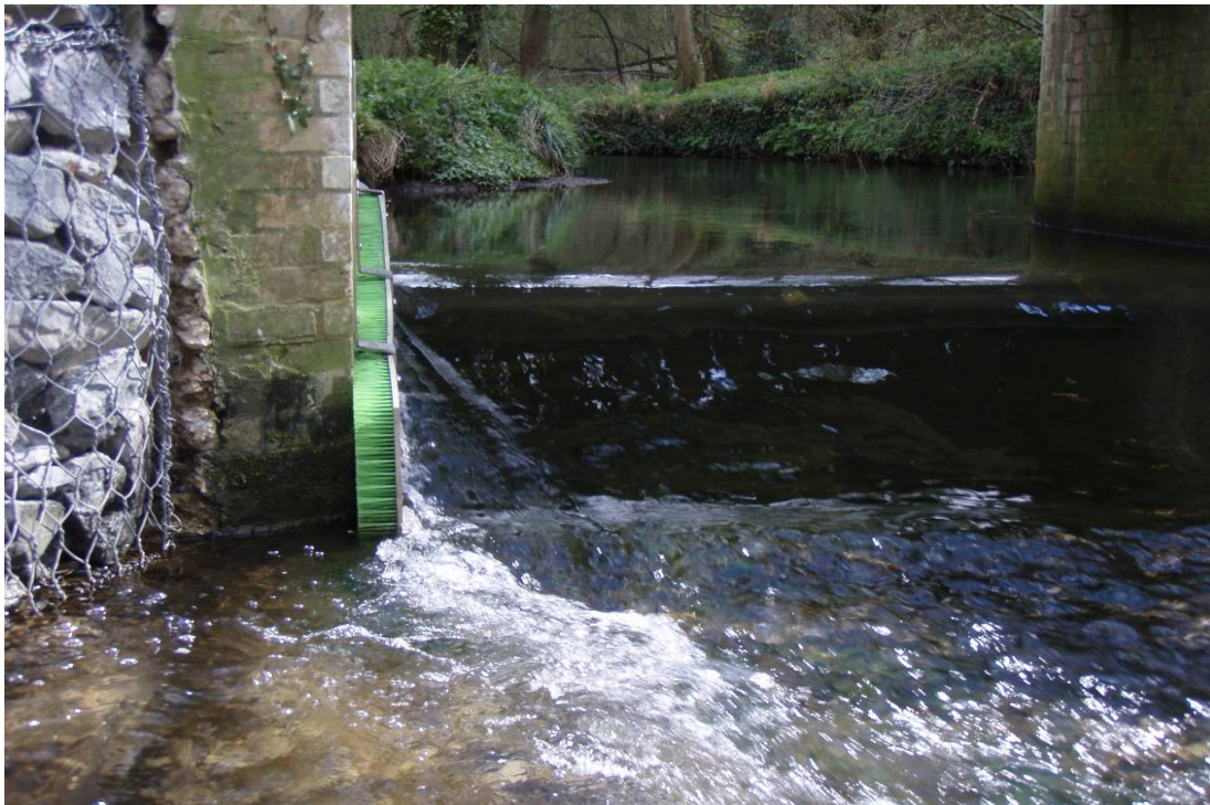
4.12 Downstream view of pass installation at Frog Mill, River Hamble (NGR: 5222 1491). Note the area of slack water on left for elver and eel to enter pass.
