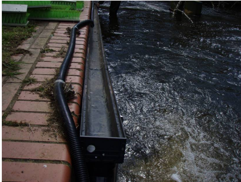
Figure 4.20: UPVC sectional drainage channel, fixed to side wall. (Hole for pumped water supply at near end, with pump tubing ready for fitting.)
