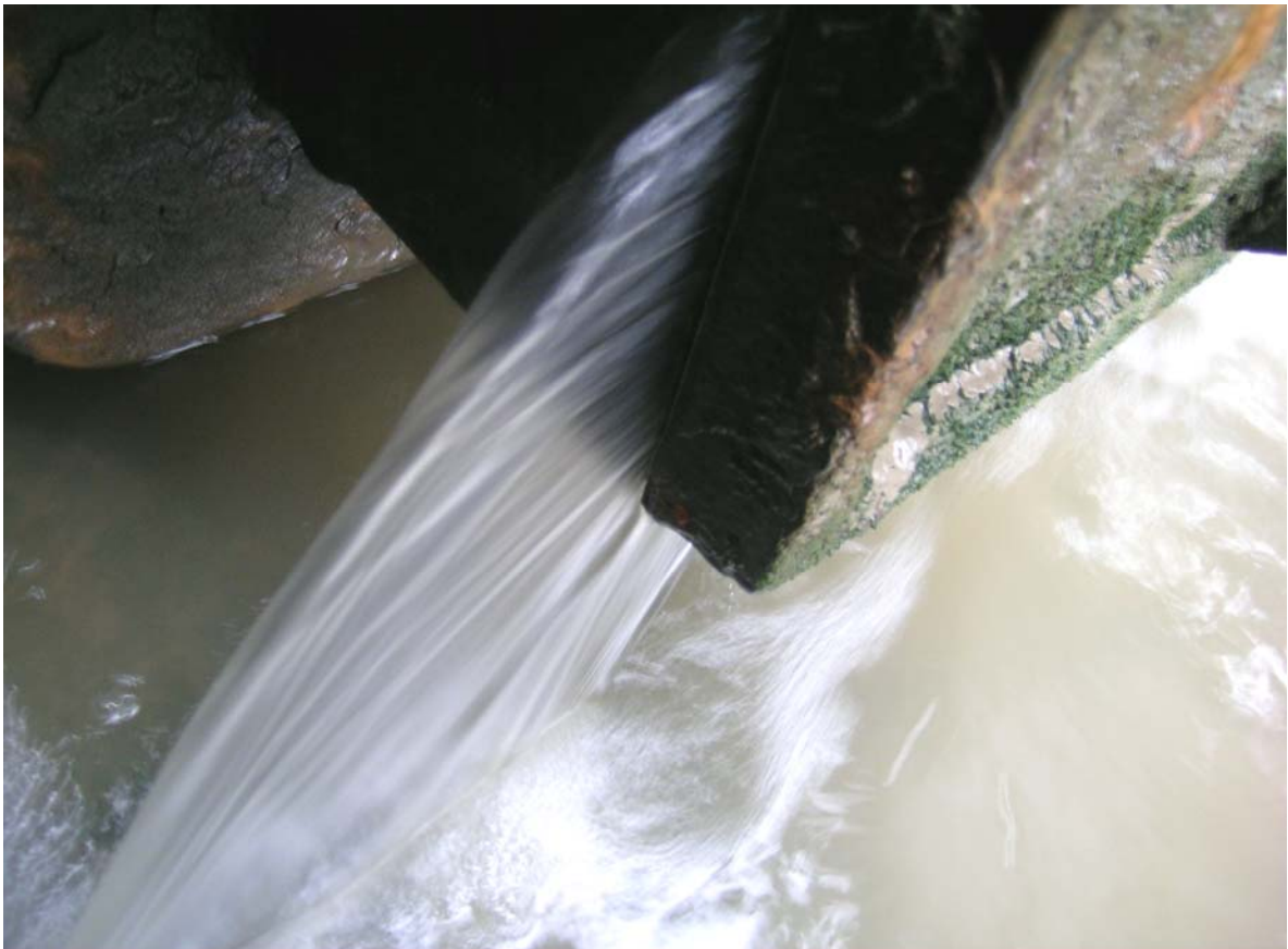
Figure 6.7: Water squirting through the gap of an almost-closed rectangular tidal flap at the mouth of a marsh drainage channel on the Thames Estuary. Even when the tide rises to the bottom of the door, this flow is too fast for elvers to overcome. As the velocity starts to fall, the gate shuts.
