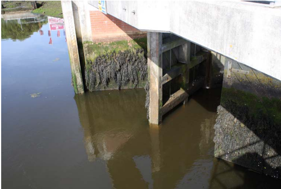
Figure 6.3: The estuary of the River Lympington in Hampshire. These tidal doors are in an open position. The tide has started to flood. The picture shows noticeable landward flow through the structure (towards the right of the picture). A few minutes later, as the landward flow increased, the doors slammed shut.
