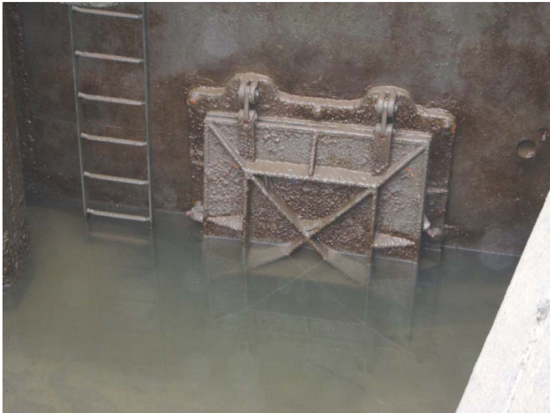
Figure 6.9: The outer flap in the structure shown in Figure 6.8. Note the two plastic bottles jammed in the flap which prevent the flap from closing completely. Were this a single flap, the jammed bottles would allow some landward flow and the passage of elvers. However, the presence of a second flap a couple of metres behind this one prevents this.
