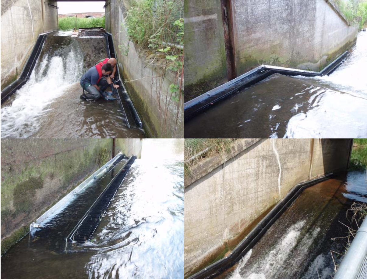
Eel pass at Stapleford Mill weir, on the River Gowy: under construction and completed.
