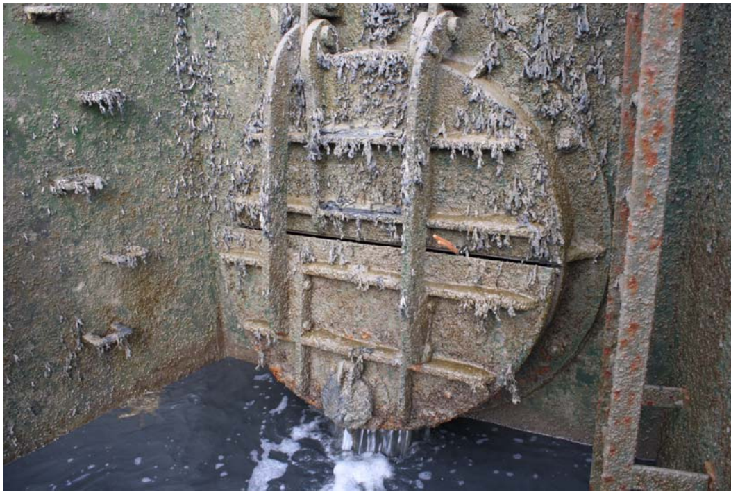
Figure 7.10: Tidal flap at Maydays Farm, Essex. This is an interesting installation as the flap is separately hinged in two halves. The lower half is fitted with a small 'cat-flap', presumably designed to operate at very low flows. However this cat flap, which is made of cast iron, is too heavy to make a useful contribution to elver passage.
