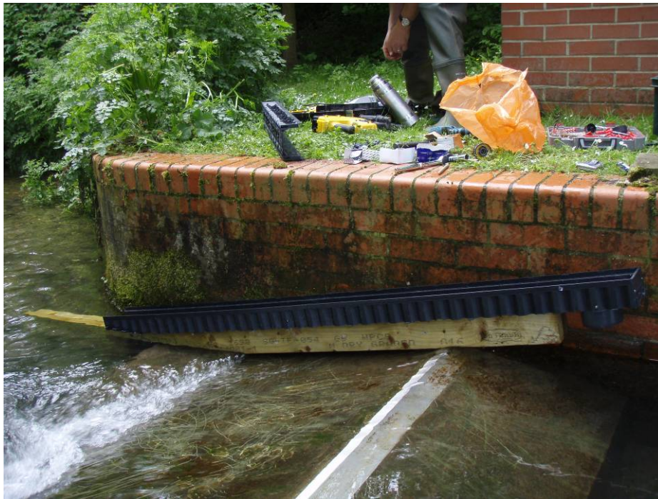
Figure 4.18: Crawling gutter under construction. These curved wing walls are found on many gauging structures. (Note the layer of fast-moving water on the downstream weir face and the clean, debris-free surface. Elvers and eels would be unable to swim through this structure.)
