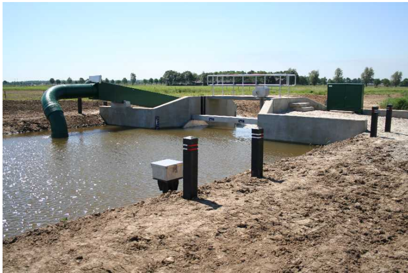
Figure 7.31: Newly constructed siphon pass at Hertogswetering near Berghem (Brabant) in May 2006.
