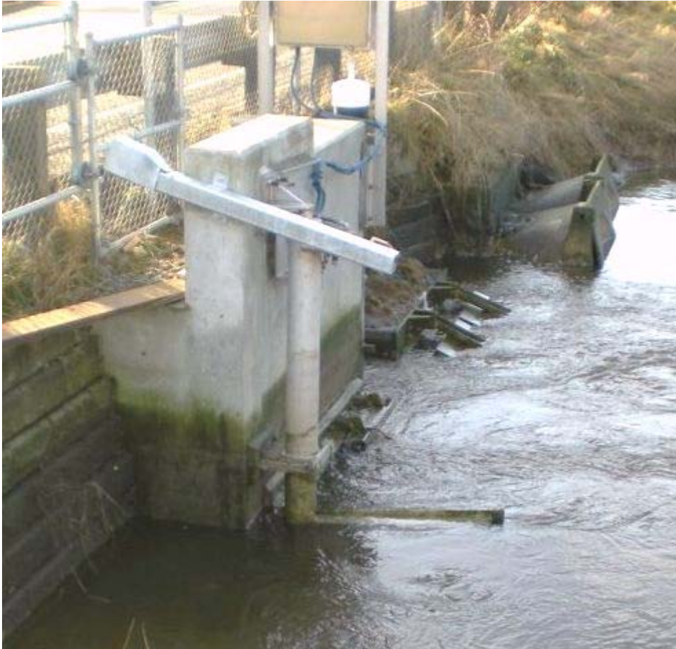
Figure 7.9: Juel Variable Backflow Flap Gate (VBFG™). The gate is fully open, on the ebb tide. Photos reproduced with permission from Juel Tide Gates of Seattle, Washington, US ( www.jueltide.com ).
