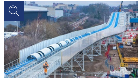
The conveyor installation at Atlas Road.
