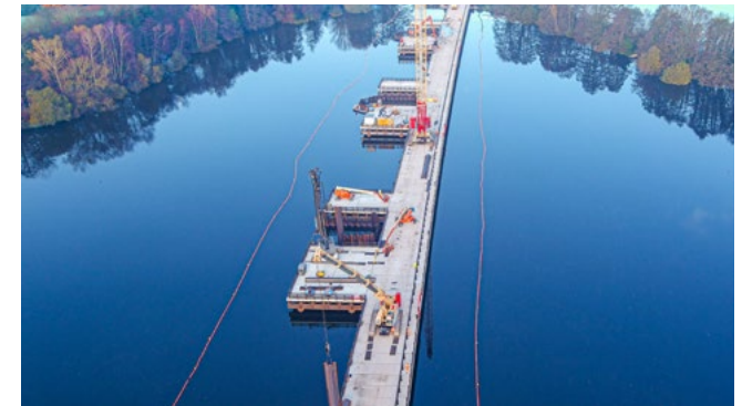
Four jetties have been built to support construction of the Colne Valley viaduct.
