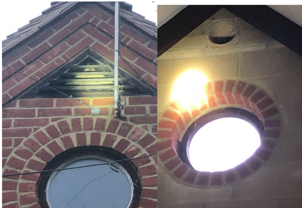
Photographs 4 & 5 Air vents (on both eastern and western gable ends of Building B12). Obstructed and cobwebbing noted.
