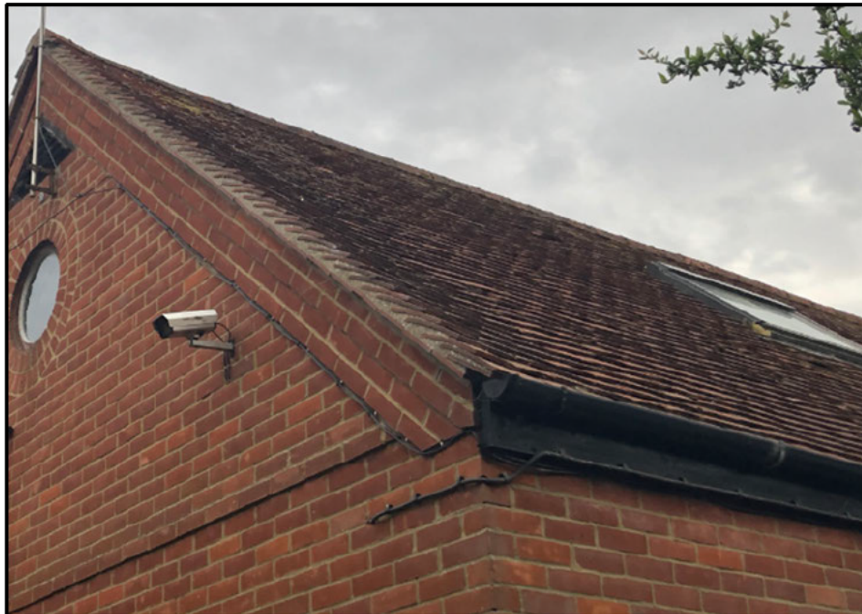
Photograph 1 Northern elevation of Section 1 with skylight. Note roof with tightly fitted tiles across the majority of the roof.
