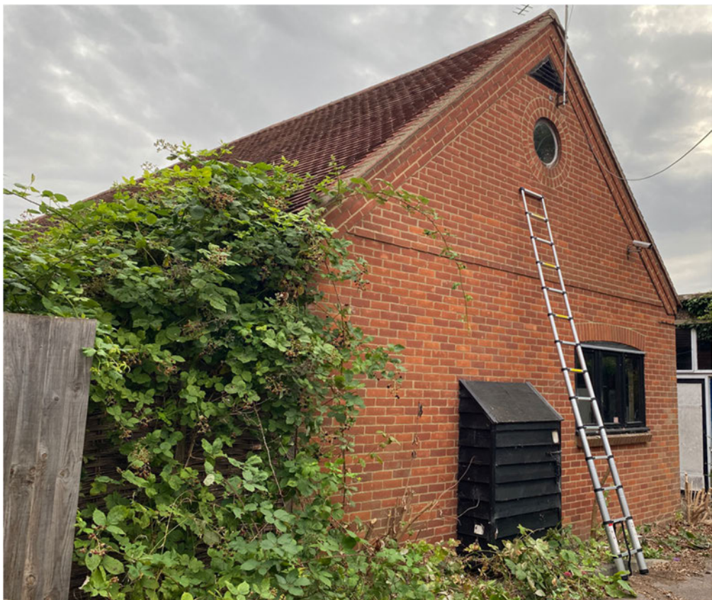
Photograph 3 Southern and eastern elevation of Section 1. Note roof with tightly fitted tiles across the majority of the roof. Note bramble cluttering potential roosting opportunities/clear flight path.
