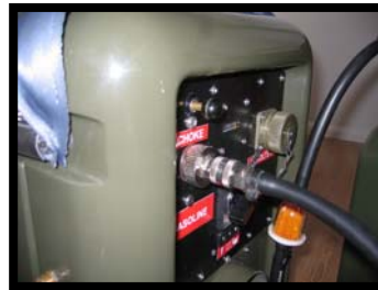
Fig 3 Fuel line connection-generator
