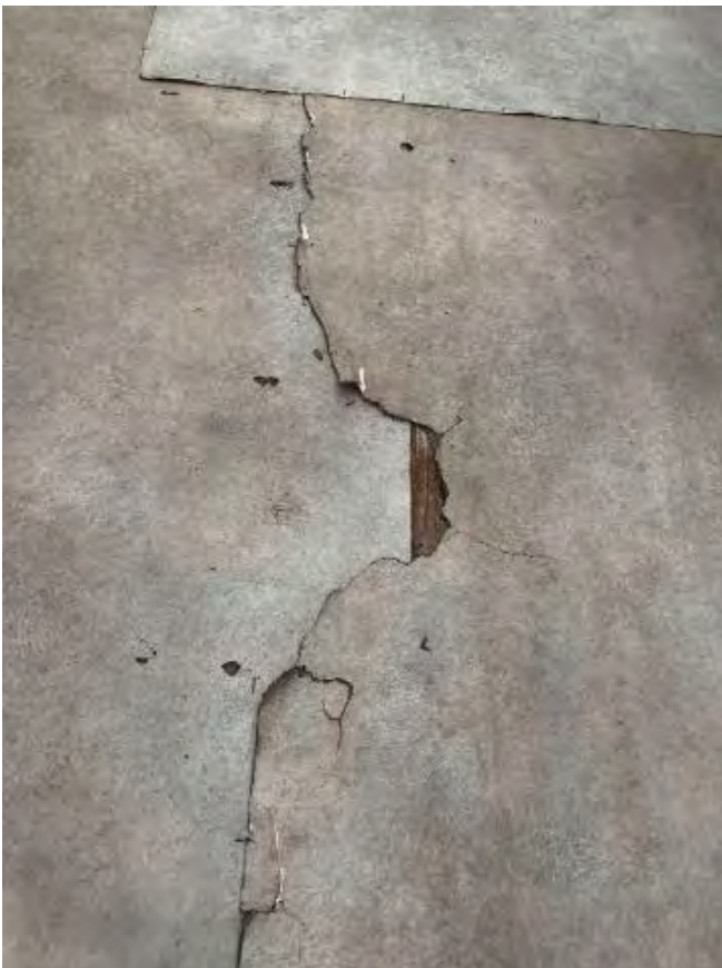
15. Loose/damaged floor covering in TH
