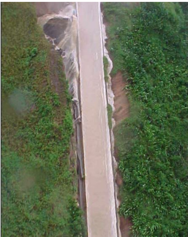
Figure 6: Overtopping of chute walls of El Guapo dam (USBR & USCE, 2019)
