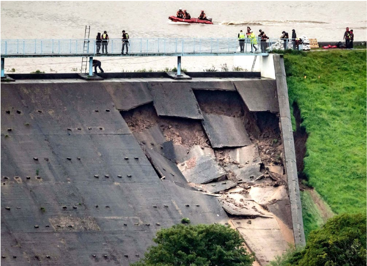
Figure 7: Spillway chute panels collapse into a void at Toddbrook Reservoir (Balmforth, 2020)
