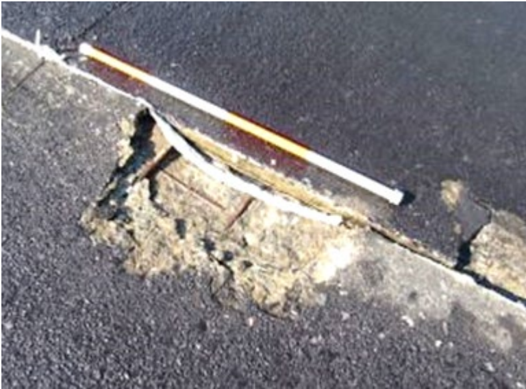
Figure 2: Transverse joint damage (Schweiger and others, 2019).
