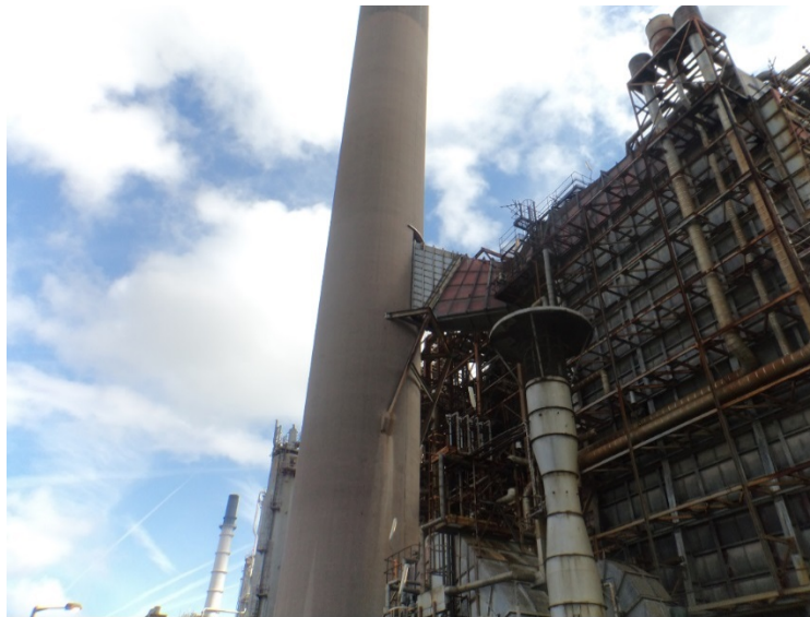
Figure 9.1 CO Boiler Outlet Duct & Stack
