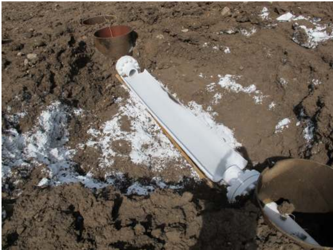
Figure 23: Photograph of the Crater and Ruptured Pipe
