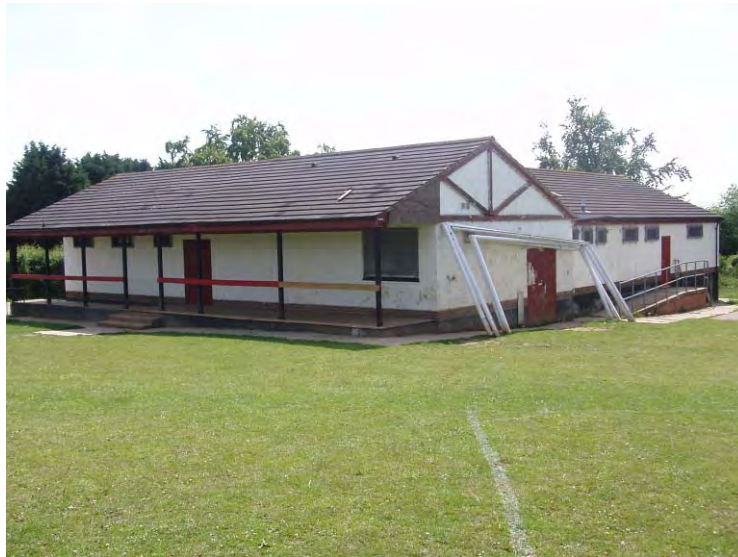
Changing facilities at Herbert Farm Playing Fields - showing signs of wear and tear
