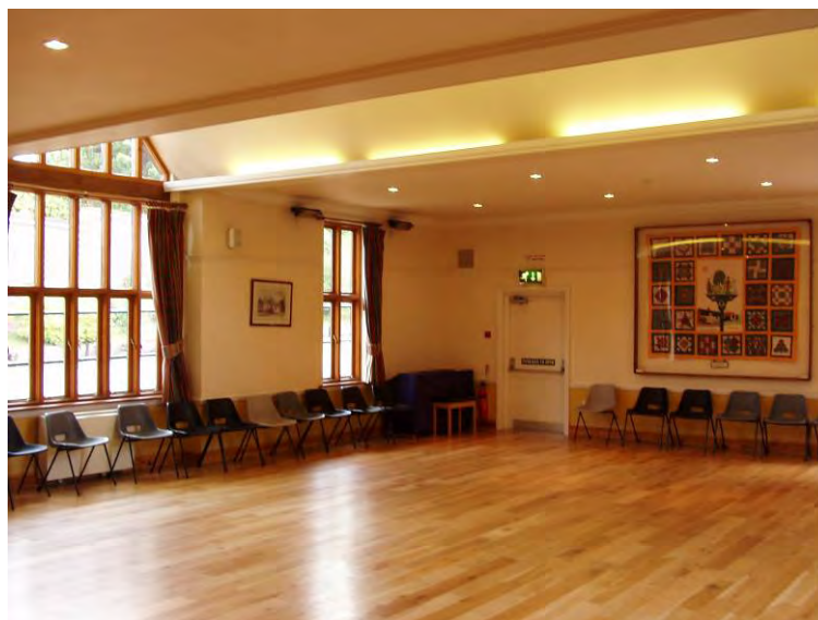
The interior of Ashdon Village Hall showing a good quality floor for recreational level sport and physical activity
