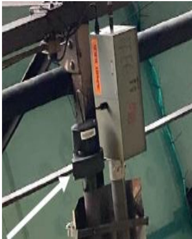
Photograph 3: Fan motor assembly fell from the gas radiant tube heater shown by arrow point
