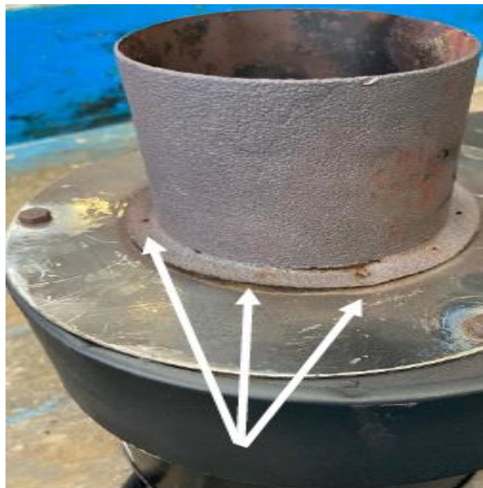
Photograph 4: Fan motor assembly fixing plate and spot-welding points on the spigot that locates onto the radiant tube emitter pipe spot welding is in poor condition, not suitable for further service. A further 60 Fan motor assembly and spigots were checked with a further five been removed due to signs of failure on the spot welding within this establishment gas radiant heater systems.
