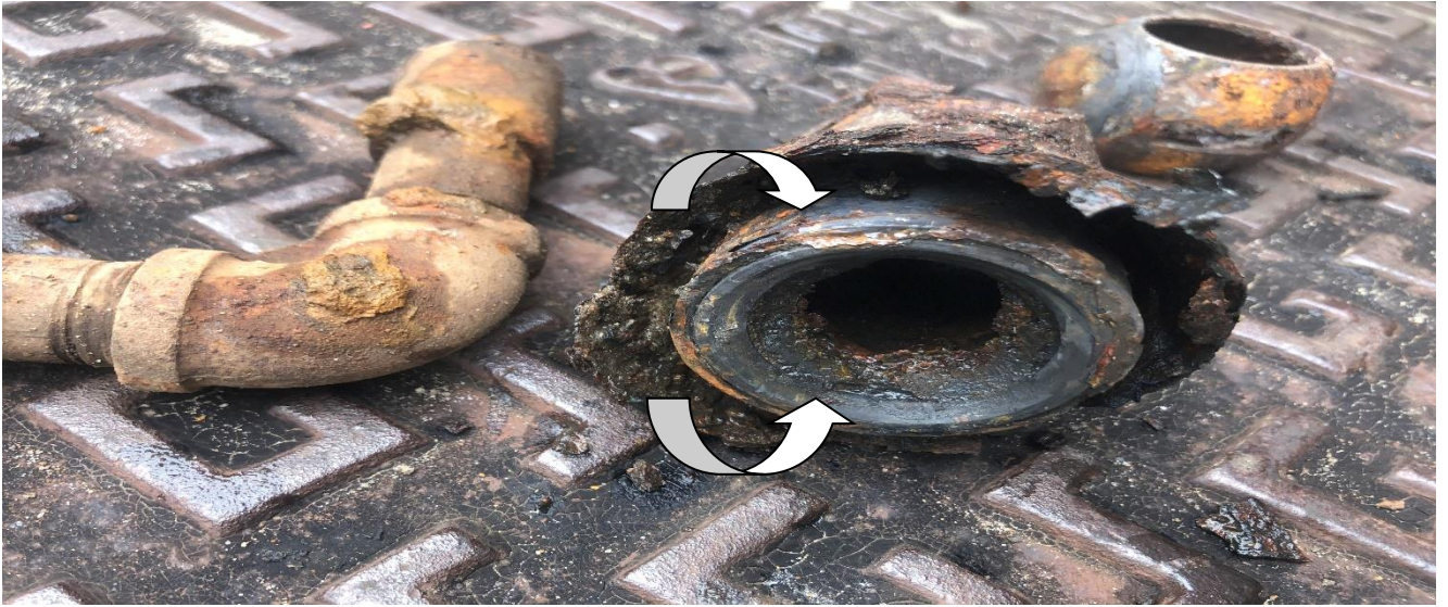
Photograph 1: Failed heating system component corroded through internally and externally
