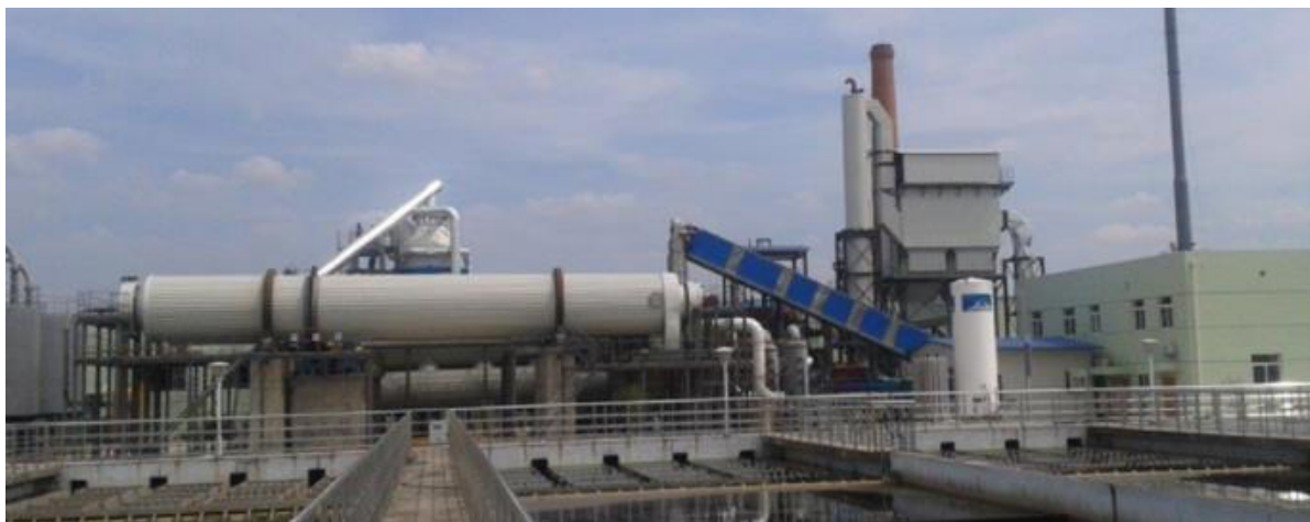
Figure 9: Splainex sewage sludge facility, throughput capacity 200 t/day (Splainex Ecosystems, 2016)
