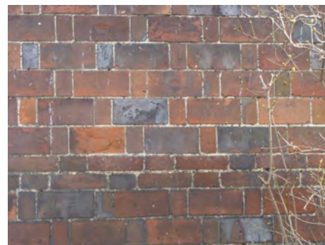
Picture 1.22 Prominent boundary wall in grounds of Elm Grove; unusual rat trap bonding
