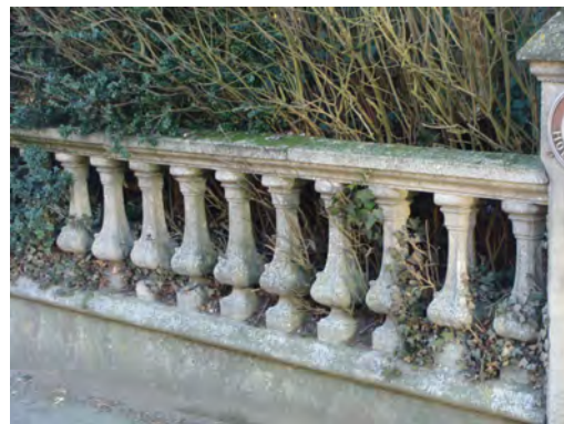
Picture 1.53 Decorative baluster boundary detailing, important for the street scene particularly in West Road
