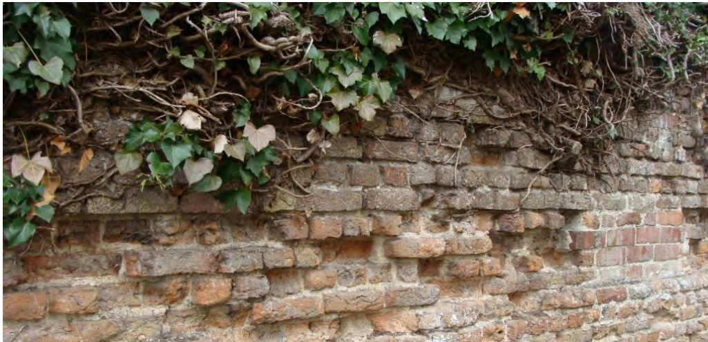
Picture 1.32 Boundary wall to Audley End Estate, an important feature and in urgent need of repair
