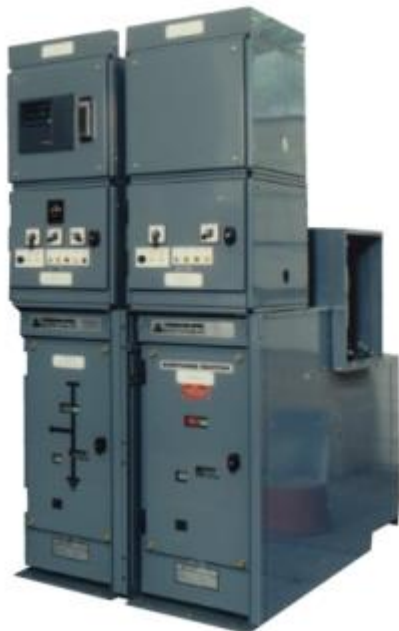
Photograph – 02: Schneider YSF6 switchboard
