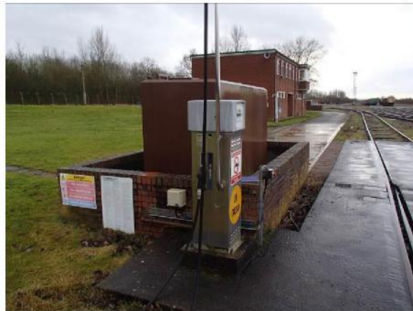
Typical Railway Refueling Installation
