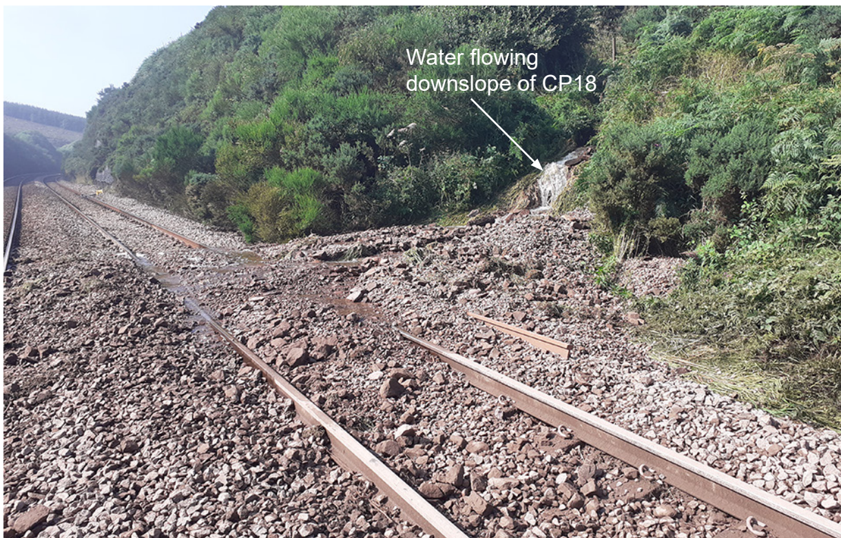
Figure 19: Washout debris on the track approximately 55 minutes after the accident. A short length of scrap rail unrelated to the accident is also visible (Story Contracting)
