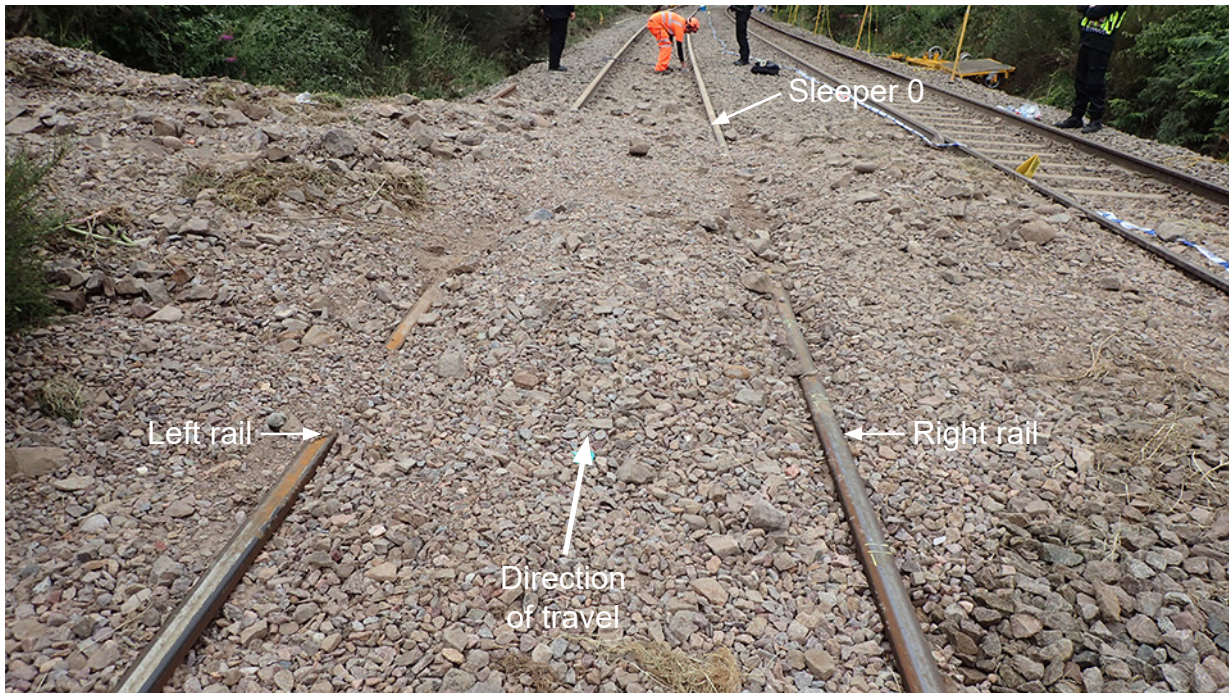
Figure 22: Washout debris covering the track and point of derailment at sleeper 0. Grooves cut by the wheels of train 1T08 through the debris are visible
