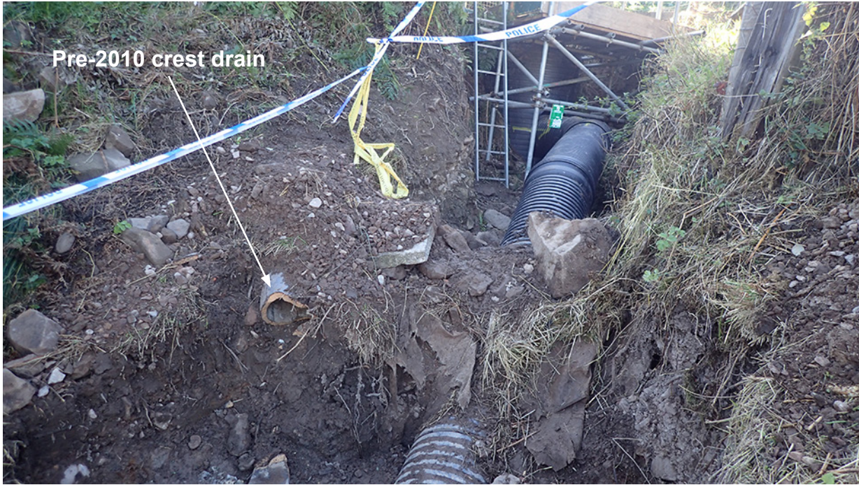
Figure G.4: Image looking upslope from near CP19 towards CP18 showing damaged end of pre-2010 crest drain close to the as-designed position of CP18. Photograph taken during post-accident investigations with scaffolding over as-built position of CP18 visible in background
