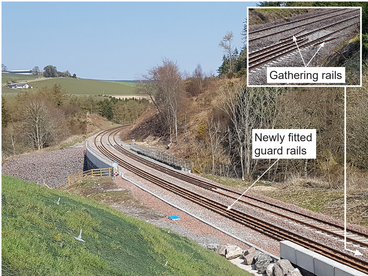
Figure 86: Guard rails fitted post-accident at bridge 325. The gathering rails are positioned at the start of the guard rails to the right of the main picture
