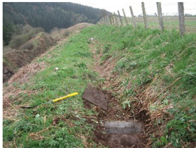
Figure G.1: Pre-2010 crest drain catchpit between CP10 and CP16 showing drain close to the cutting crest in 2010 (Carillion)
