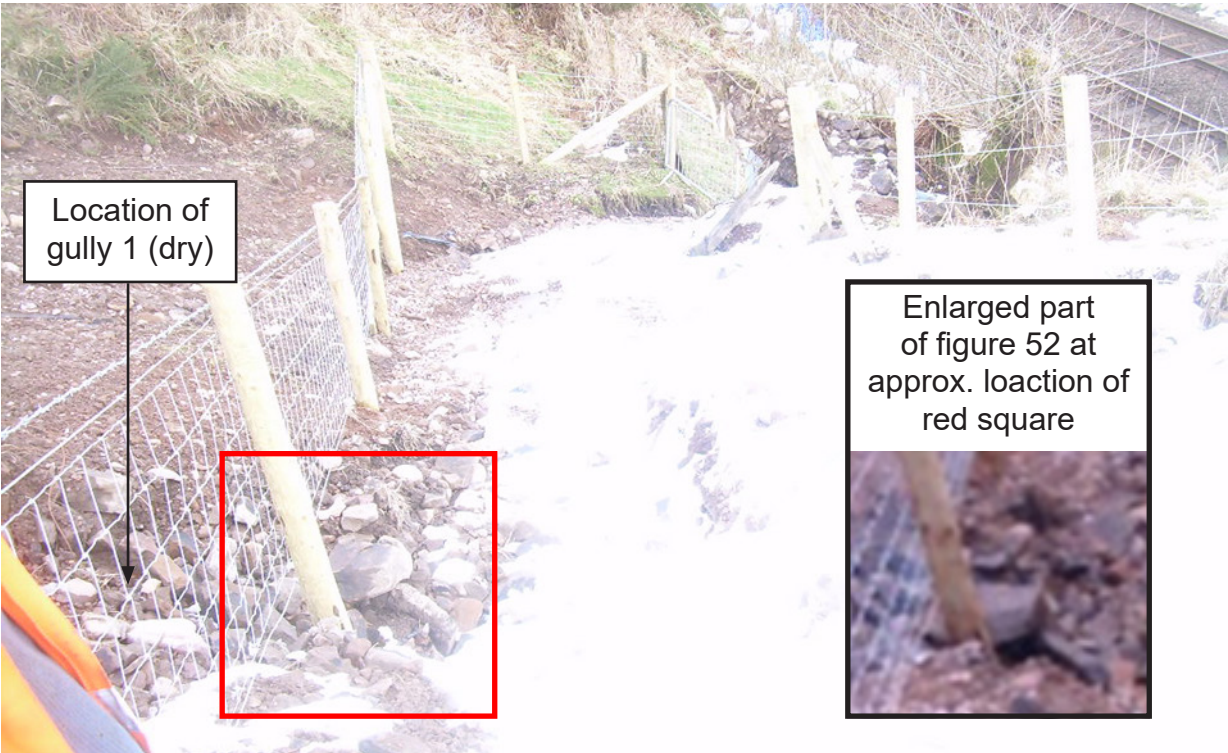
Figure 53: Surface of drain in light snow looking towards CP18 and railway in March 2013 during an inspection of the completed works (Network Rail). The original image is over-exposed
