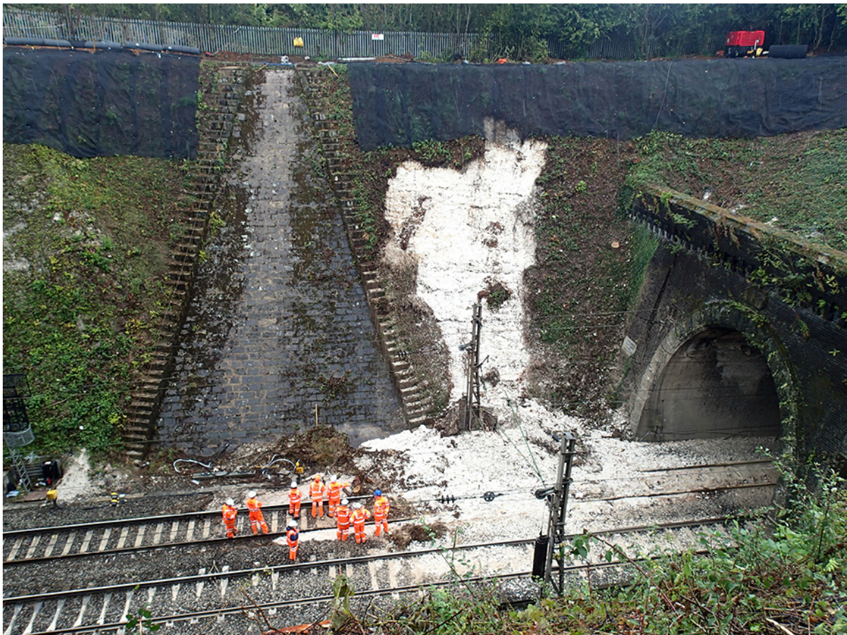
The landslip at Watford tunnel, September 2016
