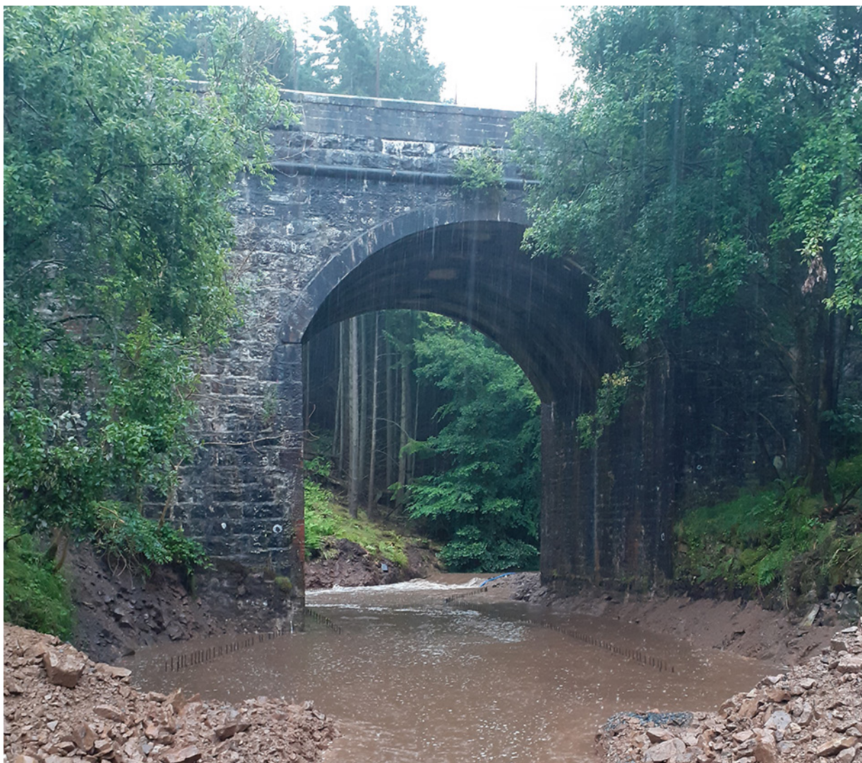
Figure F.4: Down-side elevation of bridge 325 at 08:19 hrs on 12 August 2020, shortly before the accident (Story Contracting)
