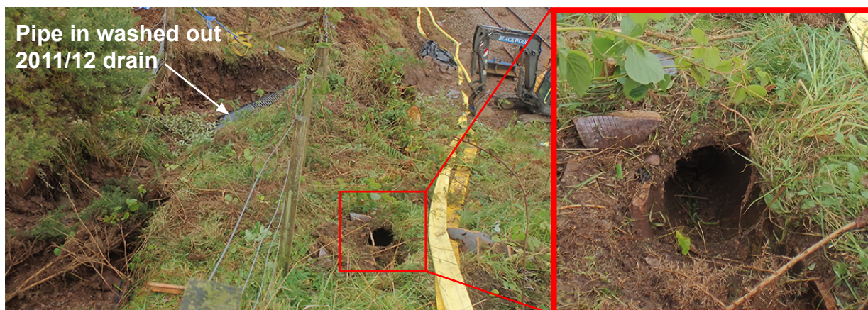
Figure G.3: Break in pre-2010 crest drain near top of washed out section of 2011/12 drain looking downslope with railway visible in top right-hand corner of image
