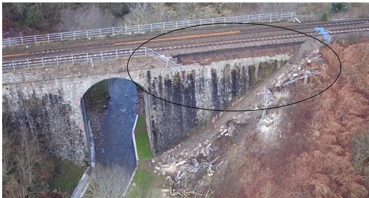
Figure M.1: South-east corner of bridge 328 following the failure of part of its parapet wall on 15 January 2021 (Network Rail)
