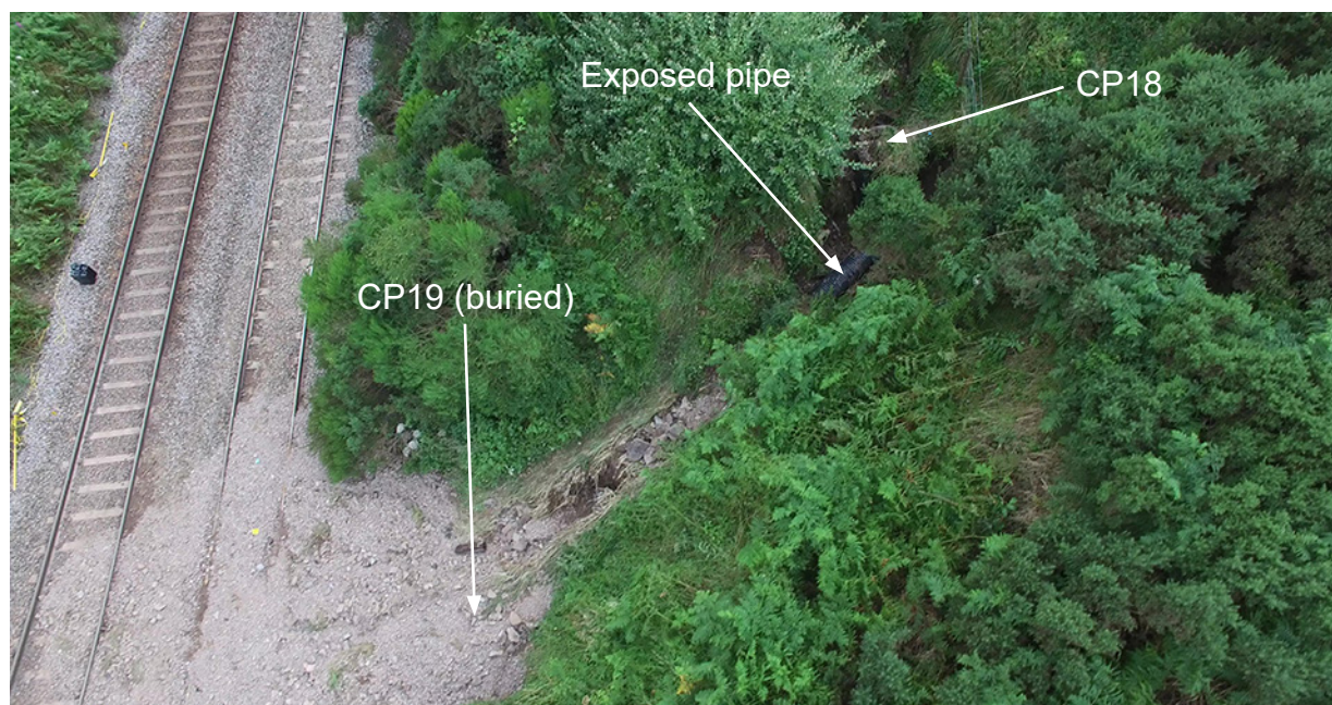
Figure 4: Washout debris on the track
