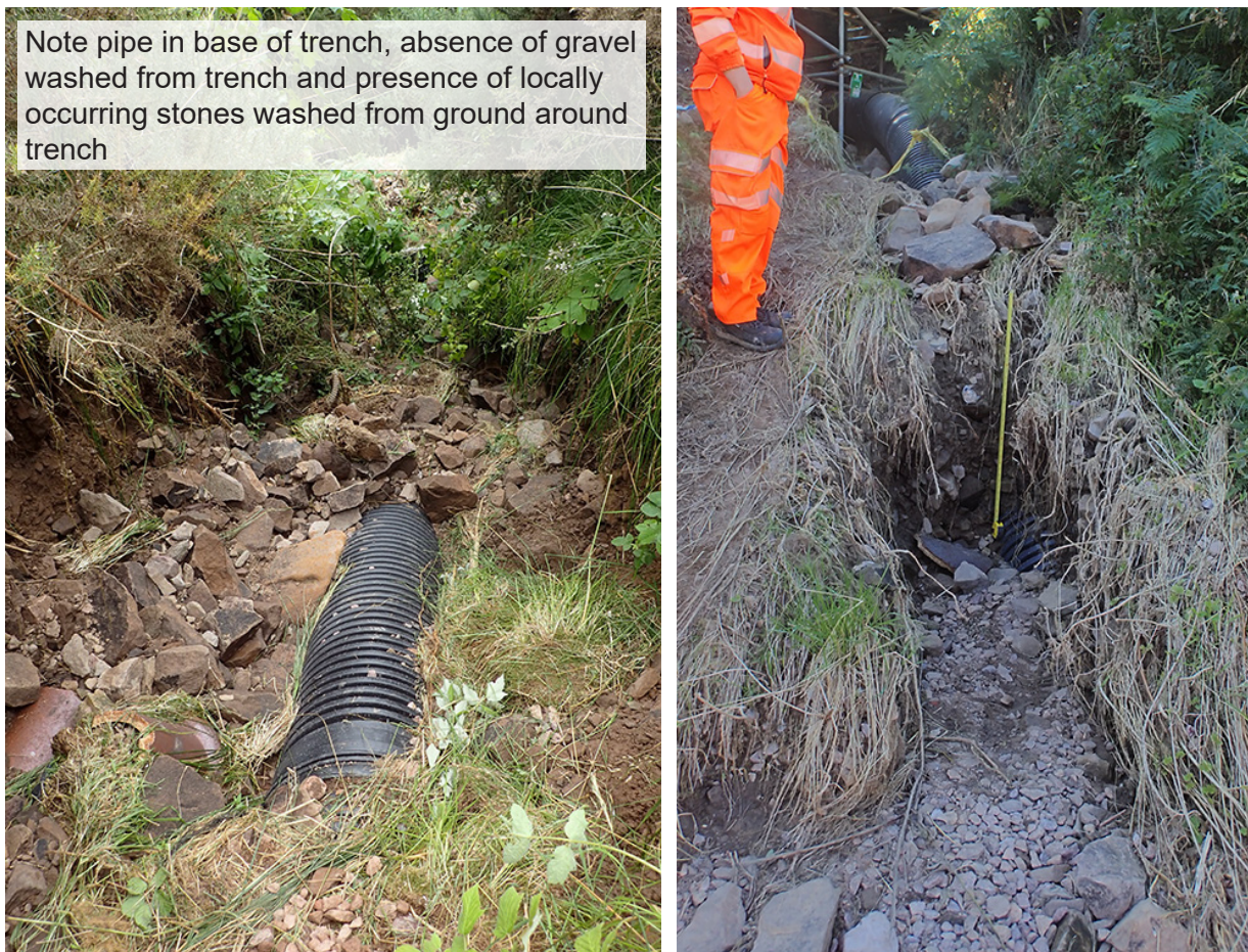
Figure 18: Washout upslope of CP18 (left image) and partial washout downslope of CP18, both images facing towards CP18
