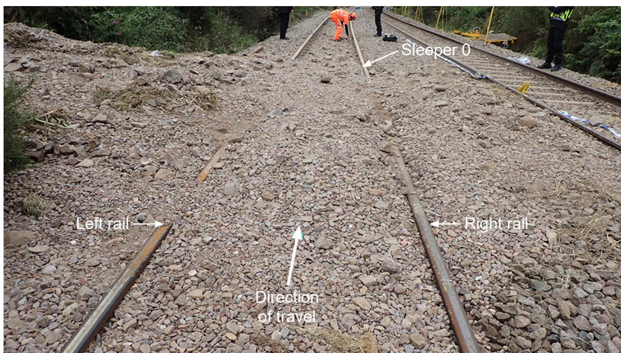
Washout debris covering the track
