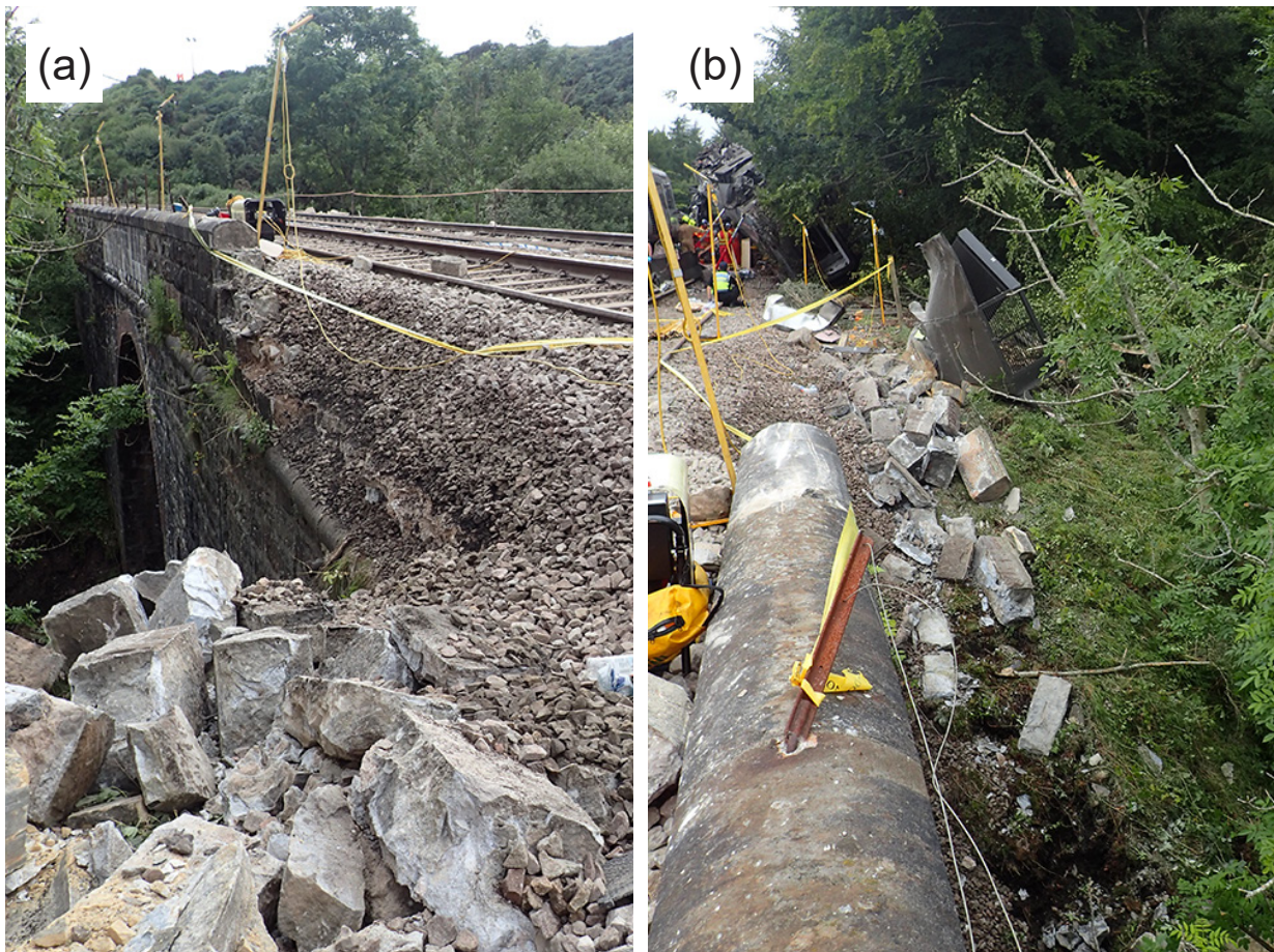
Figure F.8: Up-side parapet damage (a) looking south and (b) looking north
