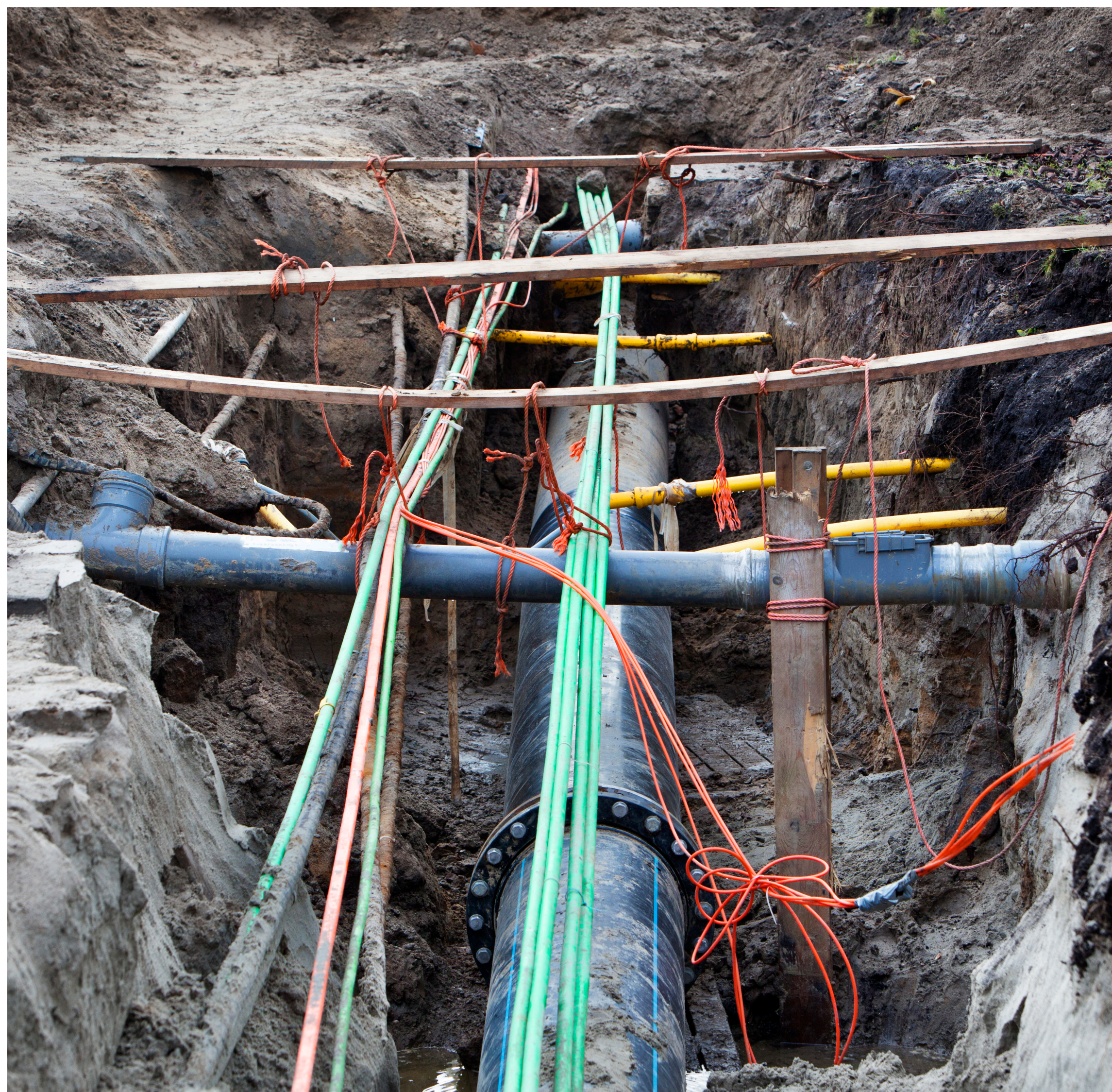
Crowded subsurface beneath a road in north London showing gas, water, electricity and telecommunication assets
