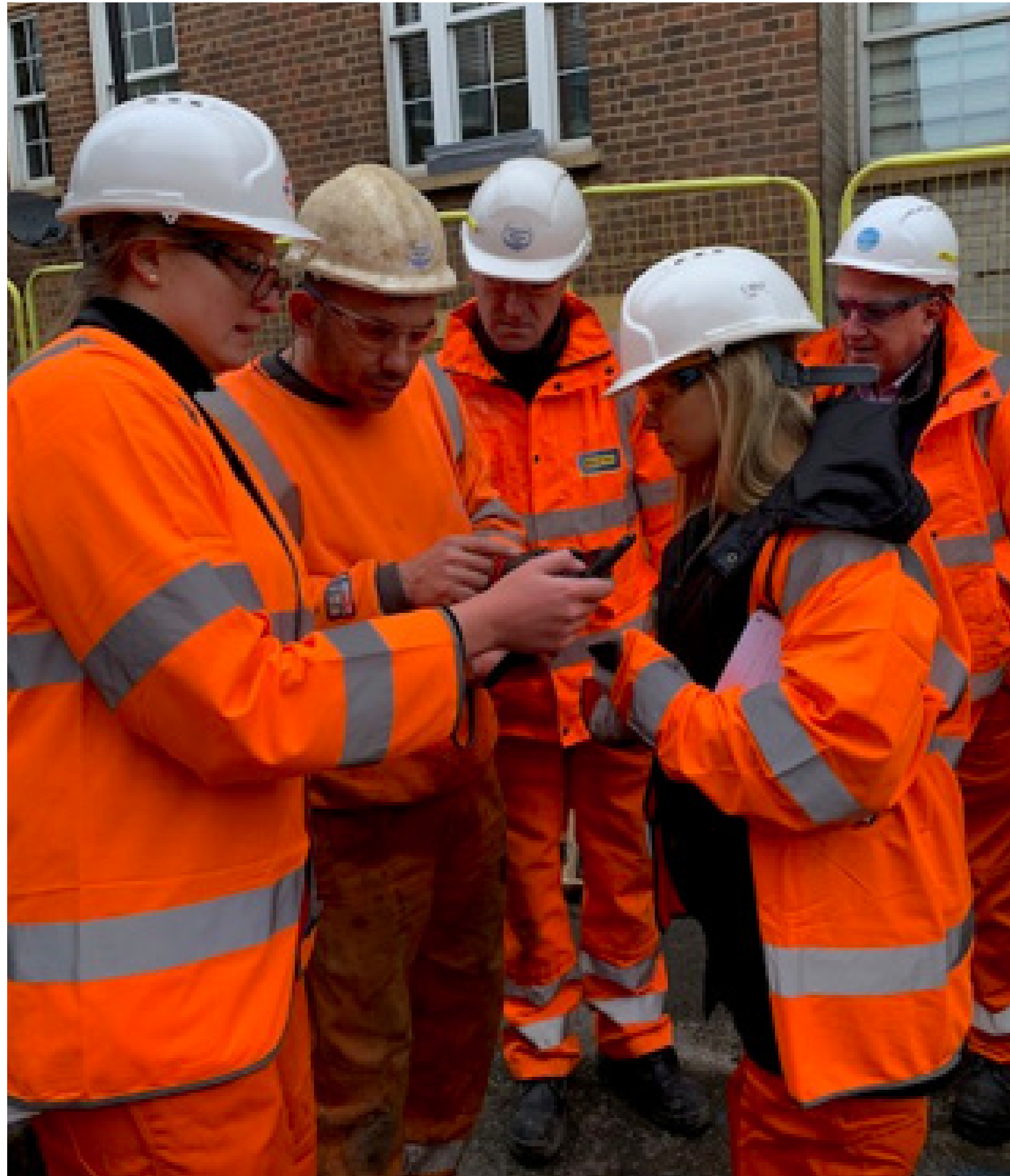
Field testing of the mobile NUAR prototype in London with the support of J Browne Construction on behalf of Thames Water
