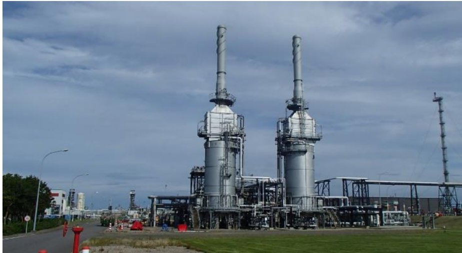
Figure 5-5: NSMP Gas Fired Hot Oil Heaters (Image: PX Group)
