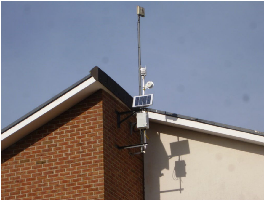
Figure 1: TEST Project weather station mounted at 12 m above ground in Widnes
