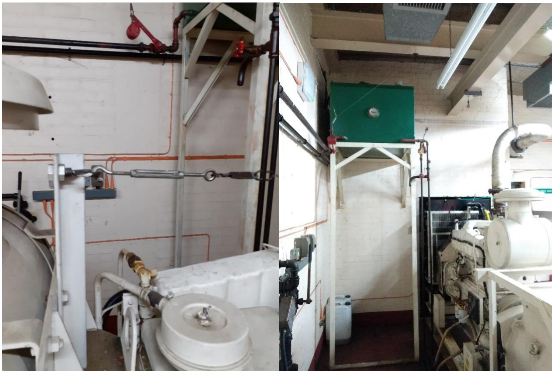
Mechanism which became loose and detached from generator, subsequently becoming jammed in the firewire pulley wheel.
