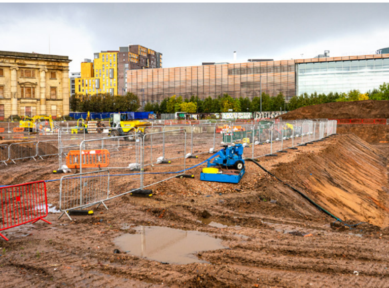
Works underway at the Phase One terminus at Curzon Street in Birmingham.
