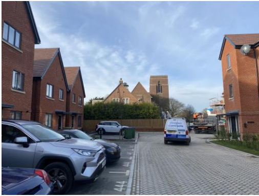
View to the east from Blunden Drive with the Sir John Moore Memorial Hall in the background
