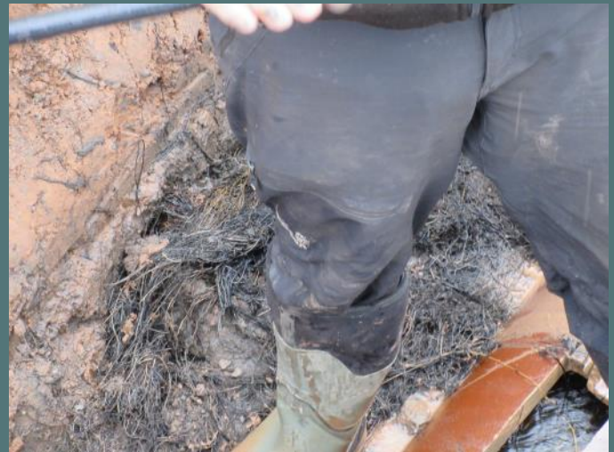
Roots that had been blocking the pipeline and contributing to flooding
