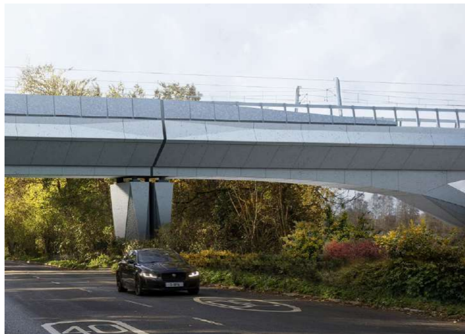
Fig.5.101_ Visualisation (10) - 4m hybrid to 4m opaque barrier transition at Moorhall Road crossing
