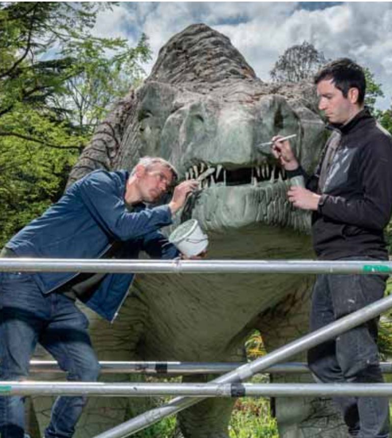
Repair of the Crystal Palace Dinosaurs, Bromley, Greater London. Funded by the Culture Recovery Fund for Heritage. Crafts people created 22 new teeth and a 'prosthetic' jaw and nose for the listed structure.
