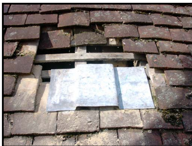
The Batslate shown here is fitted so that a whole tile will fit alongside it. Where this is not possible, tiles will require cutting. The Bat-slate is nailed (x2) to the batten.
