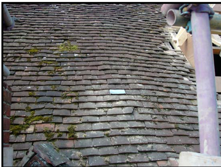
Not the best picture in the World, but this is what the Batslate looks like in the middle of a plain tile roof. From the ground it is almost invisible.
