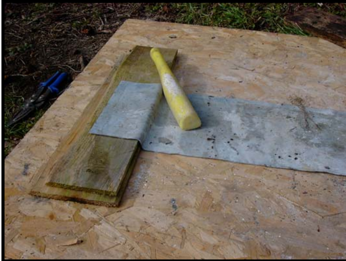
Dressing the lead over suitable sized timber. The depth of the finished Batslate should be 17-20mm.
