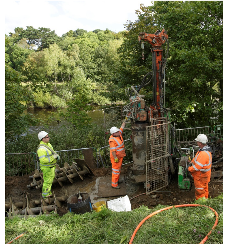
Repairing a river bank after flooding in Corbridge, Northumberland. Northumbria Integrated Drainage Partnership's commitment to building relationships has enabled collaborative action both within and beyond partnership activities.
