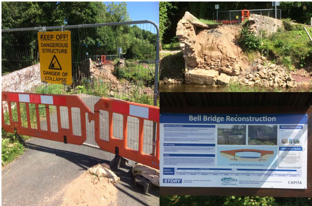
Plate 3: Bell Bridge on the River Caldrew, south of Carlisle, collapsed in late January 2016, as a result of damage sustained during Storm Desmond a month earlier. These images from July 2017 illustrate the closure (stabilisation) of the bridge pending the implementation of the full reconstruction (recovery) project. Note the information board which has been designed to explain the on-going process to the public.
