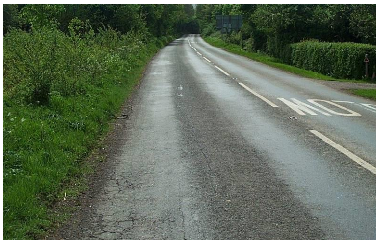
Figure 8 Variation in average texture depth across the road surface
