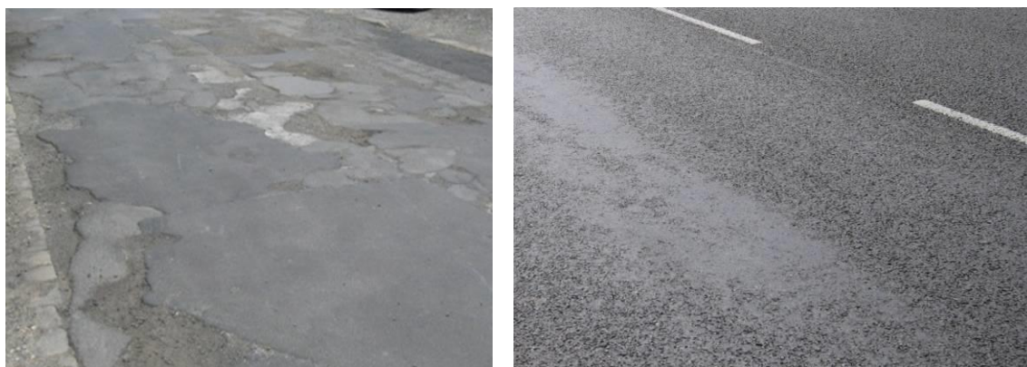
Figure 14: Wearing coarse deterioration (left) and surface deterioration (right)
