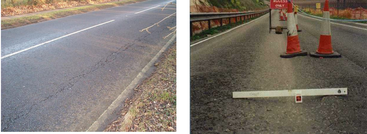
Figure 12: Wheel track cracking (left) and wheel track rutting (right)
