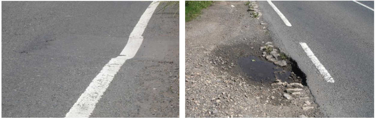
Figure 15: Settlement and subsidence (left) and edge deterioration (right)
