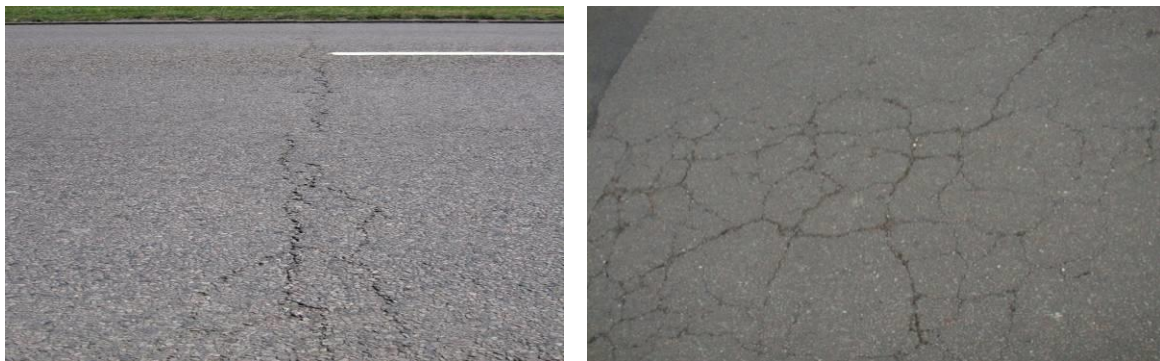
Figure 13: Transverse/reflection cracking (left) and whole carriageway cracking (right)
