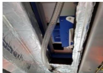
Installed ioniser & sensor to detect levels of ionisation
