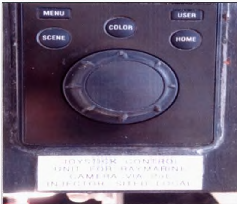
Figure 1.4.25 – Thermal Optical Camera Control Panel.
