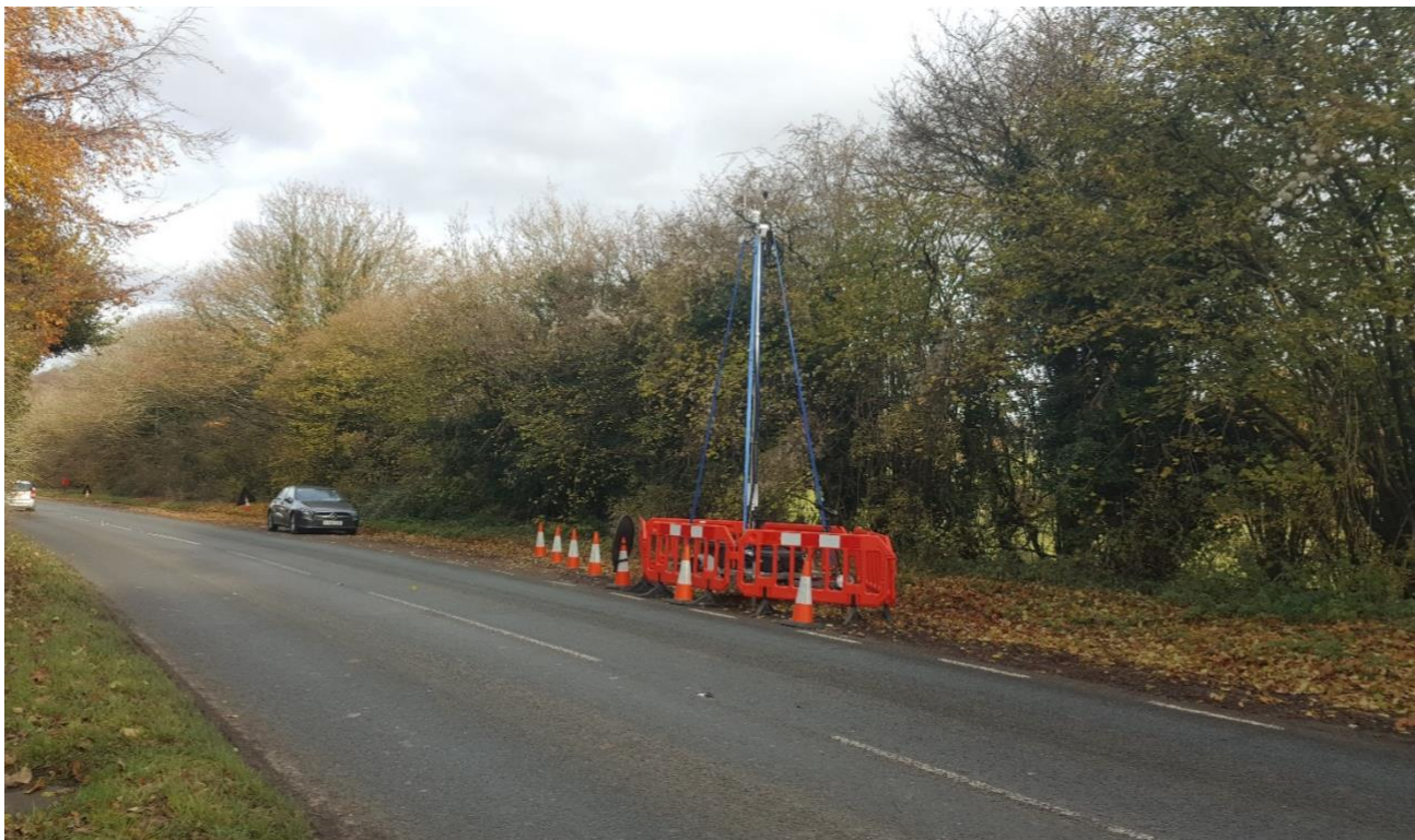
Figure 4.2. Noise camera installed on the A32 north of West Meon
