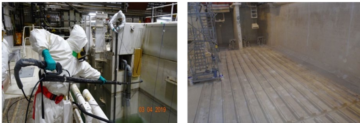
Figure 52: Use of pressure washing from a walkway (left). Fully drained pond (right).
