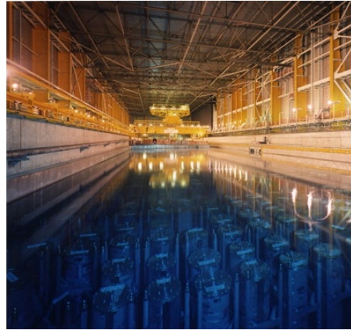
Figure 5: The Fuel Storage Ponds in THORP
