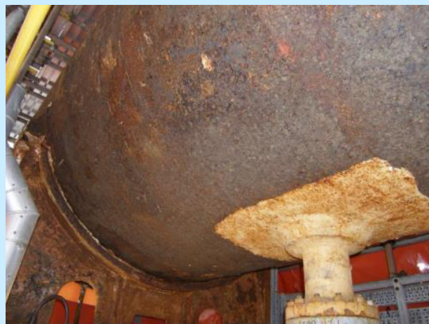
Figure 20 – CO 2 tank 21 as found
