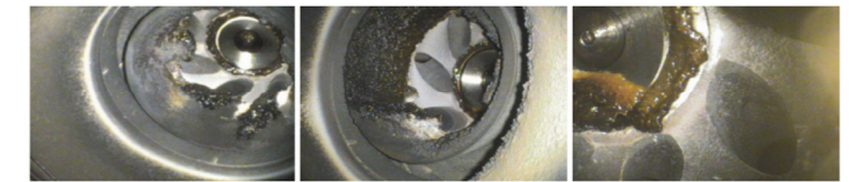
Brown material deposits in No 2 engine combustion chamber swirl cups
