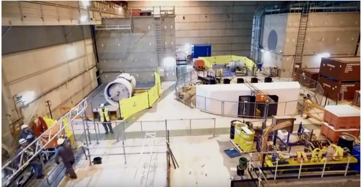
Figure A3: Image taken from promotional video of UAV flight through SGHWR building at Winfrith. [2].
