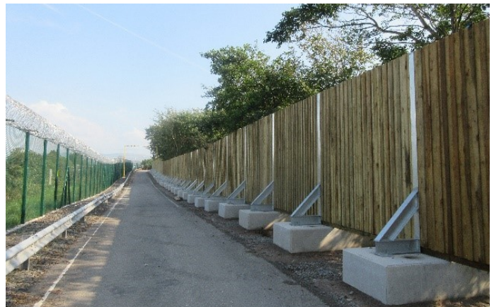
Specially-constructed barriers will mitigate the impact of construction noise on the local community
