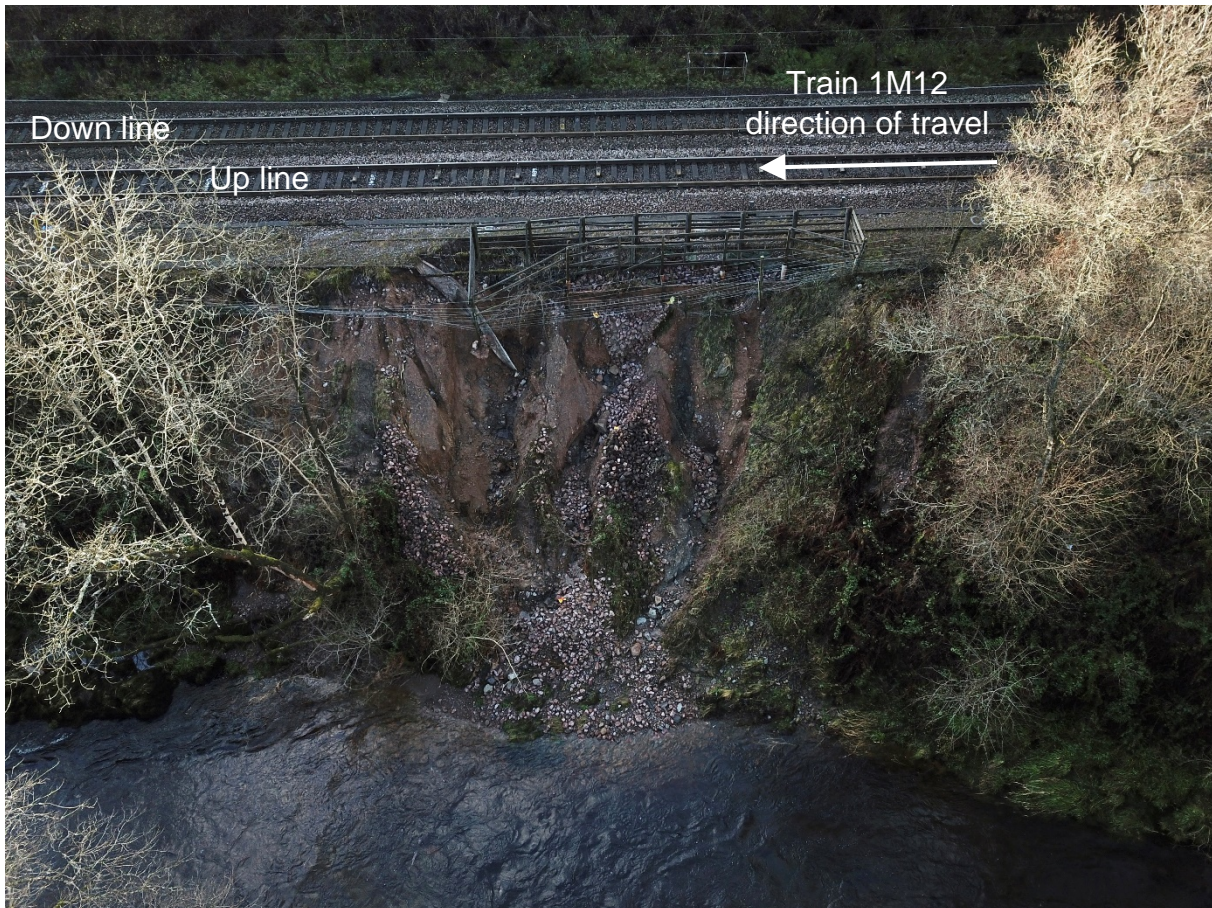
The section of embankment that was washed away by the flood water
