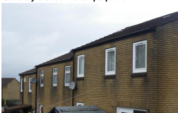
Insufficient overhang of sills and verge
