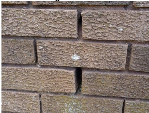
Severely eroded mortar perp end
