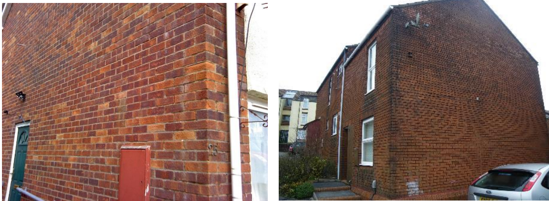
Damaged face of bricks
