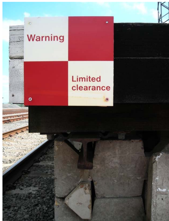
Limited clearance warning sign
