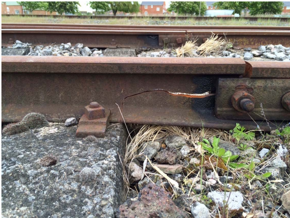
Figure 6.1 Example of a Broken Rail
