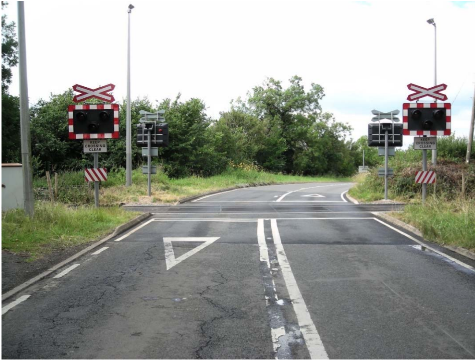
Figure 10.2 Automatic open crossing, locally monitored.
