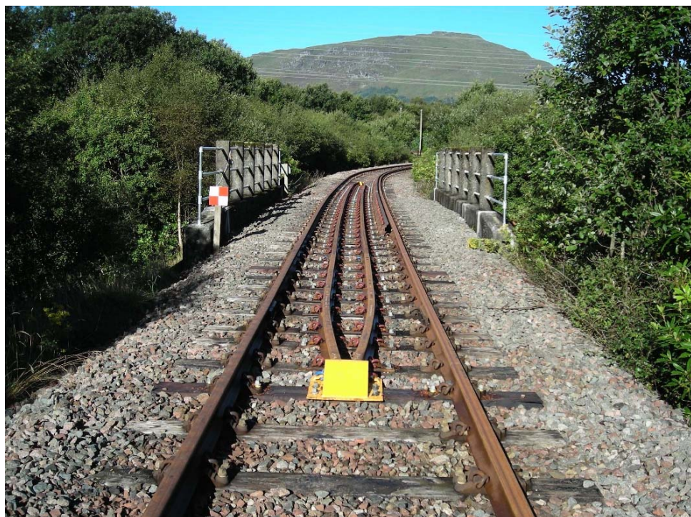
Figure 11.12 Derailment Guard Rails
