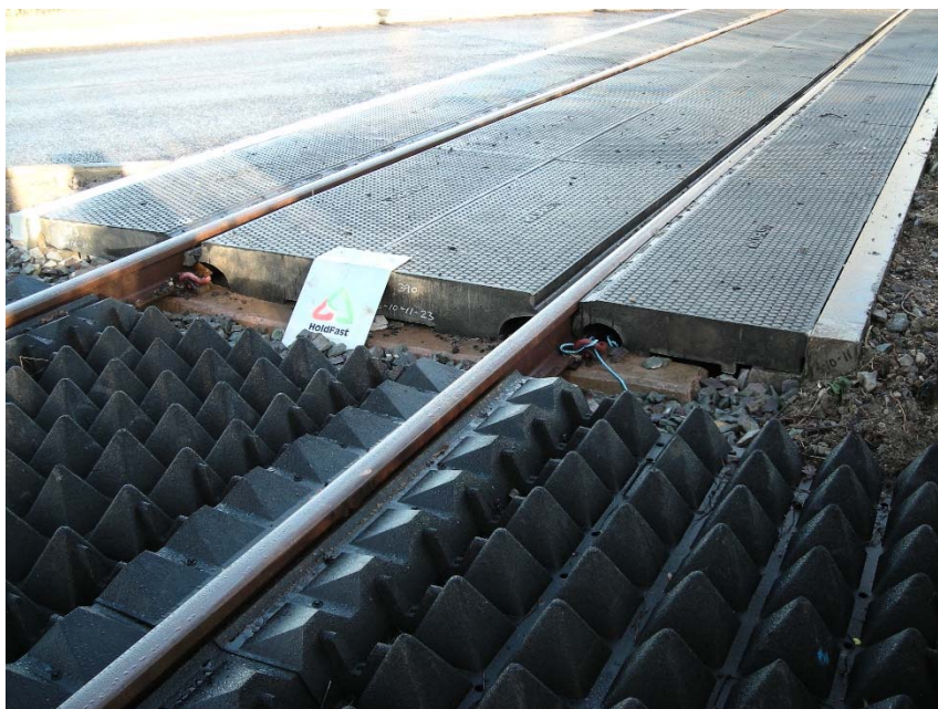
Figure 10.5 Rubber panel type crossing with rubber trespass guard panels
