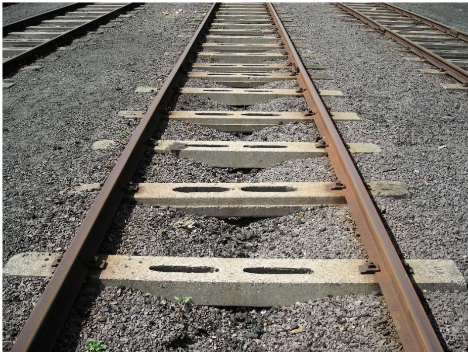
Figure 6.7 Plain line track – obsolete BS75R rail on concrete sleepers
