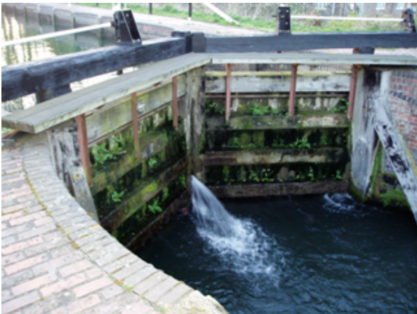
Figure 11.7 Traditional wooden lock gates
