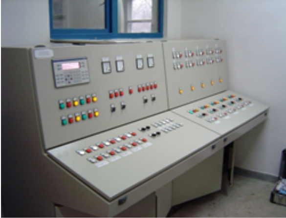
Figure 11.17 Control desk at small pumping station
