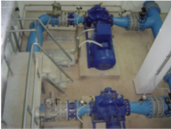
Figure 11.13 Dry well pumping installation
