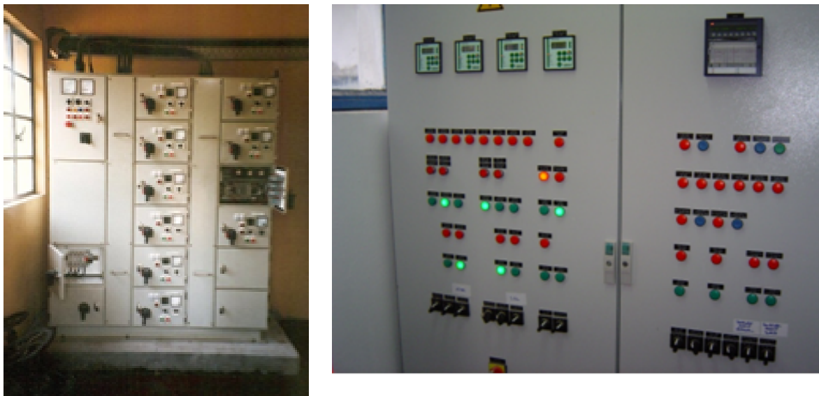
Figure 11.16 Typical examples of motor control panels
