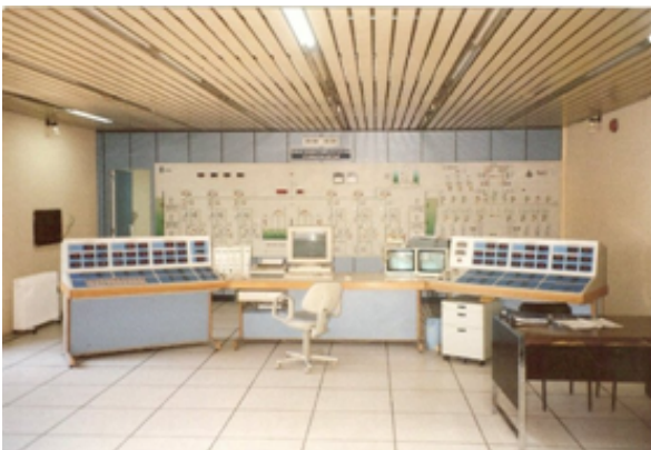
Figure 11.18 Central control room for larger scheme
