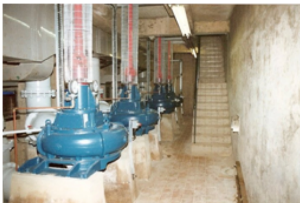
Figure 11.12 Dry well pumping installation
