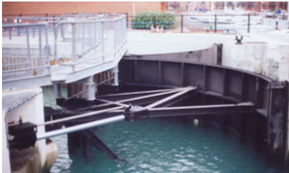
Figure 11.9 A pair of vertical axis sector gates used for a lock entrance
