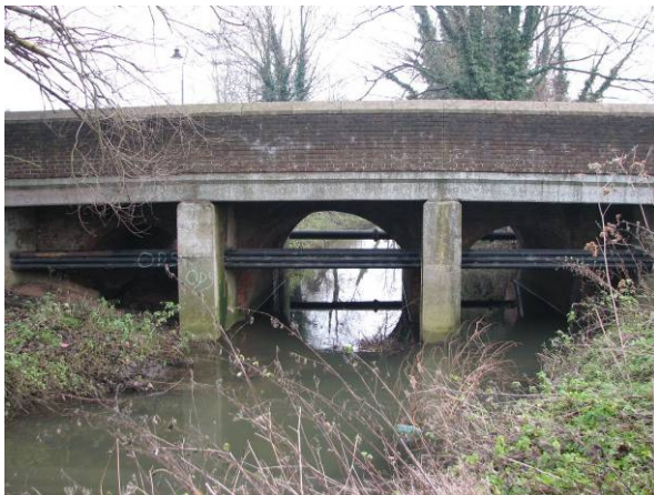
Figure 8.22 Service crossing obstructions
