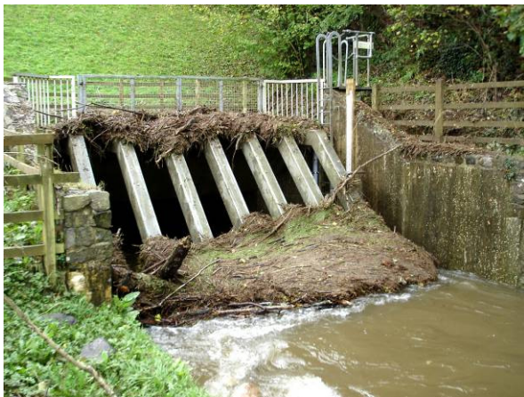
Figure 8.25 Even coarse screens can become blocked
