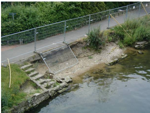
Figure 8.8 Lack of timely repairs
