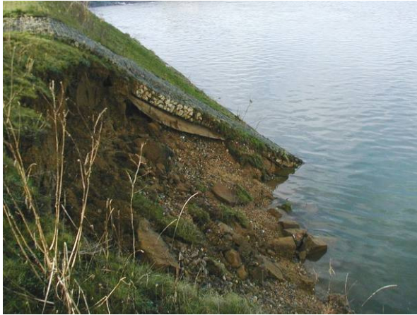
Figure 8.12 Bank protection not long enough
