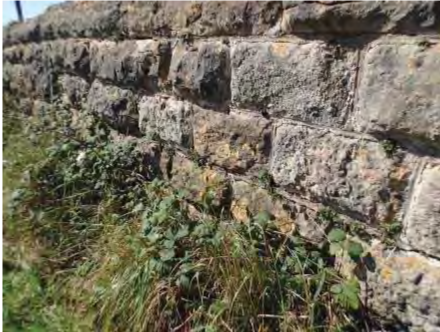
Photograph 39: example of lifting and cracking mortar noted along the C/e parapet
