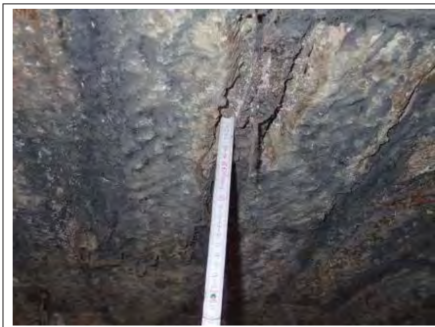
Photograph no 12: spalling at joint lines noted up to approx 50mm
