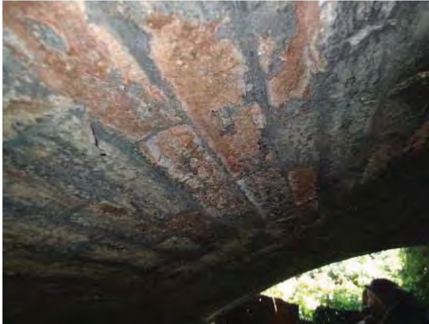
Photograph 13: example of long-standing spalling action within the soffit
