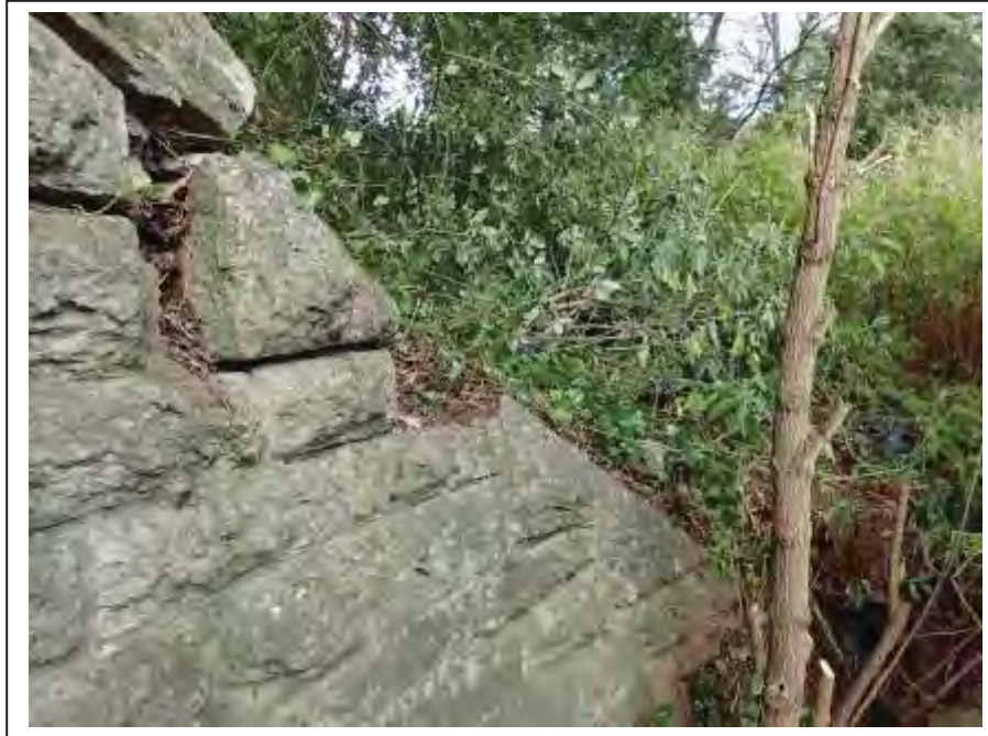
Photograph no 29: long-standing loss of copings along the U/S, L/e wingwall
