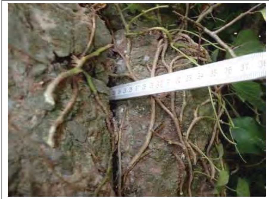
Photograph no 61: joint loss at the fracture line noted up to 240mm
