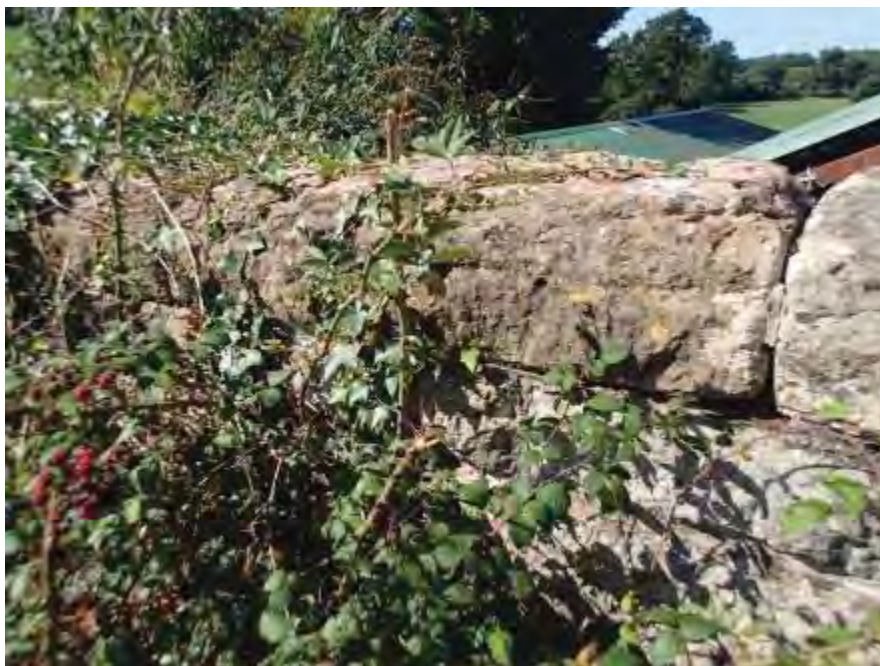
Photograph 42: a coping on the U/S of the parapet was found to lift on insertion of a lever
