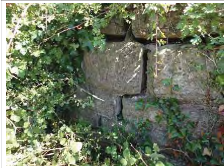
Photograph no 13: long-standing fracture and displacement noted towards the U/S quoin of the L/e parapet
