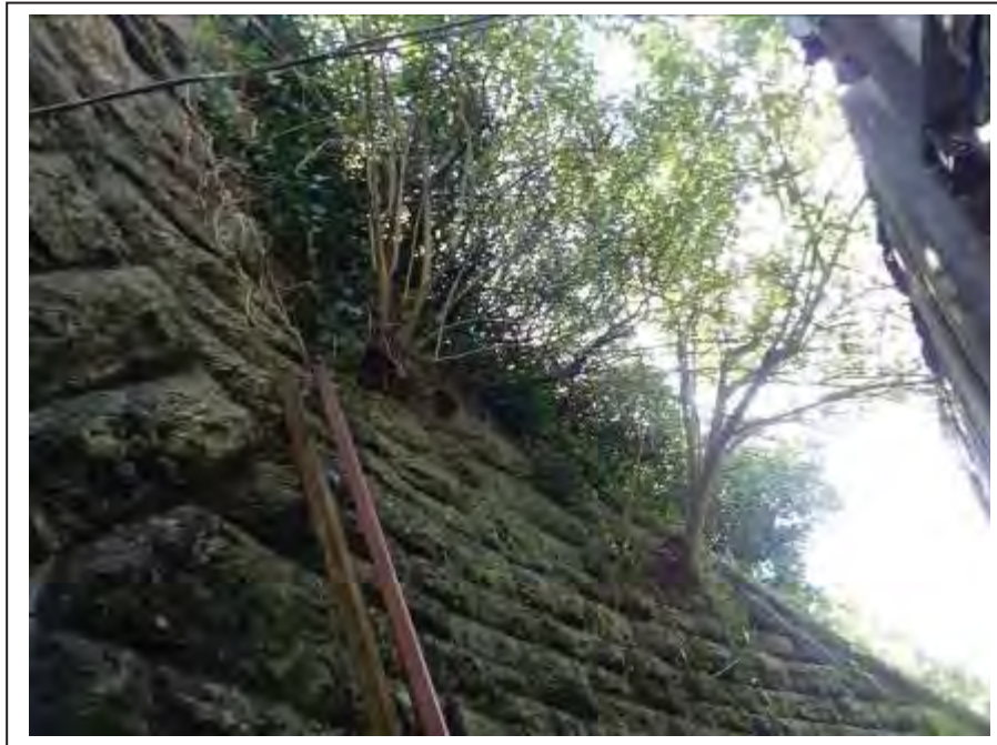
Photograph no 15: example of long-standing root ingress along the rake line of the D/S, C/e wingwall
