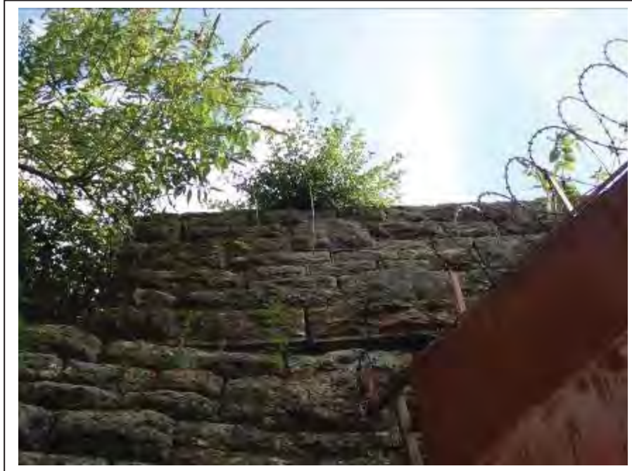
Photograph no 21: external face of the C/e parapet stonework within 2.2m of the U/S quoin showed movement under hammer at time of the previous detailed examination
