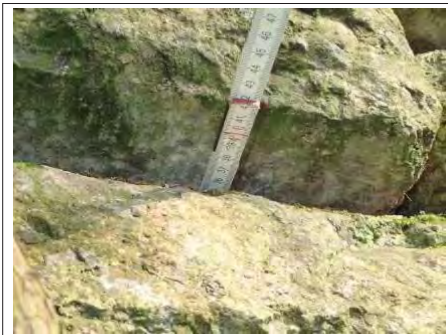
Photograph no 40: joint loss at the area of root ingress noted up to 420mm
