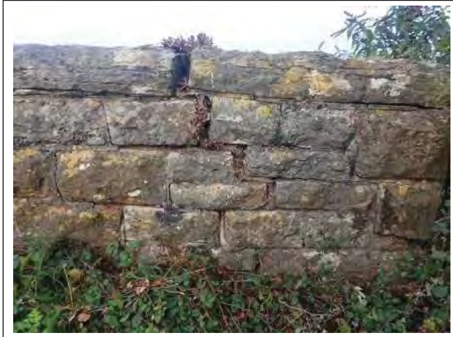
Photograph no 65: long-standing fracture and displacement noted at the U/S quoin of the C/e parapet Fractures/ displacement are caused by root ingress.
