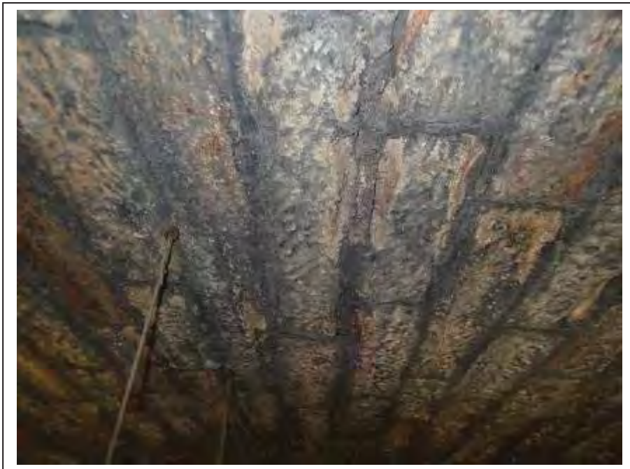
Photograph no 8: example of spalling along the joint lines within the soffit
