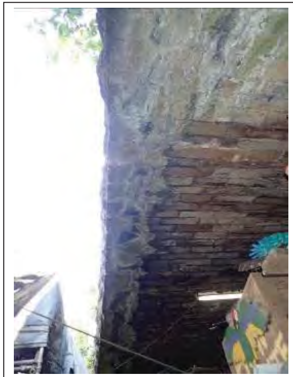
Photograph no 10: calcite deposits located to the rear of the C/e voussoirs
