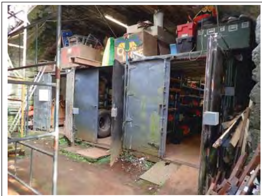
Photograph no 28: storage containers restrict access to the abutments.
