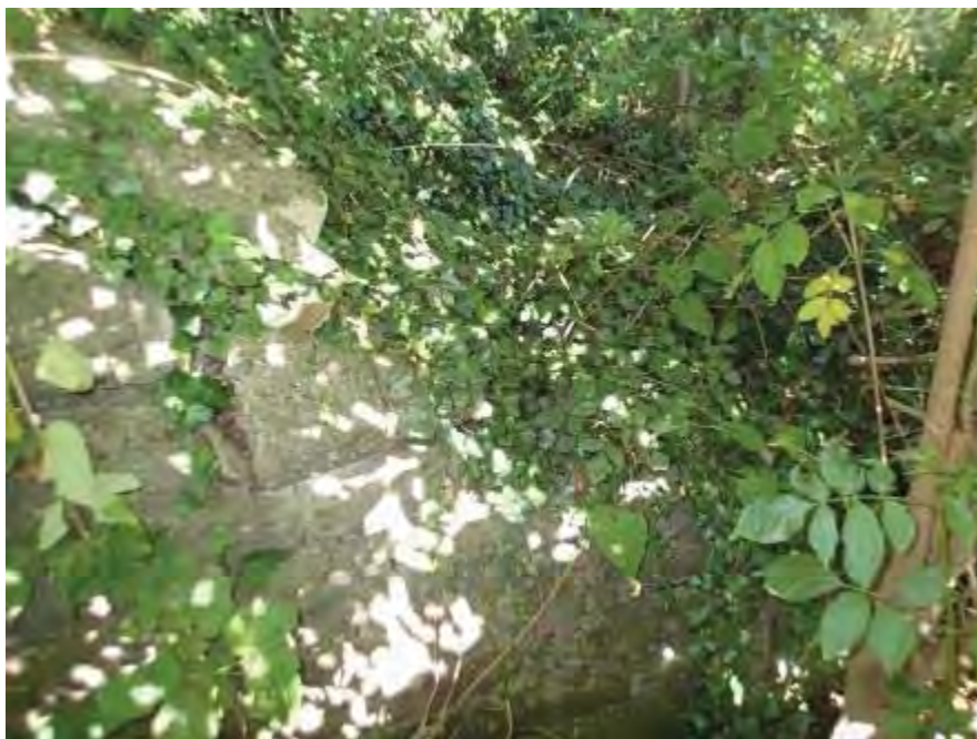
Photograph 14: long-standing coping loss is noted along the U/S, L/e wingwall
