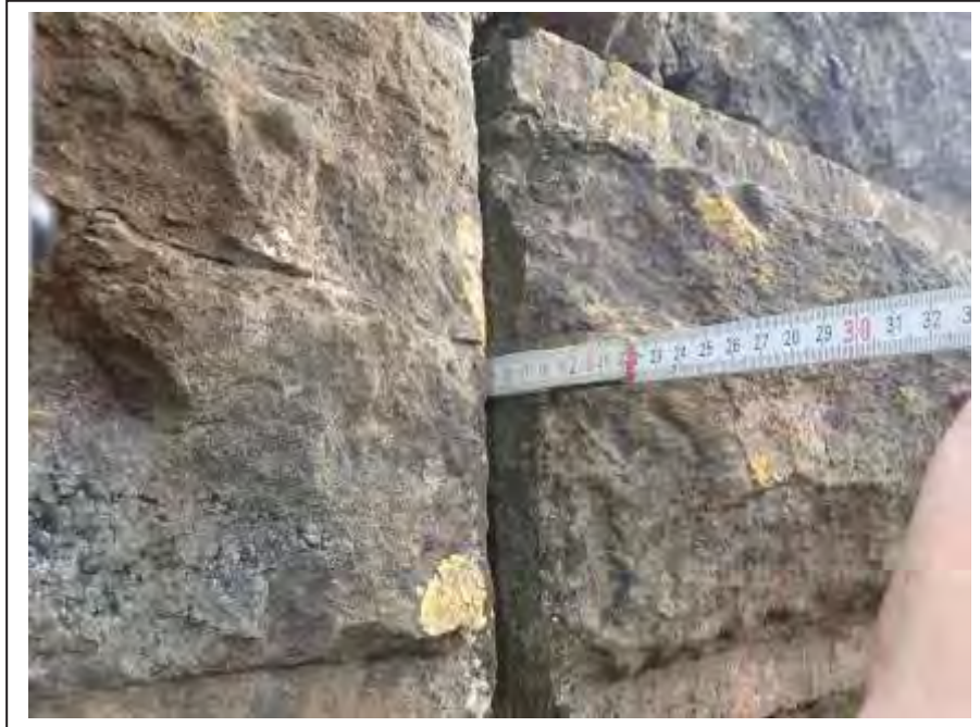
Photograph no 81: individual perp joints within the C/e stringcourse show loss up to 175mm
