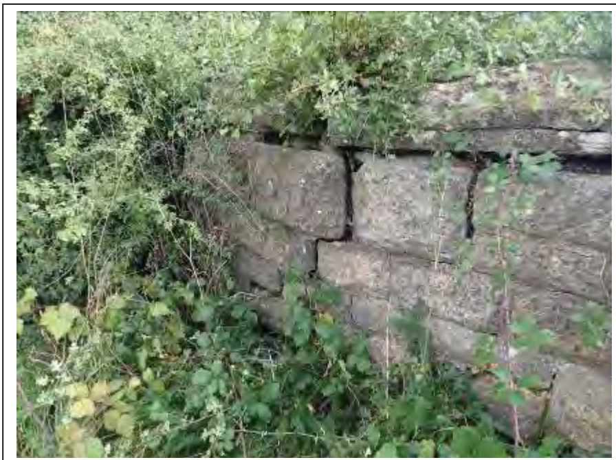
Photograph no 18: long-standing displacement of stonework at the U/S quoin of the L/e parapet
