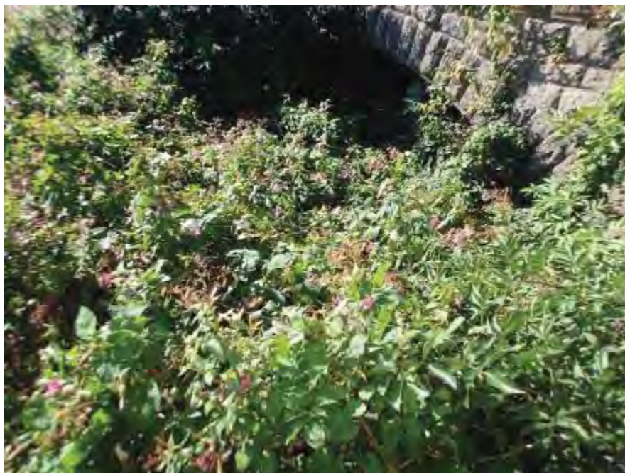
Photograph 44: widespread Himalayan Balsam is noted on the L/e of the structure
