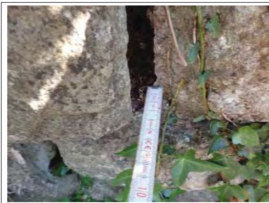
Photograph no 14: forward displacement noted up to 45mm at fracture line
