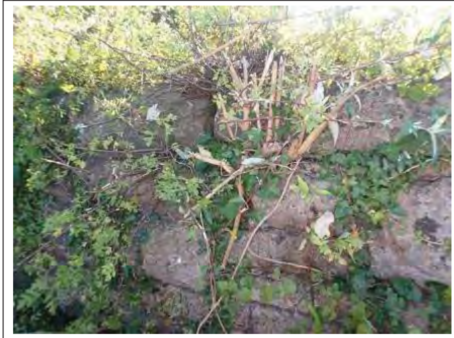
Photograph no 11: lifting copings noted along the L/e parapet due to root ingress approx 2.7m from the U/S quoin
