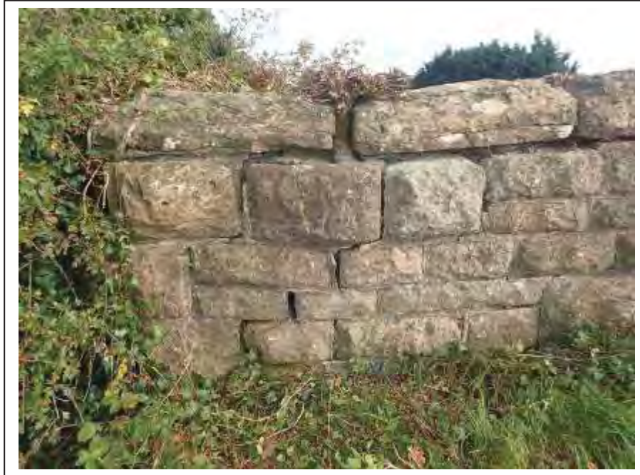
Photograph no 47: long-standing fracturing and displacement at the U/S quoin of the L/e parapet
