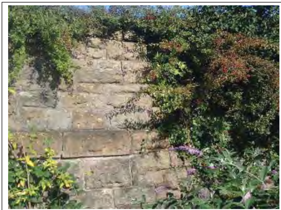
Photograph no 10: fracturing noted towards the U/S quoin of the L/e parapet within the external face
