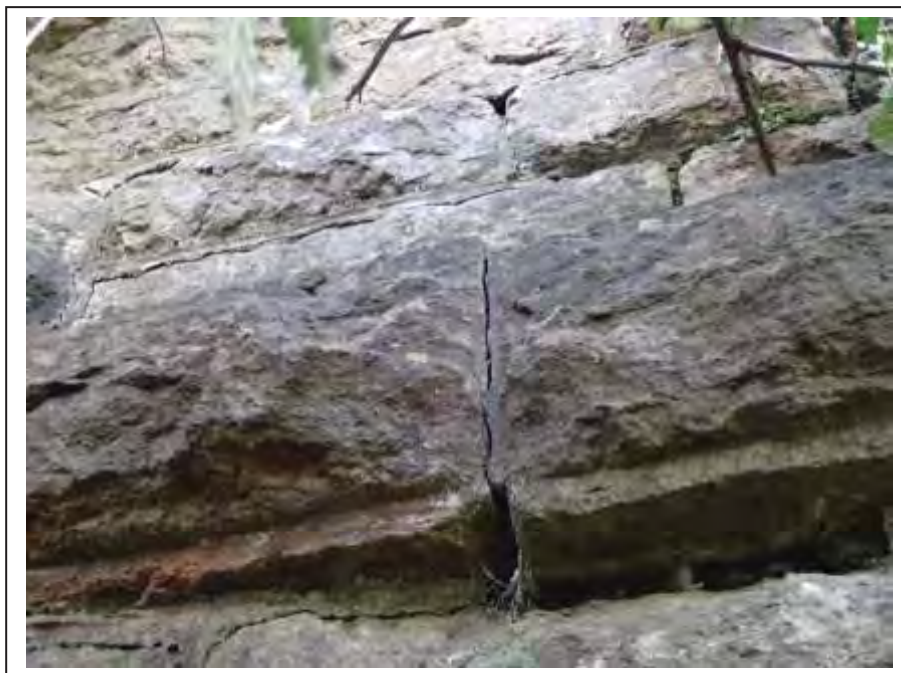
Photograph no 64: odd joints within the L/e stringcourse fractured up to 3mm
