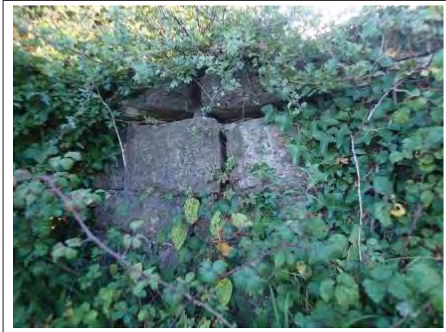
Photograph no 3: long-standing fractured and displaced stonework to internal face of the L/e parapet located towards the U/S quoin
