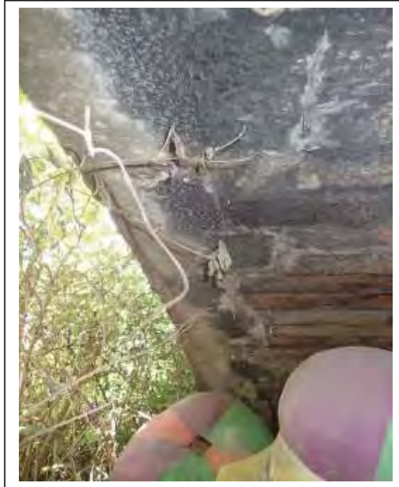
Photograph no 9: calcite deposits noted at the rear of the L/e voussoirs may cover underlying fracture.
