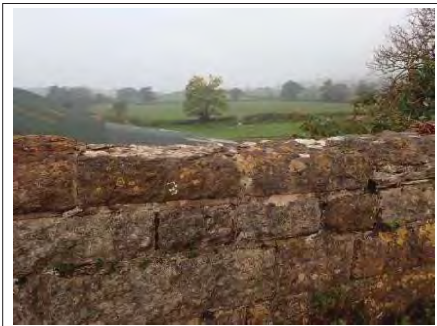
Photograph no 74: example of spalled copings noted along the C/e parapet
