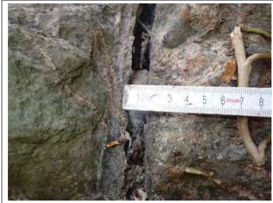
Photograph no 59: step fracture is typically open to 16mm
