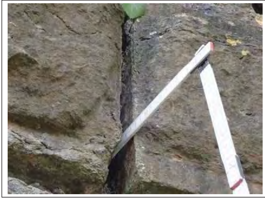
Photograph no 63: odd joints within the L/e stringcourse show loss up to 80mm
