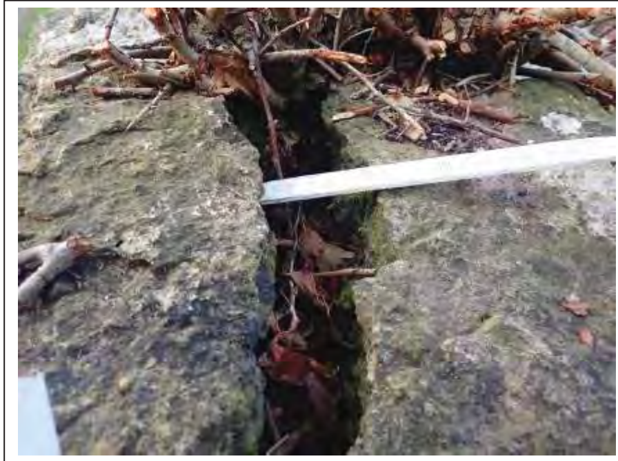
Photograph no 69: fracture within the coping noted to 65mm
