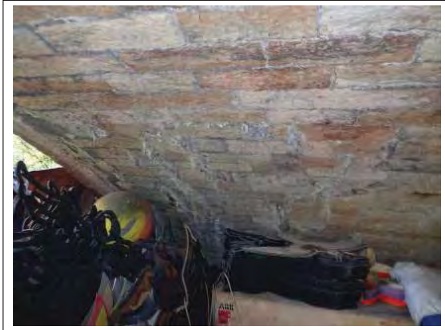
Photograph no 23: example of calcite/ efflorescence staining within the soffit
