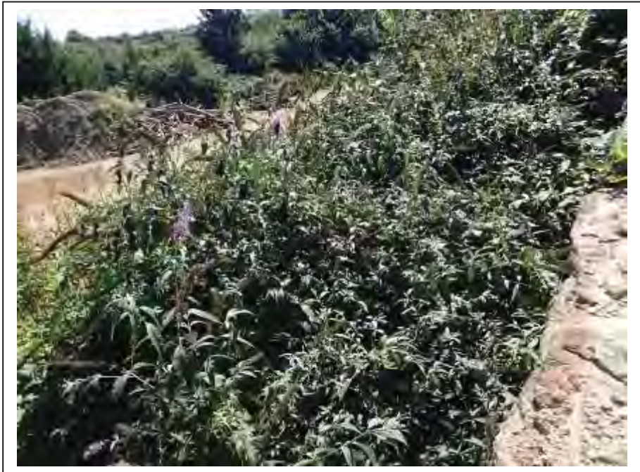
Photograph no 7: dense vegetation restricts access to the L/e elevation. View looking down from the L/e parapet
