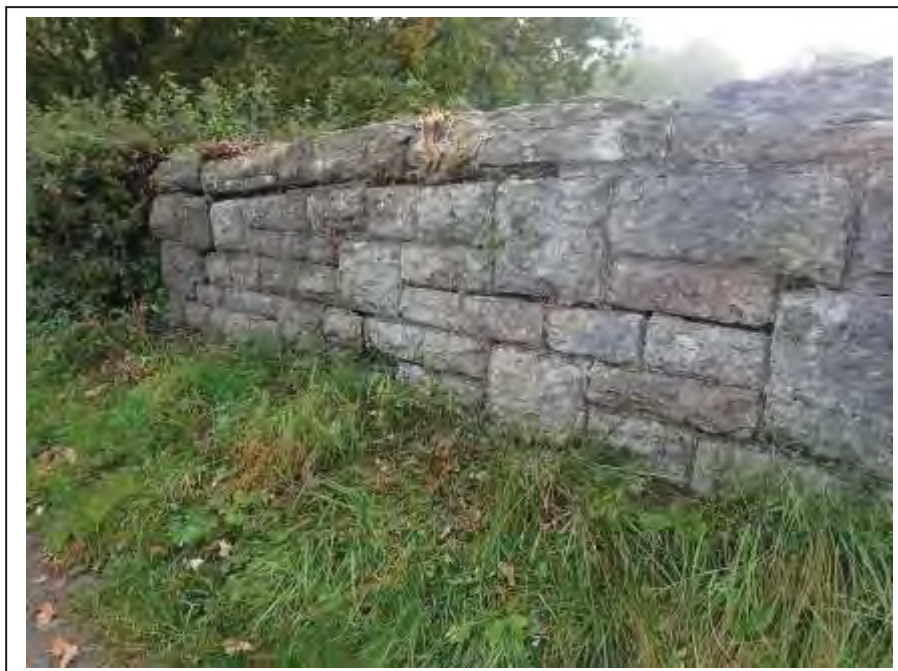
Photograph no 50: widespread joint loss within the L/e parapet noted from the U/S quoin through to 3.8m
