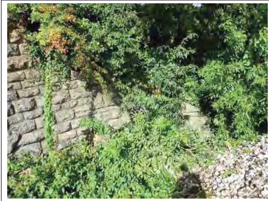
Photograph no 5: general view of the U/S, L/e wingwall
