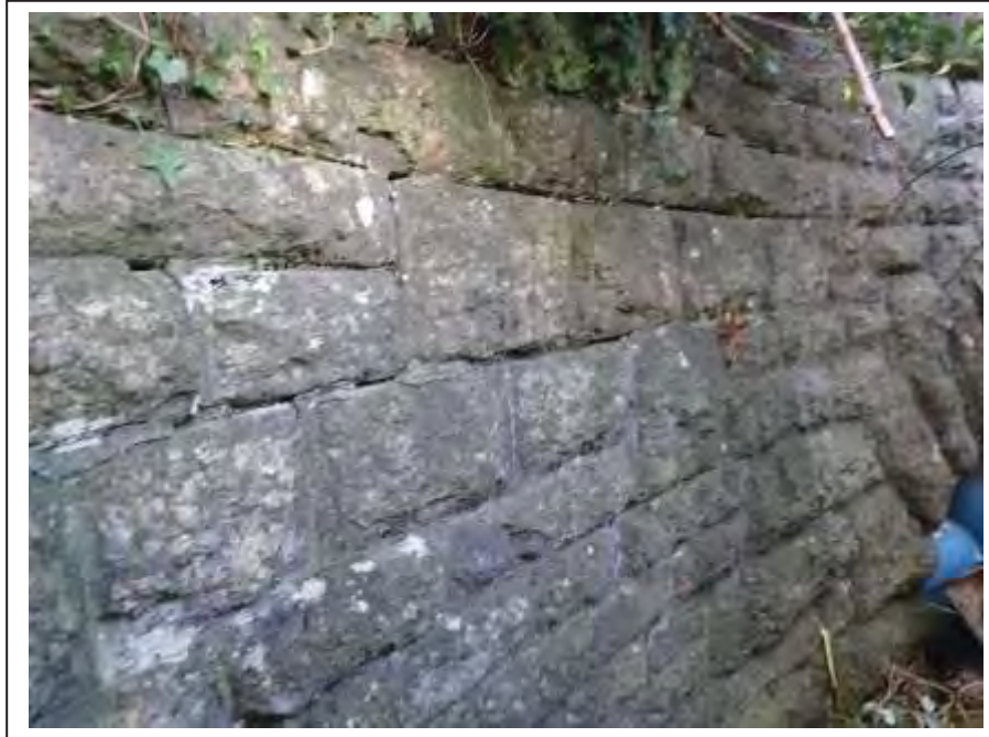
Photograph no 33: example of joint loss within the D/S, L/e wingwall
