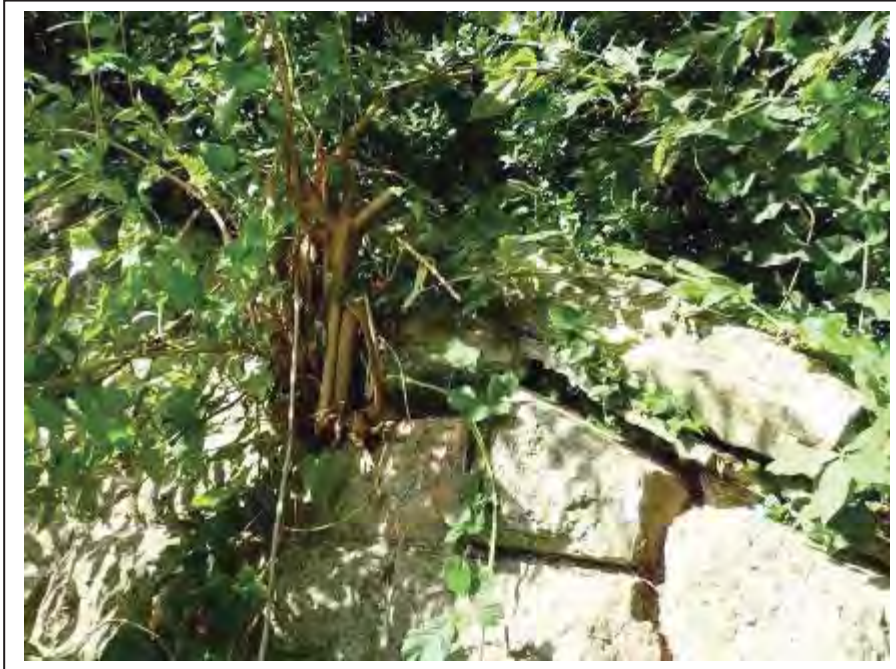
Photograph no 13: root ingress along the rake line of the U/S, L/e wingwall results in lifting copings
