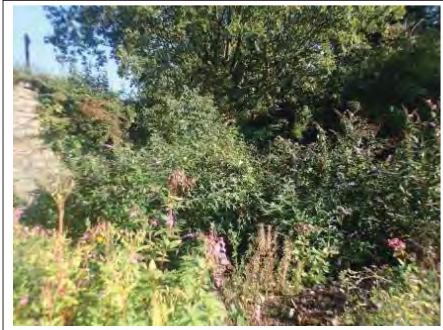
Photograph no 17: U/S, L/e wingwall covered by vegetation
