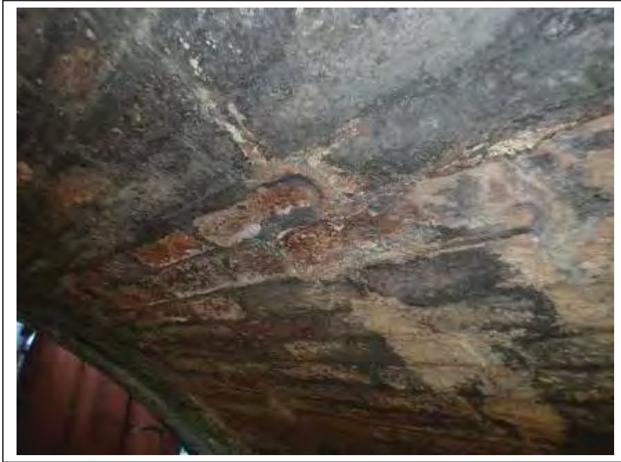
Photograph no 7: example of odd open joints within the soffit
