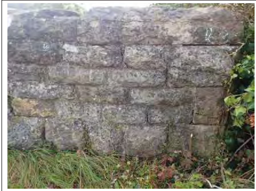
Photograph no 49: series of fractures noted at the D/S quoin of the L/e parapet
