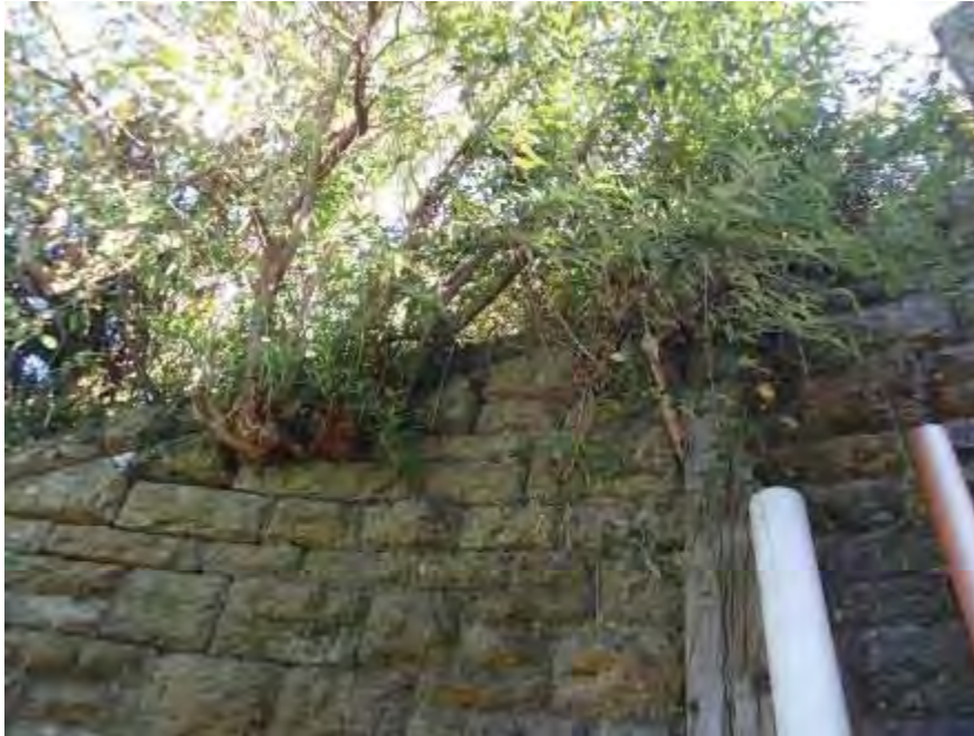
Photograph 17: example of root ingress located along the rake line of the U/S, C/e wingwall
