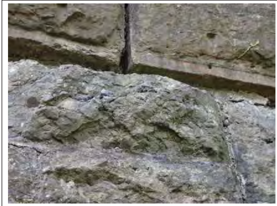
Photograph no 25: evidence of erosion within the stonework to the L/e spandrel
