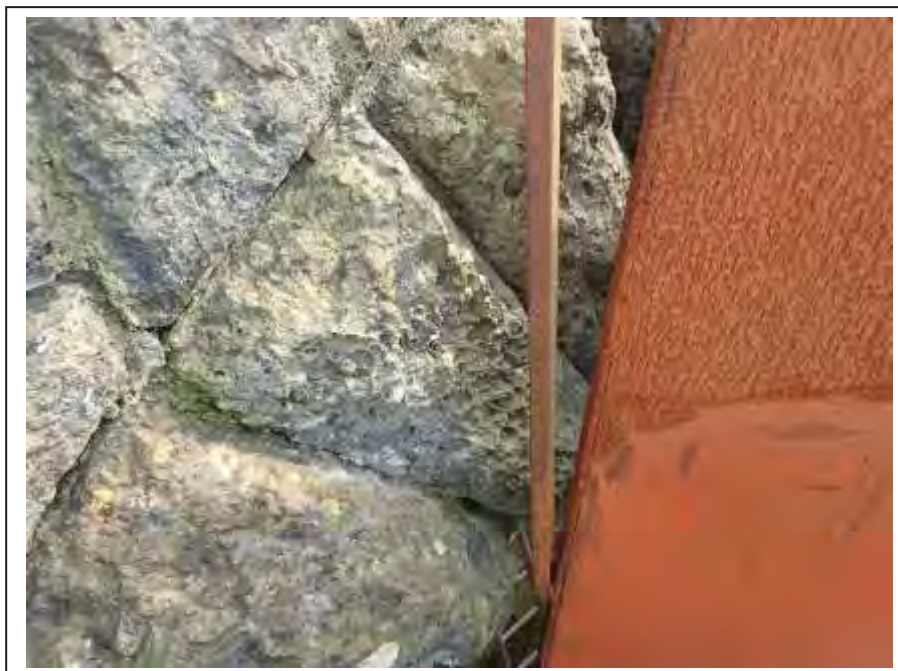
Photograph no 20: example of surface erosion within the C/e voussoirs
