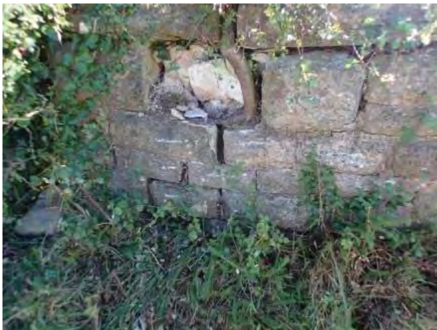
Photograph 22: long-standing displaced fracture located at the U/S quoin of the L/e parapet Stones marked with blue chalk are found loose
