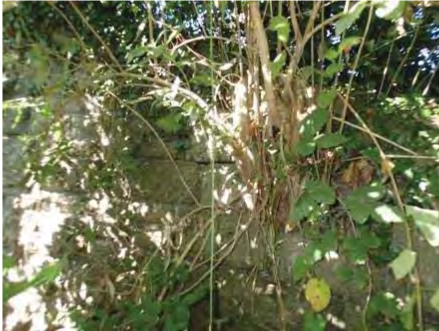
Photograph 15: root ingress along the rake line of the U/S, L/e wingwall results in lifting copings
