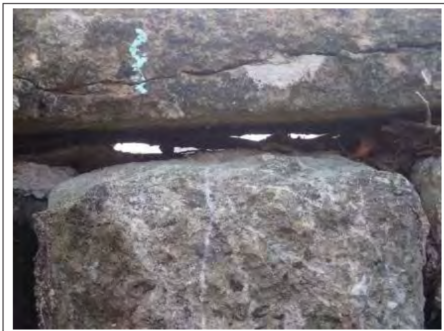
Photograph no 56: daylight visible through the copings along the L/e parapet
