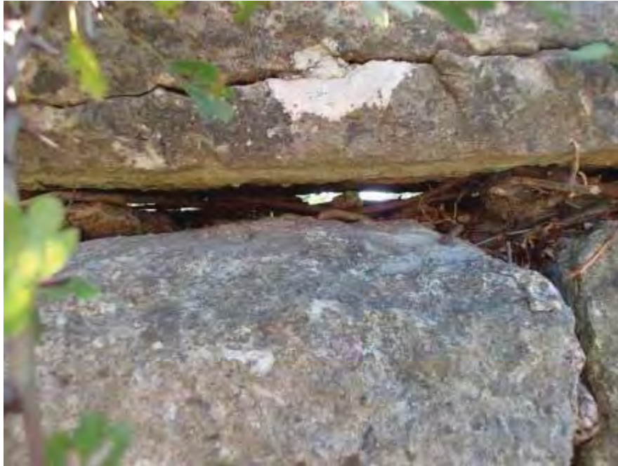
Photograph 29: daylight is visible through the coping bed
