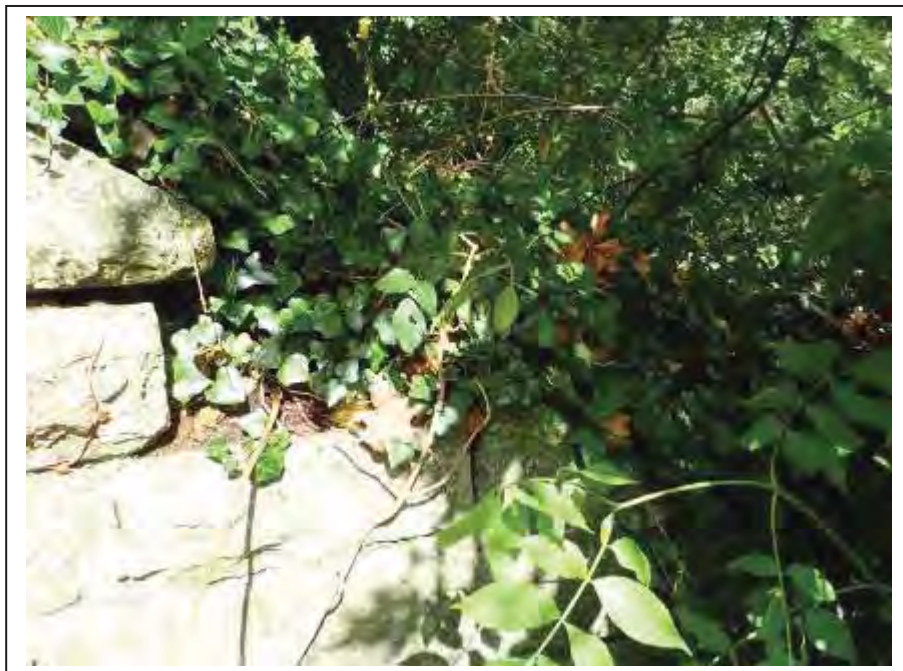
Photograph no 12: long-standing coping loss noted along the U/S, L/e wingwall
