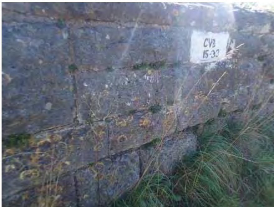
Photograph 30: example of lifting and cracking mortar noted along the L/e parapet
