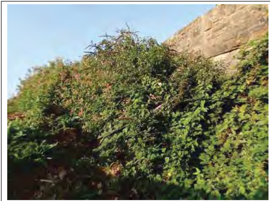
Photograph no 12: vegetation growth located in front of the L/e elevation
