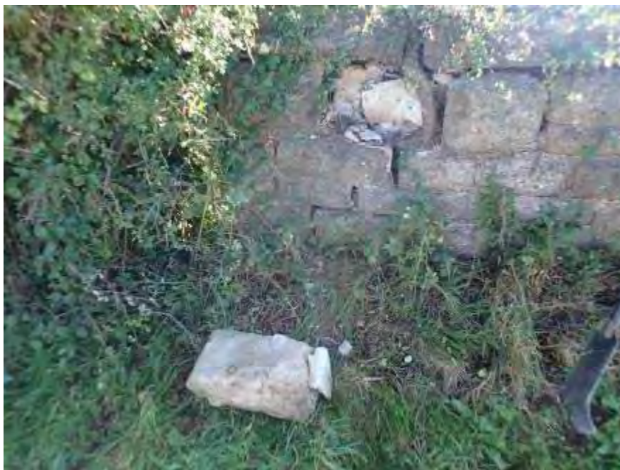
Photograph 20: failure of stone at line of displaced fracture at the U/S quoin of the L/e parapet occurred during the examination
