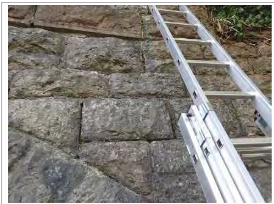
Photograph no 24: example of joint loss within the L/e spandrel noted up to 50mm U/S of the spandrel shown
