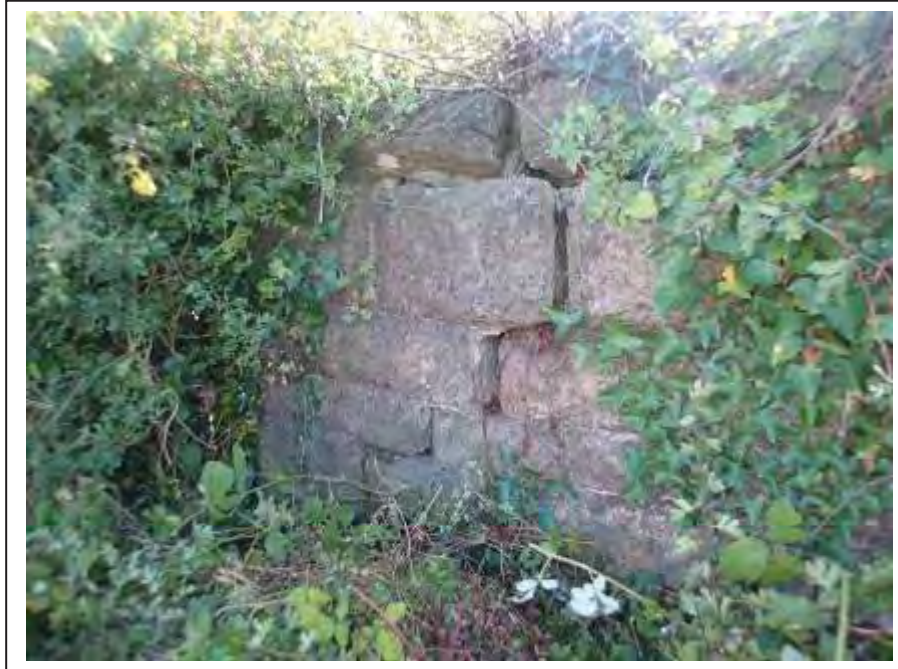
Photograph no 9: long-standing fractured and displaced stonework to internal face of the L/e parapet located towards the U/S quoin
