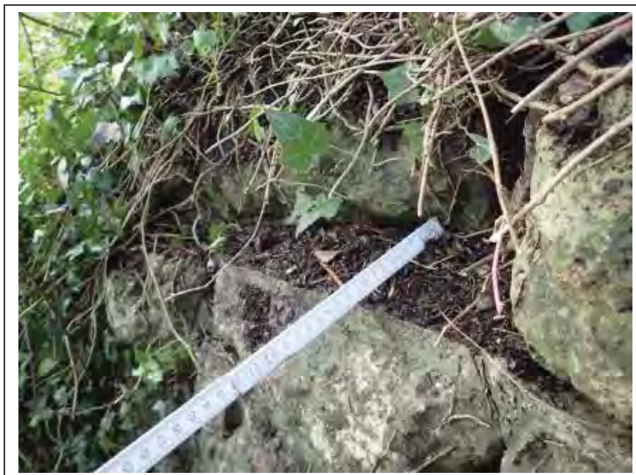
Photograph no 34: displacement of copings at the toe end of the D/S, L/e wingwall noted up to 110mm
