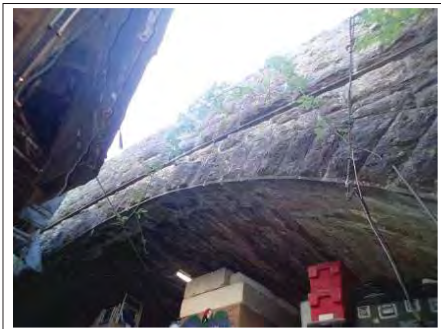
Photograph no 2: Country elevation: view at the rear of the installed buildings Voussoirs appear in good order.
