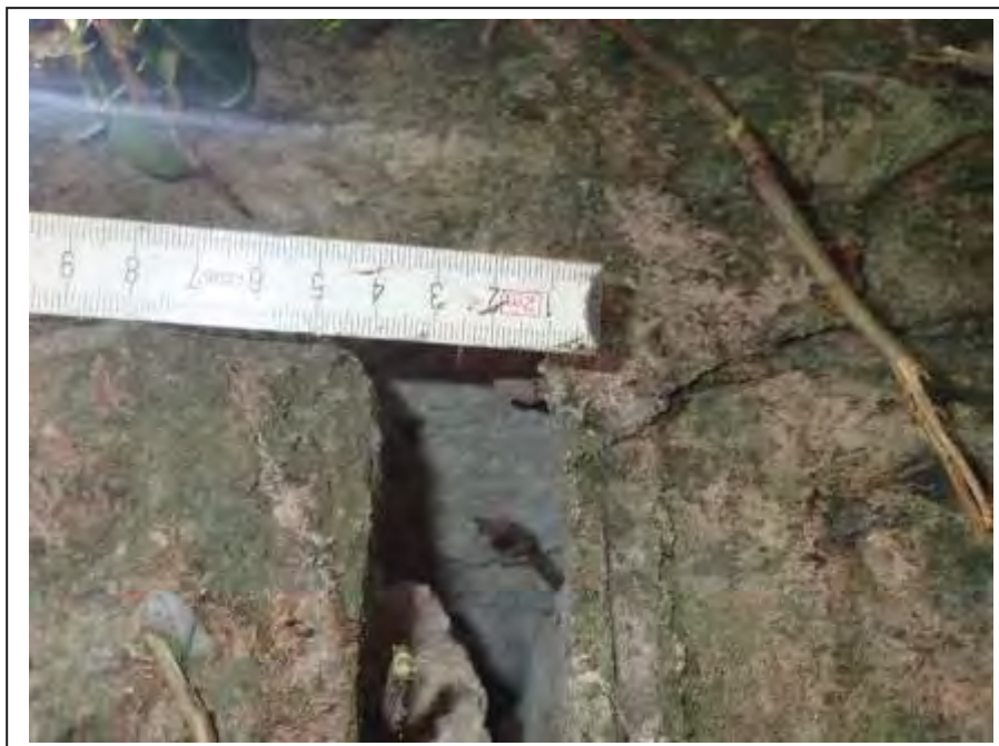
Photograph no 60: step fracture opens to a max of 40mm
