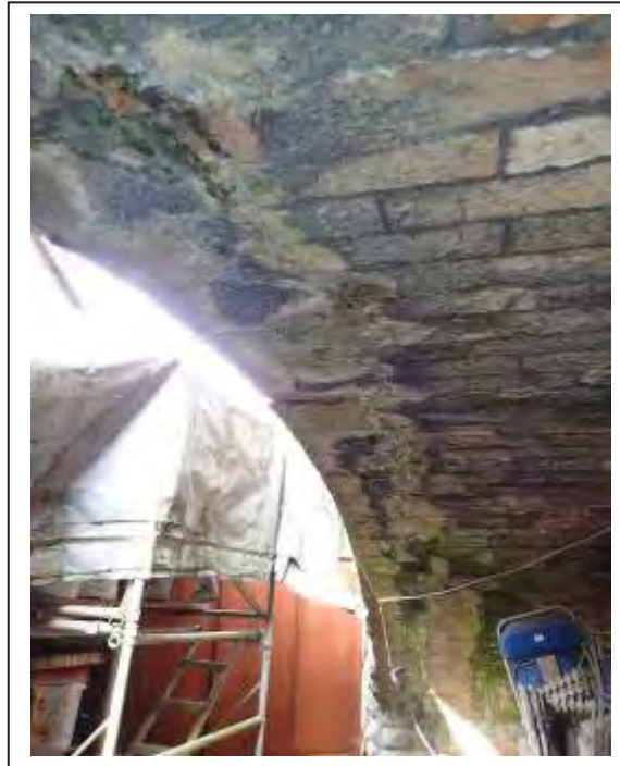
Photograph no 21: calcite deposits to rear of the C/e voussoirs may cover an underlying fracture.
