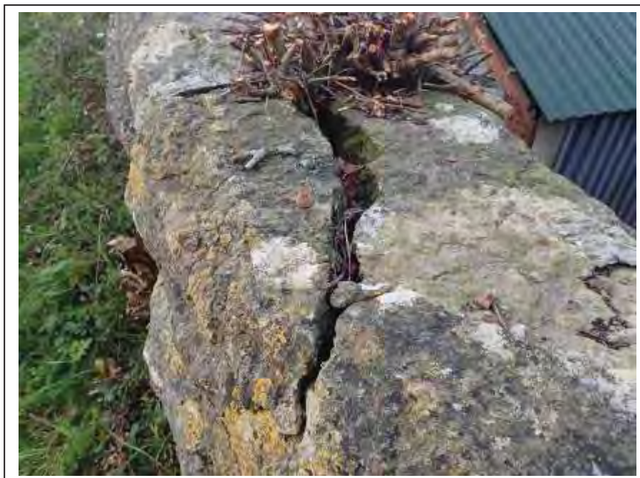
Photograph no 68: fracture within the coping at the U/S quoin of the C/e parapet
