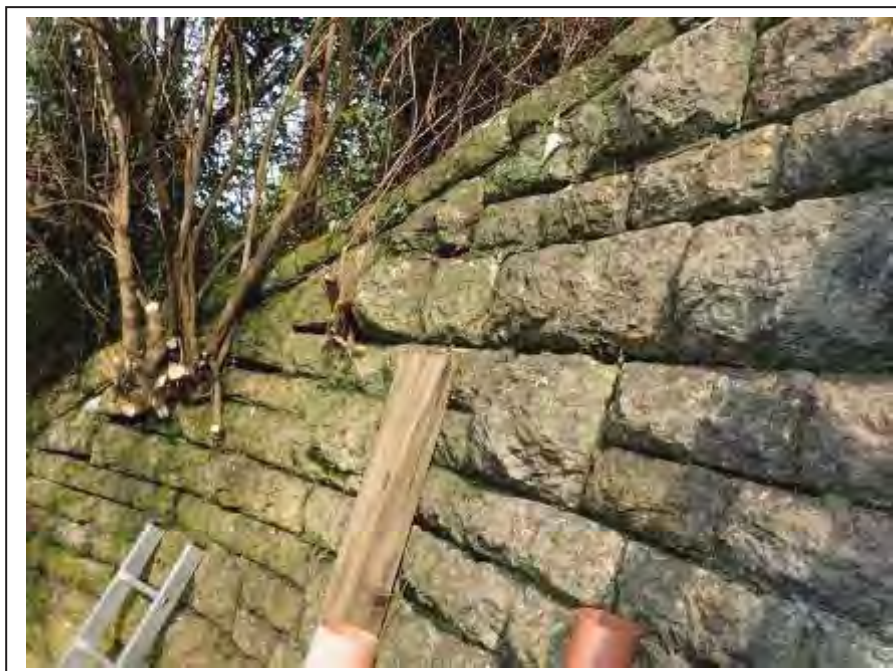
Photograph no 36: example of joint loss within 1m of the copings noted along the U/S, C/e wingwall
