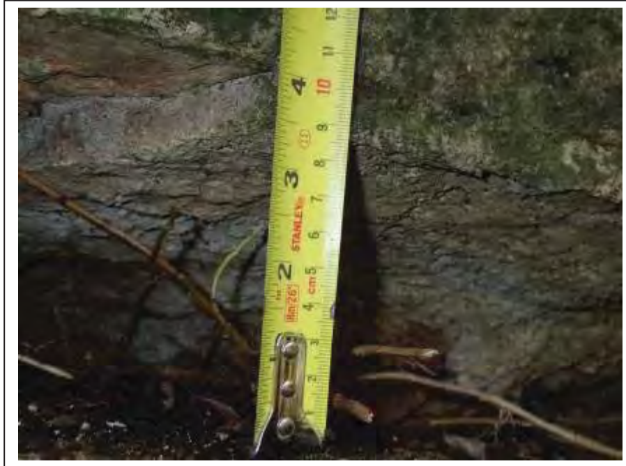
Photograph no 31: displacement noted up to 88mm
