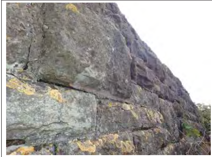
Photograph no 79: individual stones are found pushing within the loose stonework.
