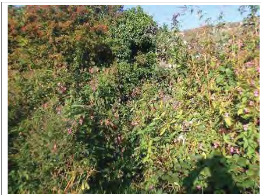
Photograph no 18: D/S, L/e wingwall covered by vegetation
