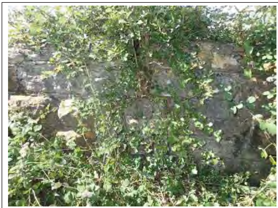
Photograph no 18: long-standing fracture noted towards the U/S quoin of the C/e parapet
