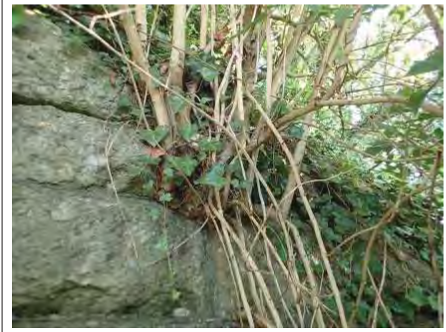
Photograph no 11: sapling growth noted within the U/S, L/e wingwall
