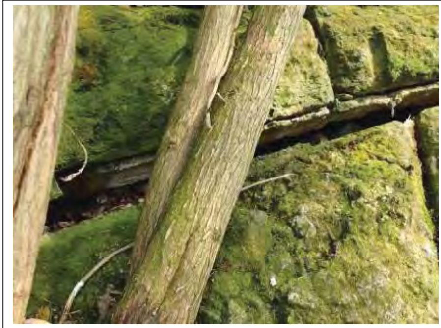
Photograph no 41: lifting of copings at the root ingress noted up to 50mm
