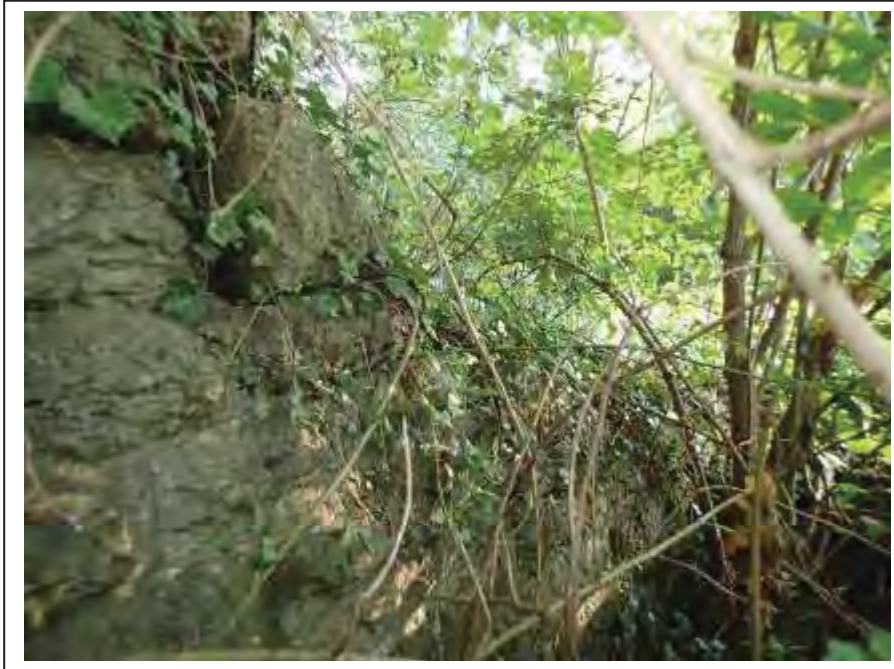
Photograph no 9: long-standing loss of copings to the U/S, L/e wingwall
