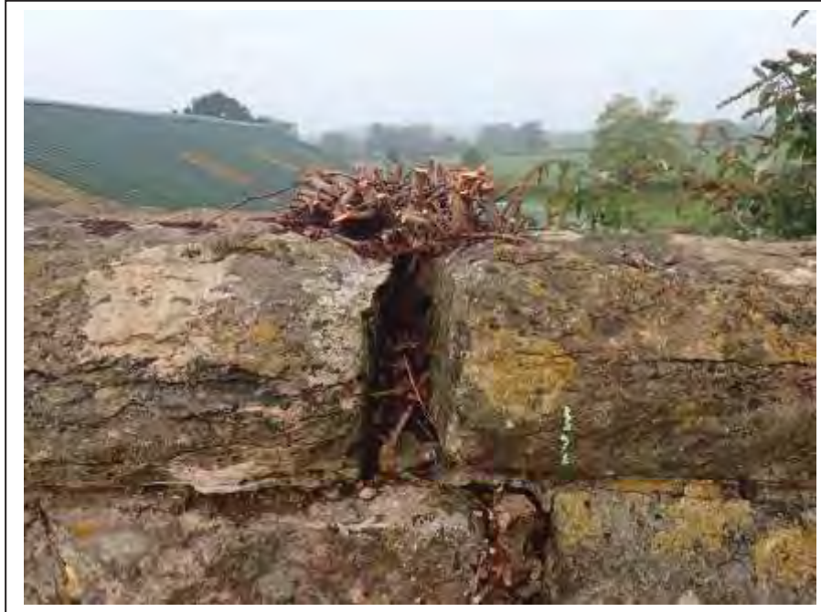
Photograph no 67: root ingress at the coping joint results in fracture open to 75mm
