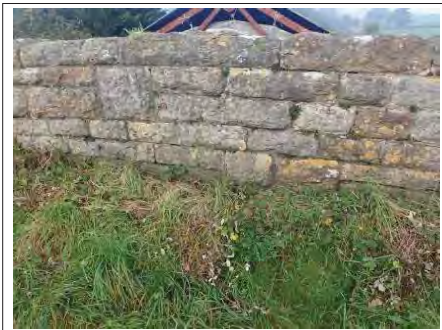
Photograph no 72: odd areas of joint loss within the remaining area of the C/e parapet
