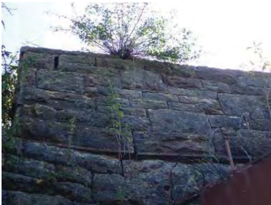
Photograph 40: long-standing loose and displaced stonework is noted within the external face of the C/e parapet at the U/S quoin
