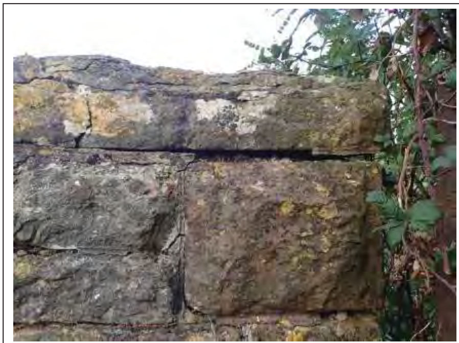
Photograph no 76: deep joint loss noted to full width of the coping at the U/S quoin of the C/e parapet
