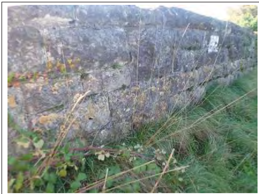
Photograph no 12: lifting and cracking mortar content with odd stones found to move on hammer within the L/e parapet
