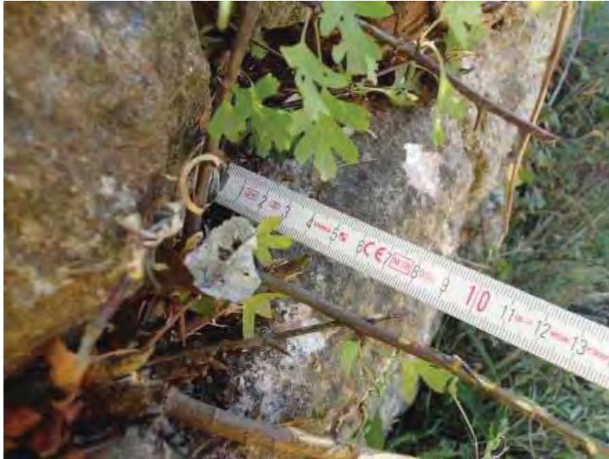
Photograph 27: long-standing inward displacement of the copings was noted up to 60mm
