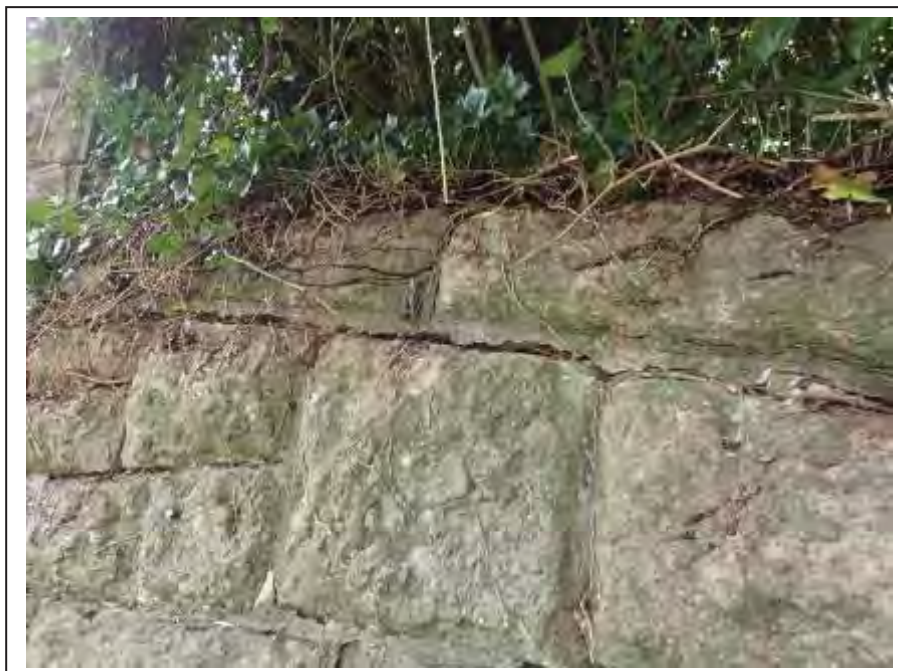
Photograph no 32: remaining copings to upper section of the U/S, L/e wingwall bed fractured to 20mm
