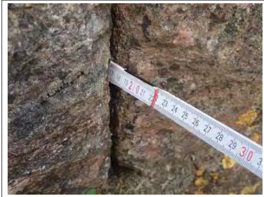
Photograph no 73: joint loss within the internal face of the C/e parapet noted up to 180mm
