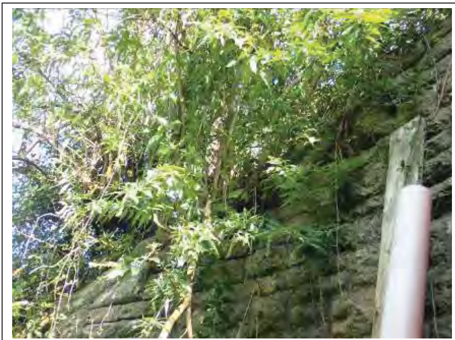
Photograph no 14: example of long-standing root ingress along the rake line of the U/S, C/e wingwall
