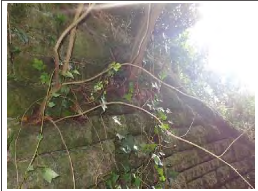
Photograph no 45: example of root ingress within the upper sections of the D/S, C/e wingwall
