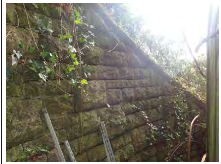
Photograph no 43: example of joint loss within the D/S, C/e wingwall
