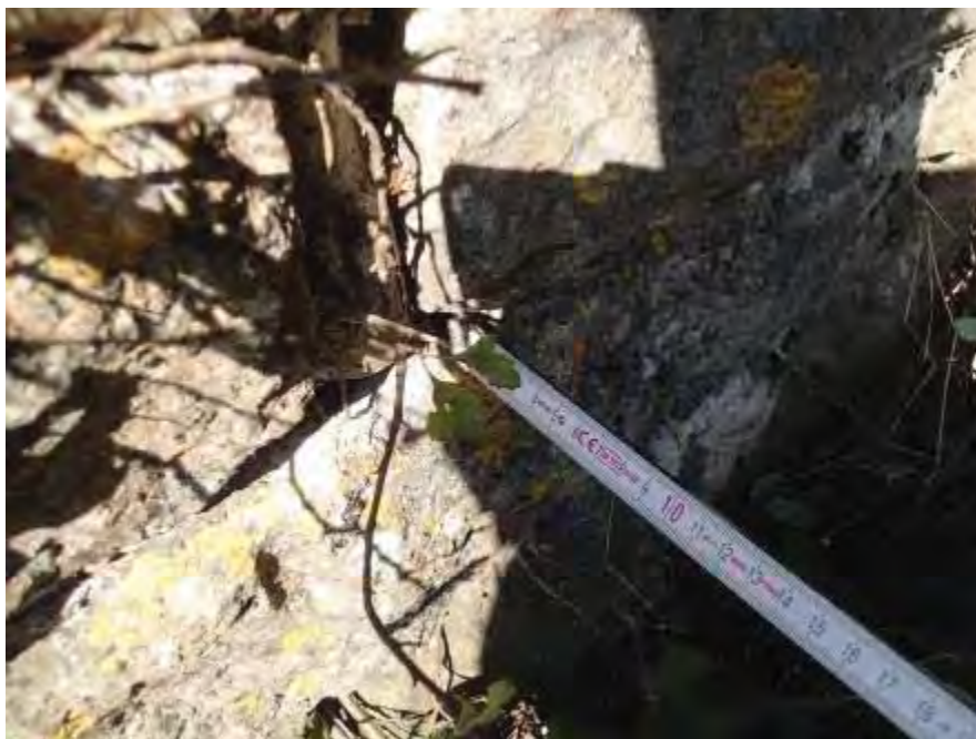
Photograph 34: displacement within the C/e parapet noted up to 20mm
