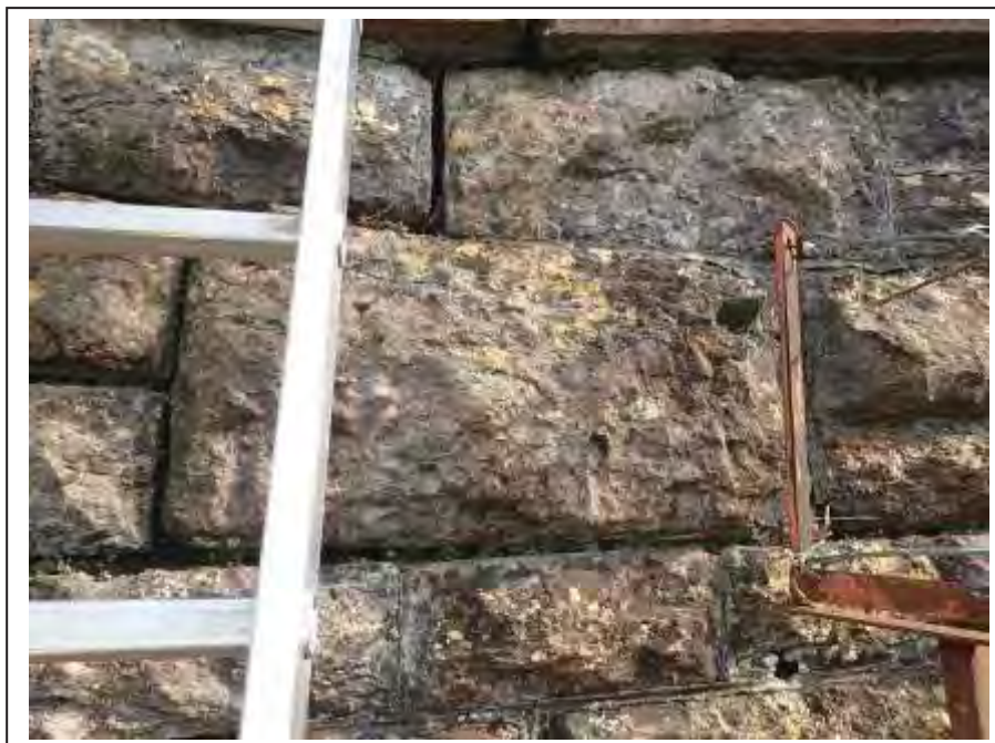
Photograph no 26: example of joint loss within the C/e spandrel U/S of the spandrel shown
