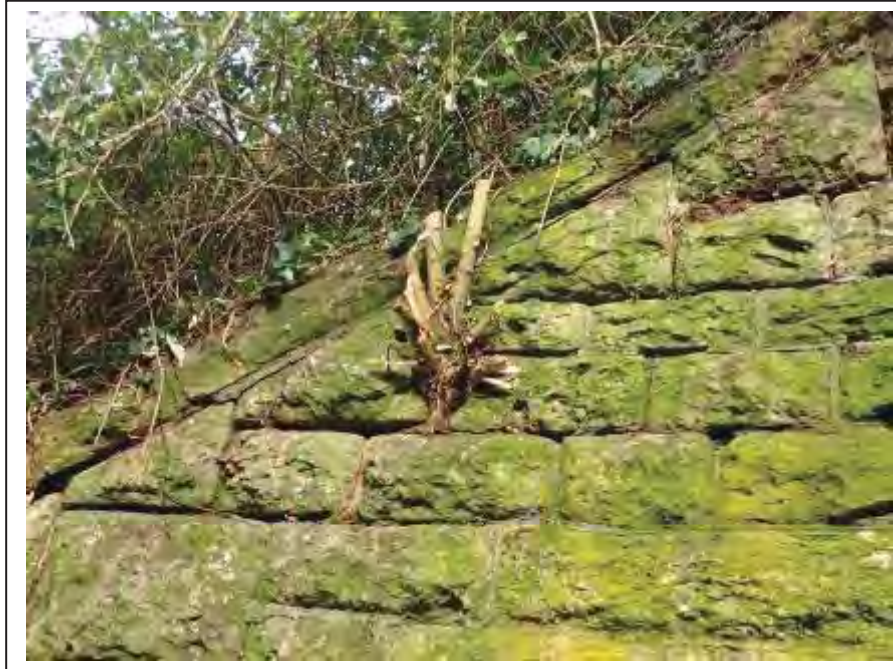
Photograph no 37: root ingress located approx 3.8m from the toe end of the U/S, C/e wingwall
