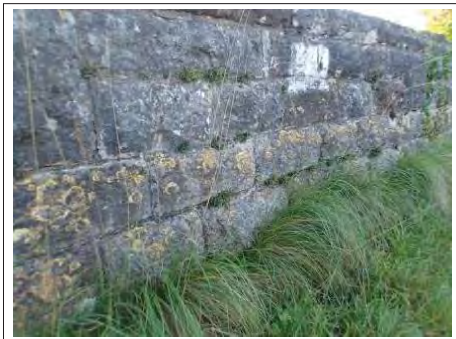
Photograph no 6: lifting and cracking mortar content with odd stones found to move on hammer within the L/e parapet
