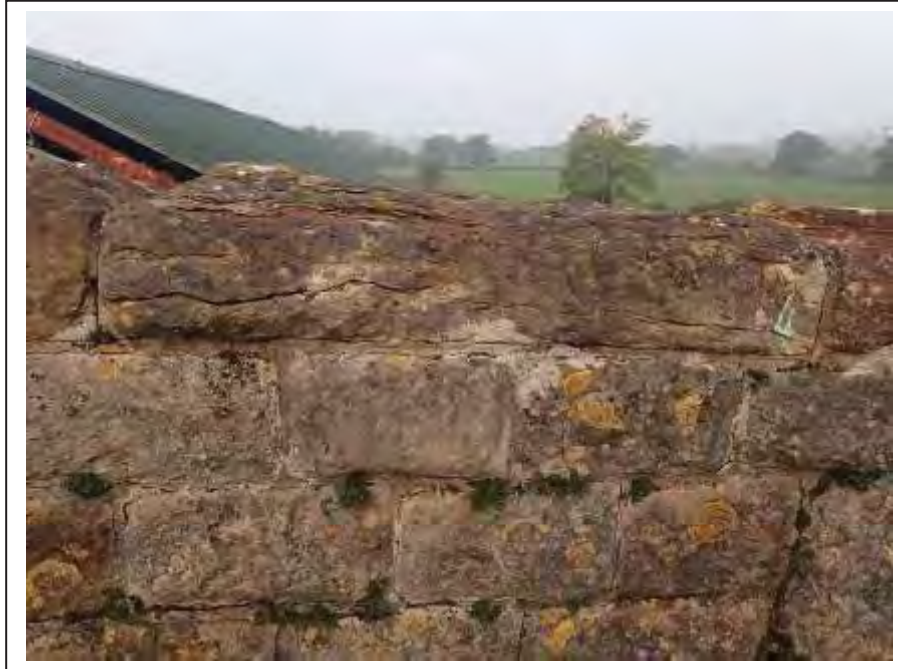
Photograph no 75: example of grain fractures within the C/e parapet copings
