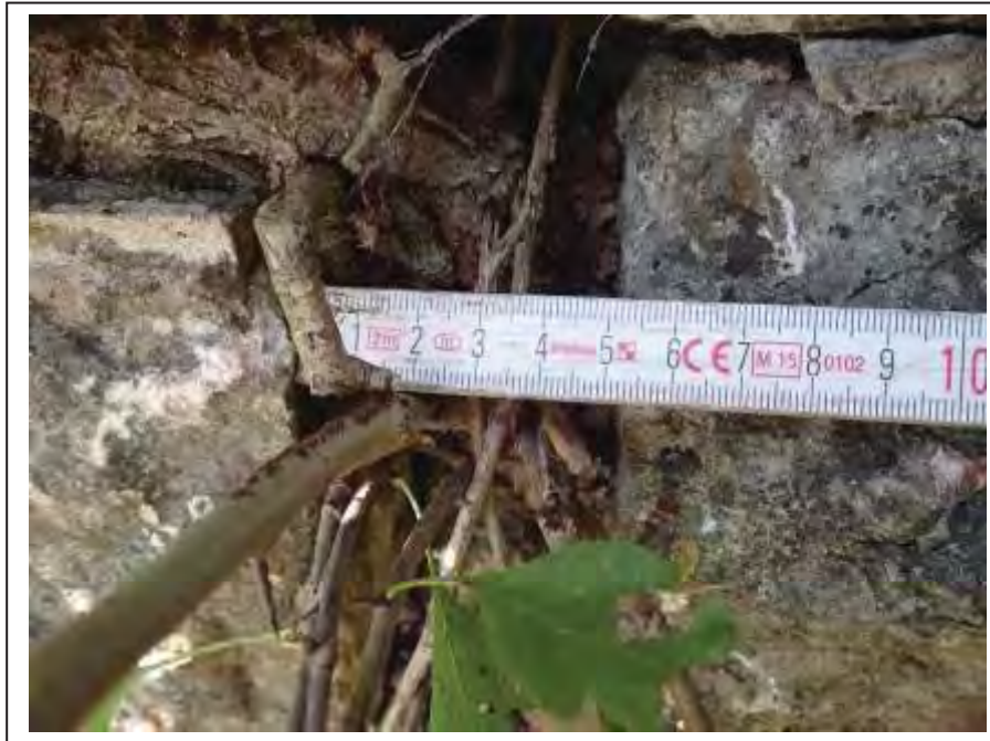
Photograph no 19: fracture open to 50mm within the C/e parapet
