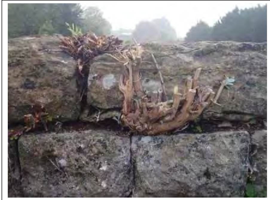
Photograph no 53: root ingress below the L/e copings approx 2.6m from the U/S quoin
