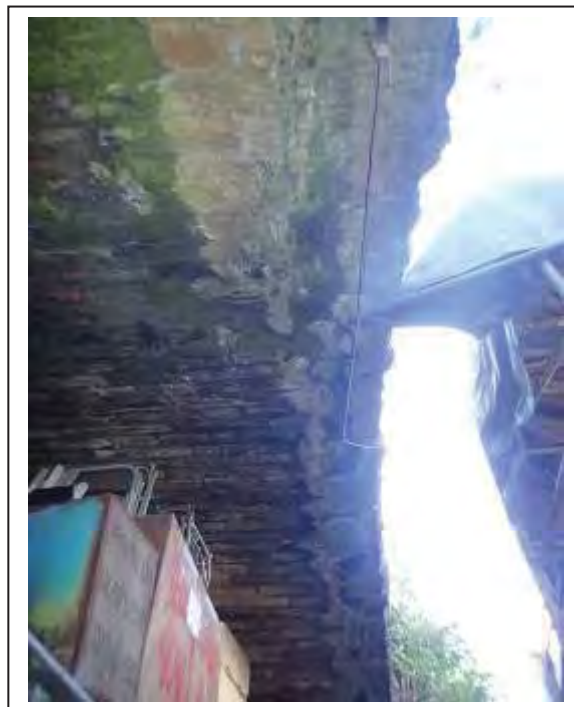
Photograph no 6: calcite deposits to the rear of the C/e voussoirs may cover an underlying fracture.
