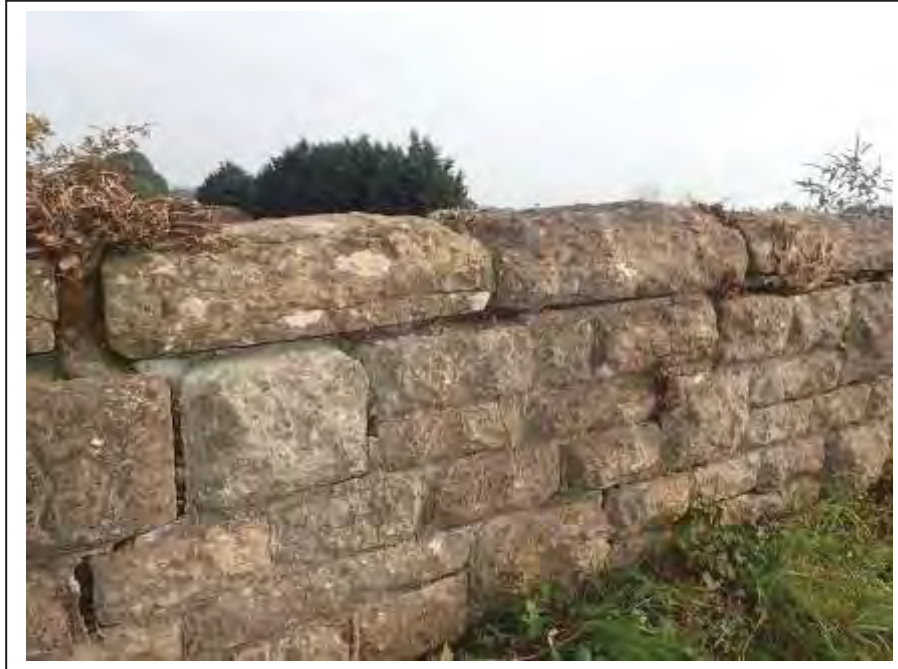
Photograph no 55: long-standing root ingress noted within the perp joints and along the coping bed of the L/e parapet
