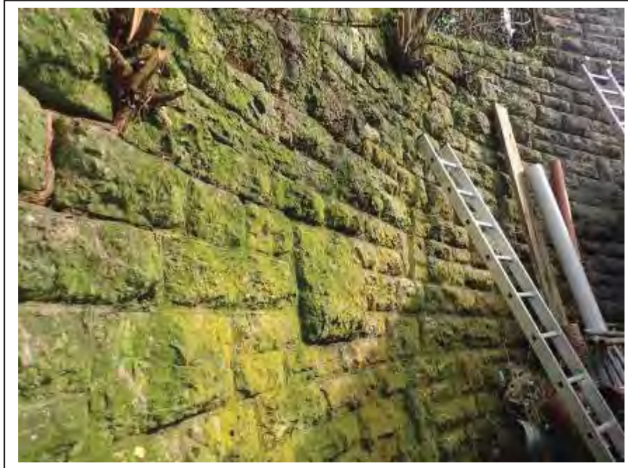
Photograph no 35: example of joint loss within 1m of the copings noted along the U/S, C/e wingwall
