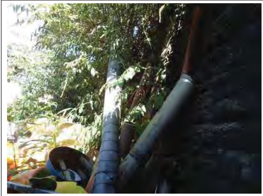
Photograph no 23: vegetation and stored items at the U/S, C/e wingwall restrict the examination.
