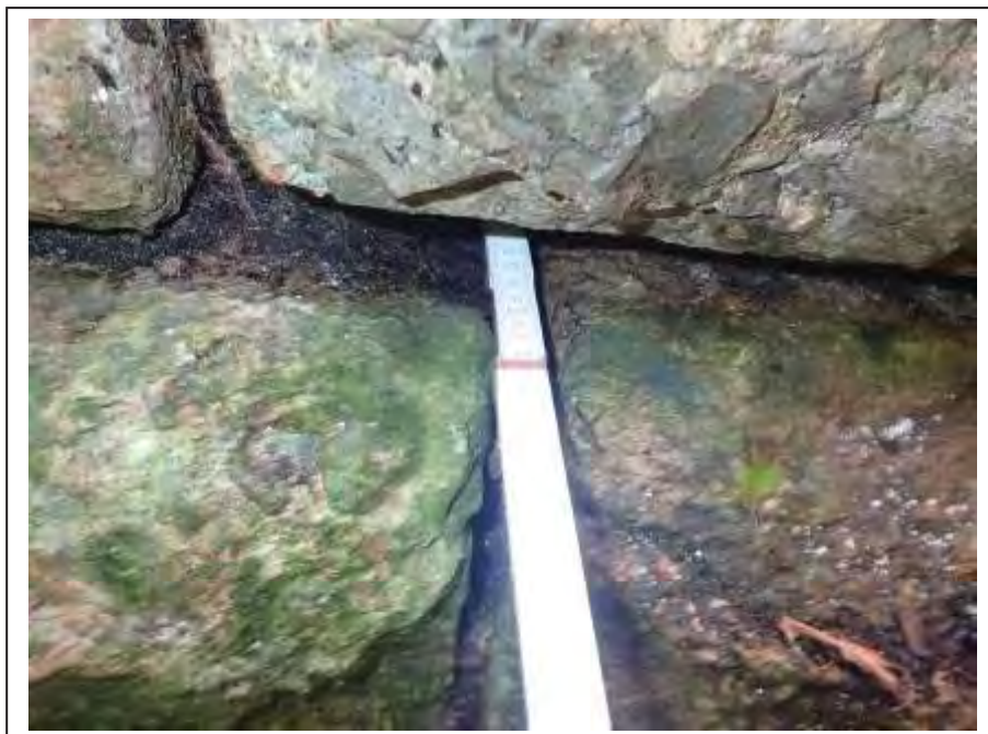
Photograph no 44: joint loss within the D/S, C/e wingwall noted up to 220mm
