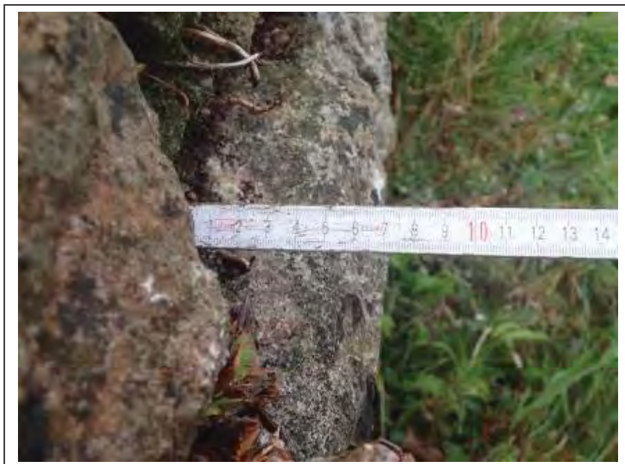
Photograph no 54: root ingress at 2.6m results in inward displacement of the copings up to 60mm
