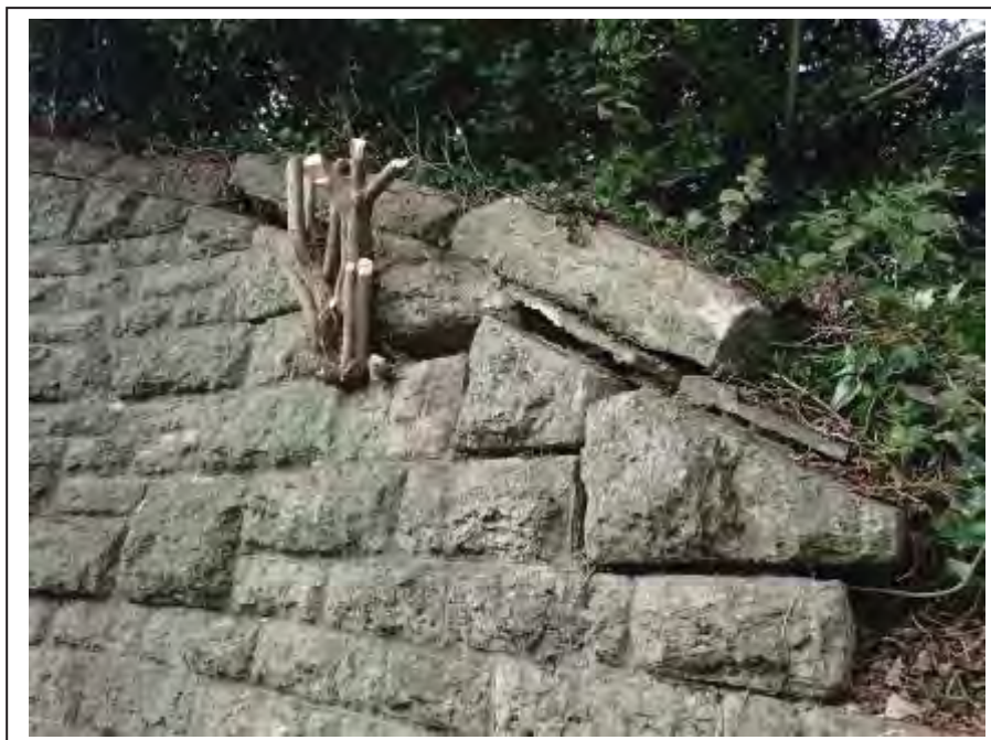
Photograph no 30: root ingress within the U/S, L/e wingwall displaces cut stones and copings.
