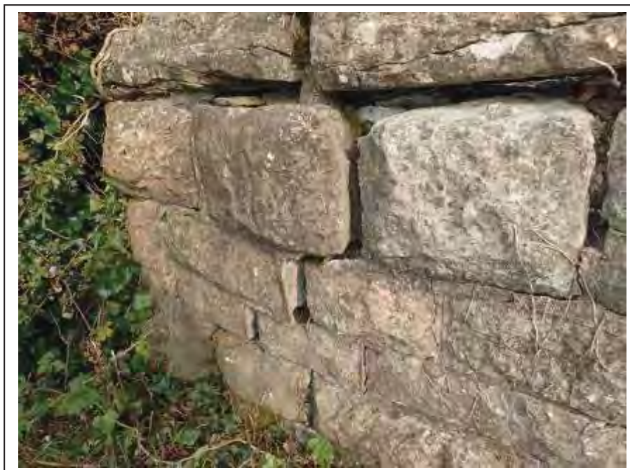
Photograph no 48: long-standing fracturing and displacement at the U/S quoin of the L/e parapet
