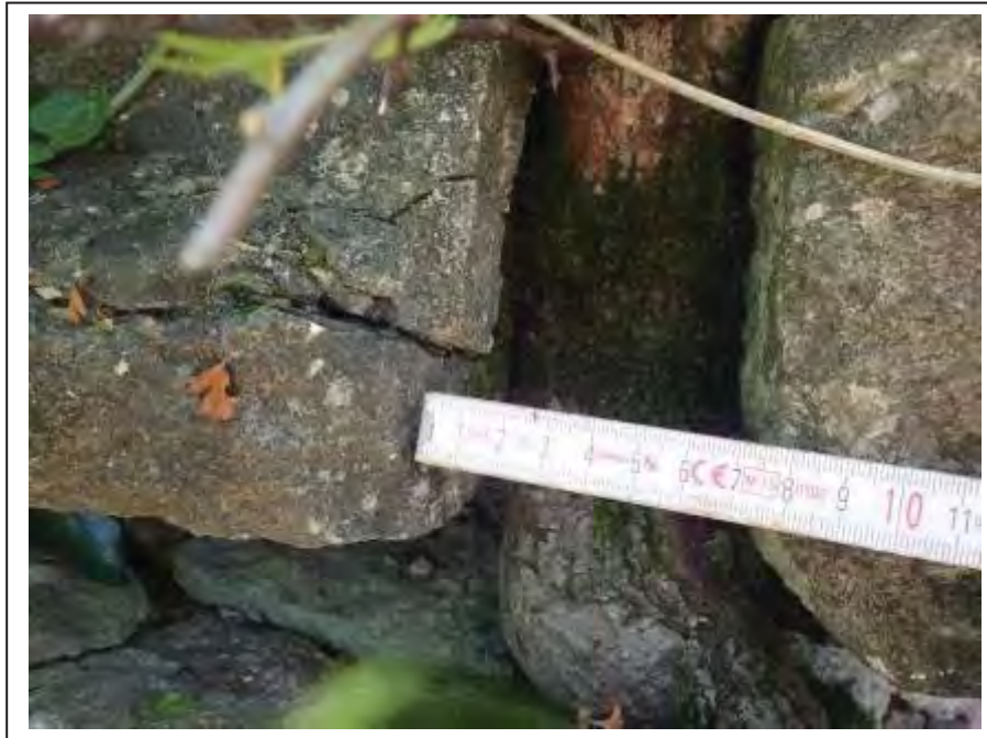
Photograph no 15: displacement at the coping noted up to 70mm
