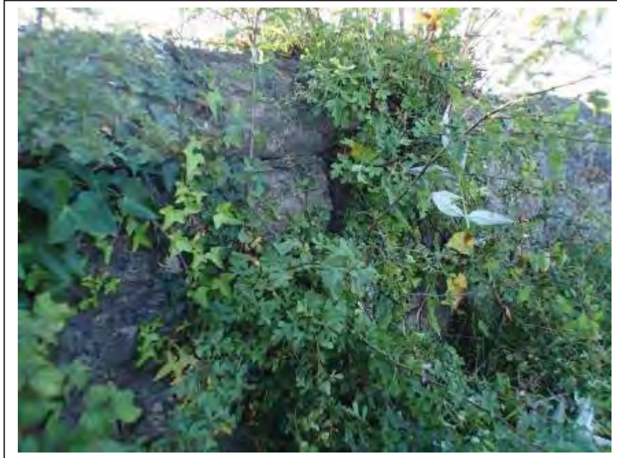
Photograph no 5: lifting copings noted along the L/e parapet due to root ingress approx 2.7m from the U/S quoin
