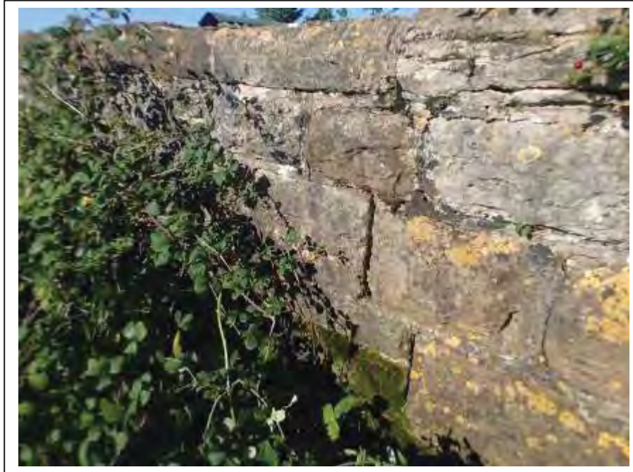
Photograph no 15: odd areas of mortar loss with odd stones found to move on hammer within the C/e parapet
