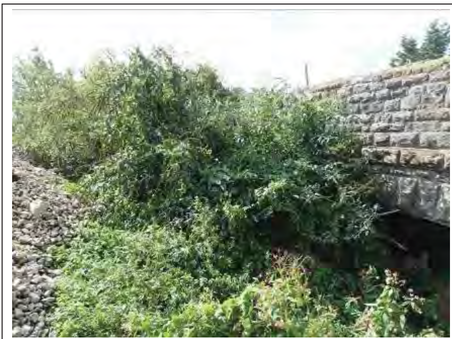
Photograph no 6: access to the D/S, L/e wingwall was restricted due to vegetation growth
