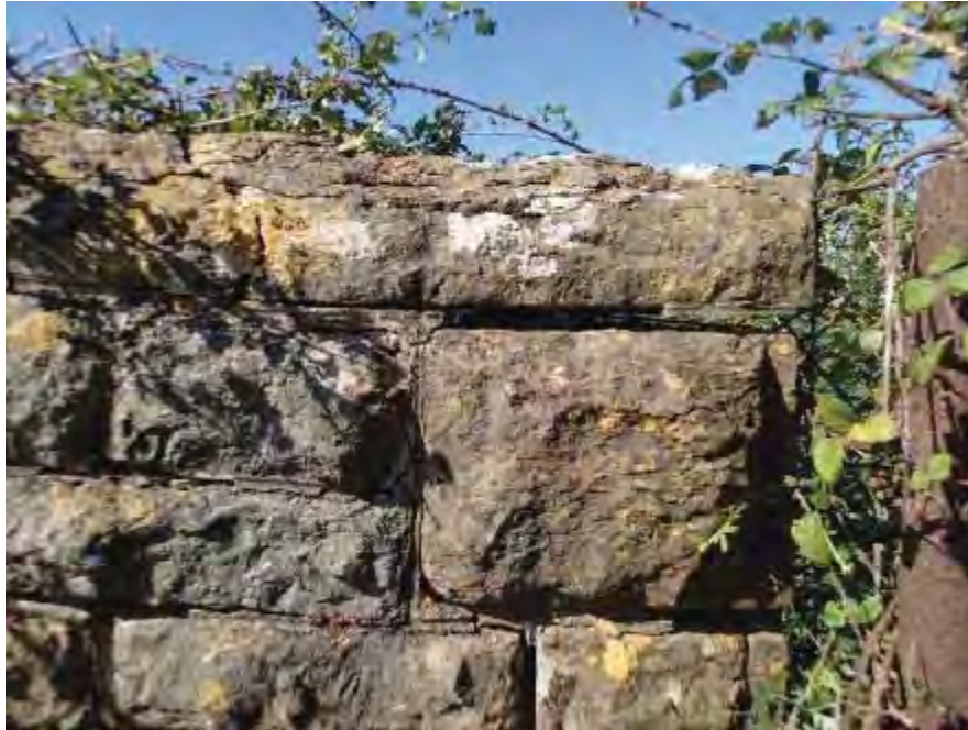
Photograph 41: fractured and loose coping is noted at the U/S quoin of the C/e parapet
