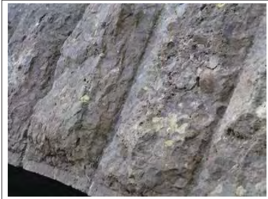
Photograph no 17: example of surface erosion within the L/e voussoirs
