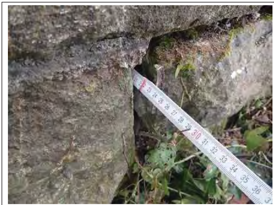
Photograph no 52: joint loss within the L/e parapet noted up to 220mm
