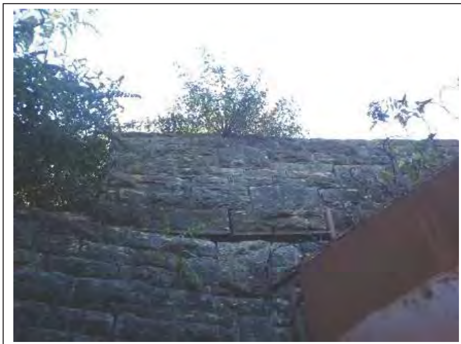
Photograph no 14: long-standing step fracture visible to the external face of the C/e parapet on the U/S Associated pushing stonework noted to approx 15mm
