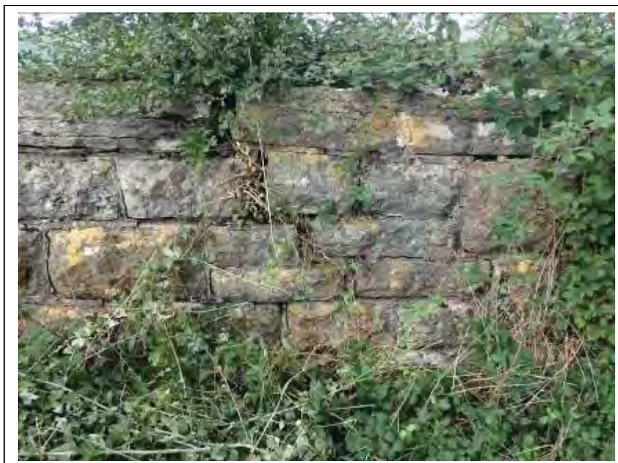
Photograph no 20: long-standing root ingress noted along the copings and within the C/e parapet towards the U/S quoin
