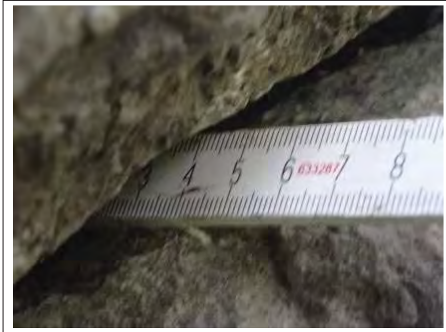
Photograph no 19: example of joint loss noted along the extrados joint on the L/e up to 50mm
