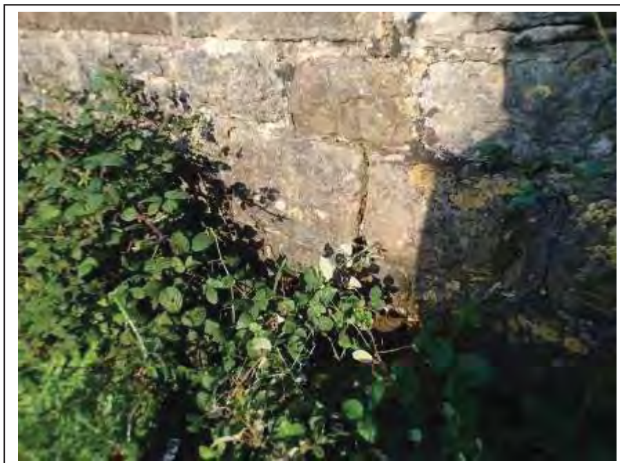
Photograph no 8: odd areas of mortar loss with odd stones found to move on hammer within the C/e parapet
