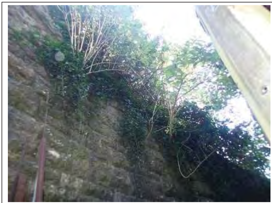
Photograph no 20: vegetation and sapling growth to the face of the D/S, C/e wingwall
