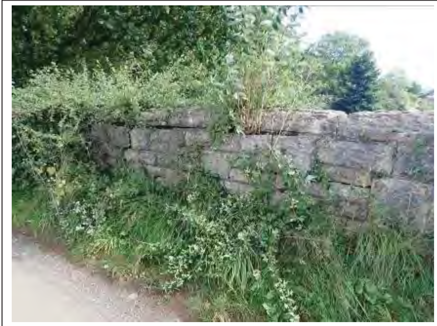
Photograph no 17: long-standing root ingress noted along the copings and within the L/e parapet towards the U/S quoin
