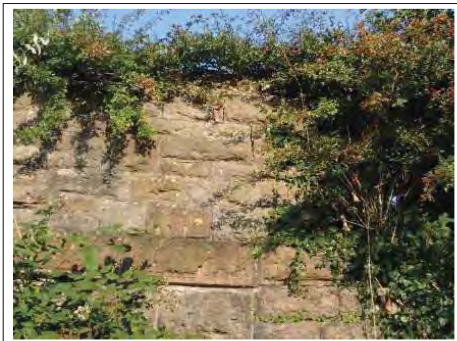
Photograph no 4: fracturing noted towards the U/S quoin of the L/e parapet within the external face
