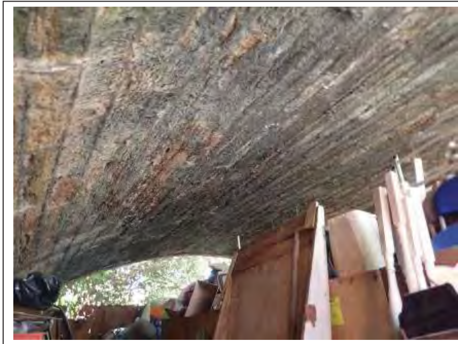
Photograph no 11: odd spalled stones noted within the soffit
