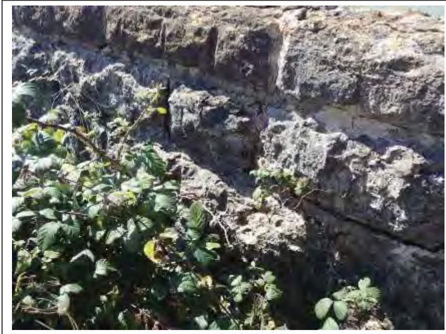
Photograph no 21: odd stones found to move under hammer within the C/e parapet
