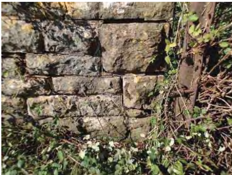
Photograph 36: step fracture at the U/S quoin within the C/e parapet
