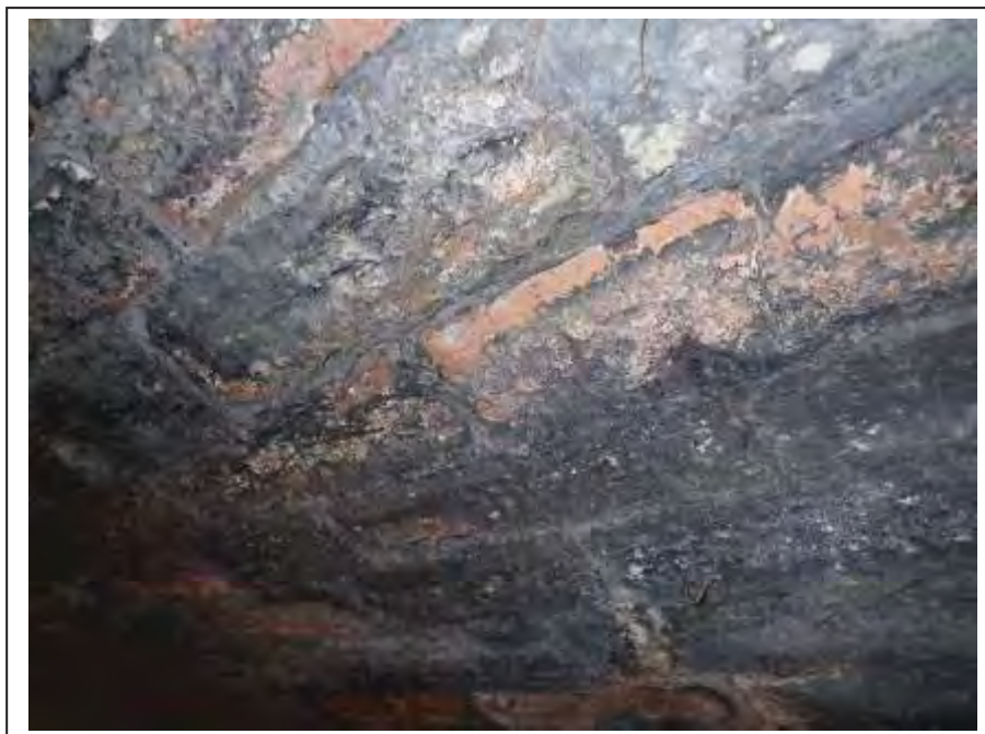
Photograph no 22: example of spalling noted within the soffit.
