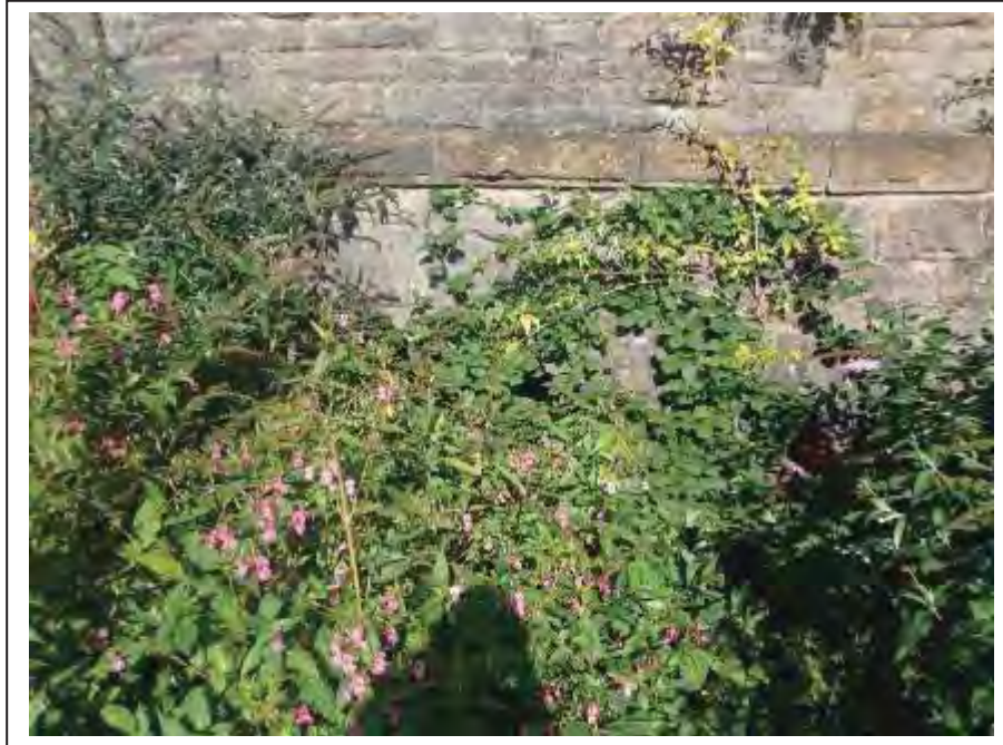
Photograph no 5: vegetation restricts full inspection of the L/e voussoirs. Evidence of long-standing joint loss noted at the extrados joint
