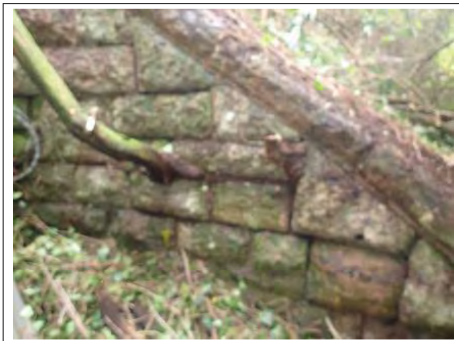
Photograph no 46: example of root ingress towards the toe end of the D/S, C/e wingwall
