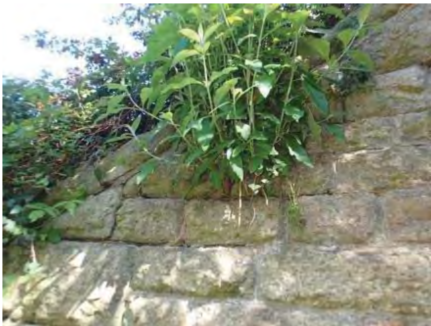
Photograph 16: example of root ingress located along the rake line of the U/S, C/e wingwall
