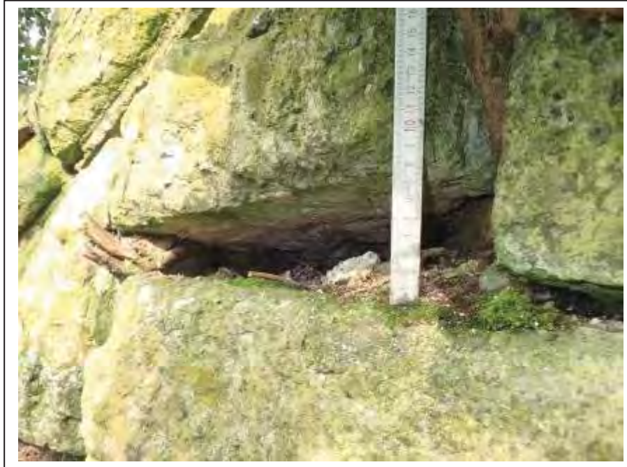
Photograph no 39: lifting stones noted up to 80mm at the root ingress at 1.9m
