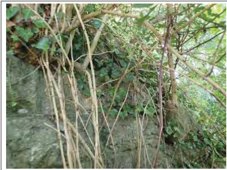
Photograph no 10: some displaced copings at cut stones noted along the U/S, L/e wingwall
