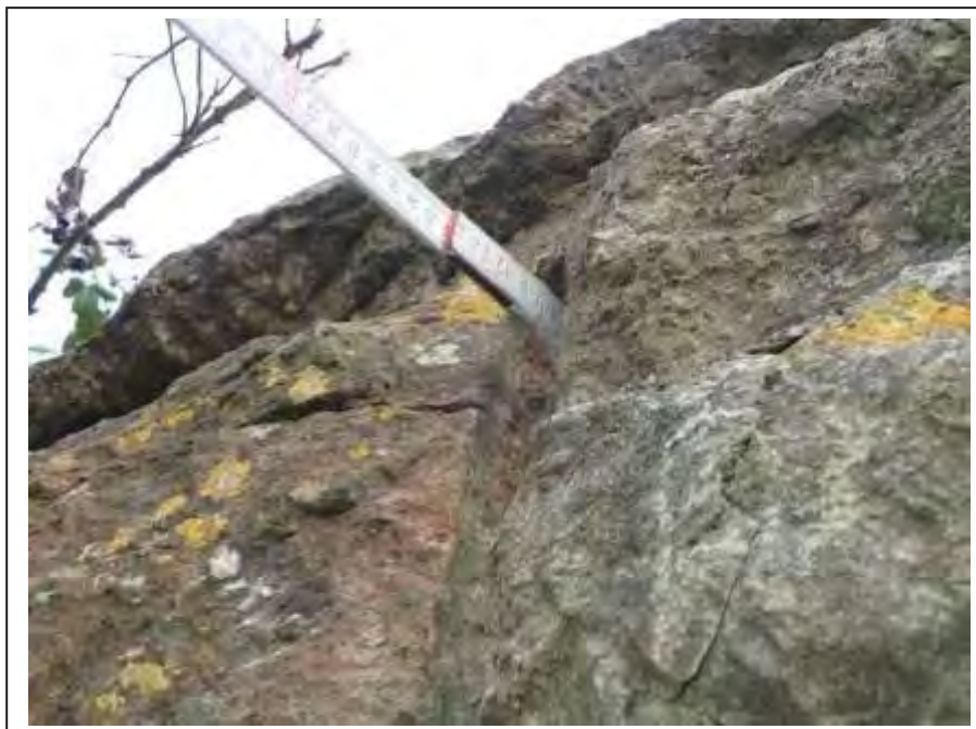
Photograph no 80: joint loss within the external face of the C/e parapet noted up to 180mm
