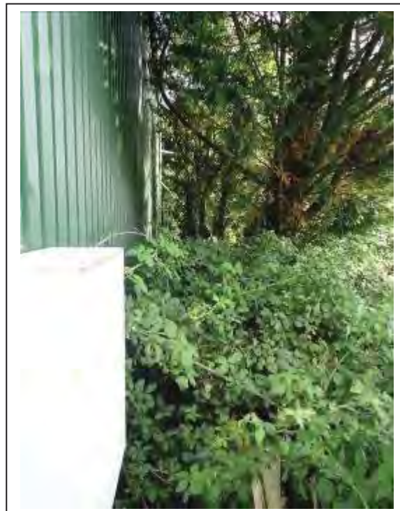
Photograph no 16: access to the toe end of the D/S, C/e wingwall was restricted due to dense vegetation
