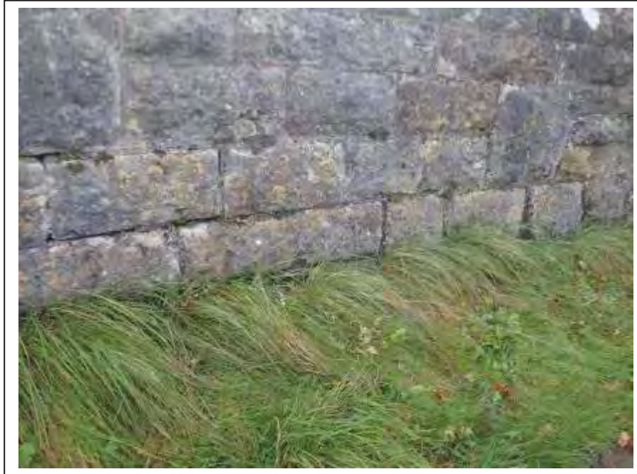
Photograph no 51: example of odd areas of joint loss within the remaining area of the L/e parapet
