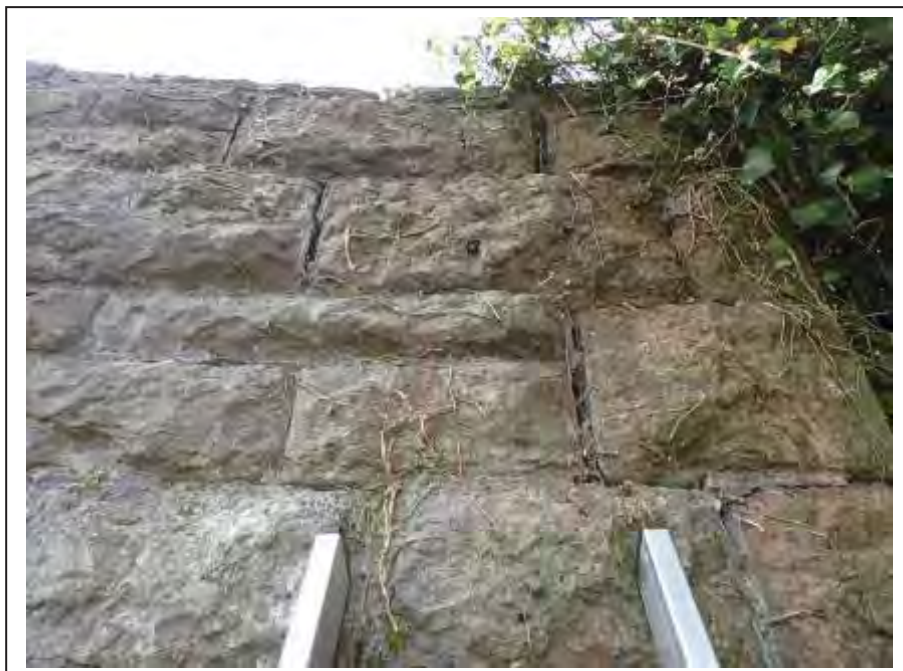
Photograph no 58: step fracture to the external face of the L/e parapet at the U/S quoin
