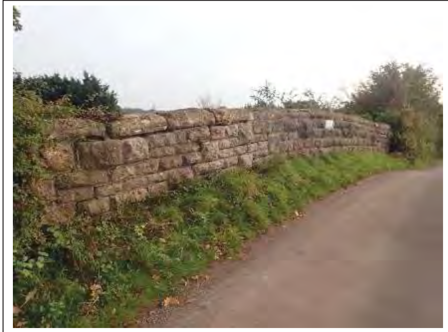
Photograph no 11: internal face of the L/e parapet
