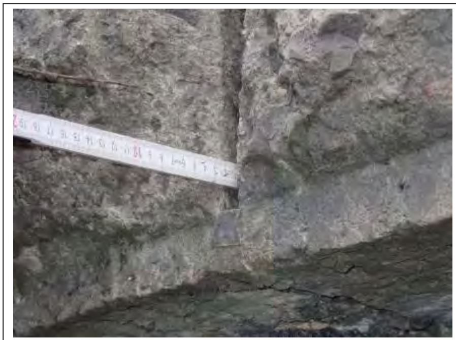
Photograph no 18: example of joint loss noted to individual perp joints within L/e voussoirs
