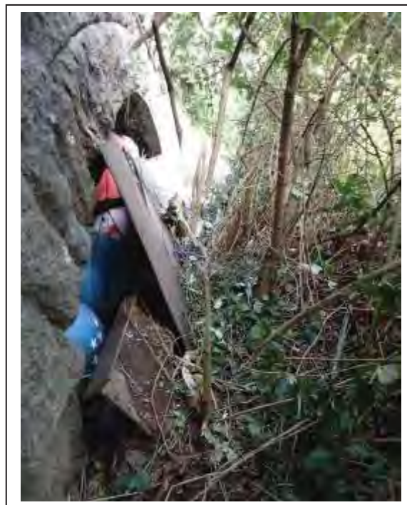
Photograph no 16: poor access encountered on the L/e of the structure Please note: the vegetation could not be cleared back from the face of structure any further due to concerns of disturbing the Himalayan Balsam encountered on site.
