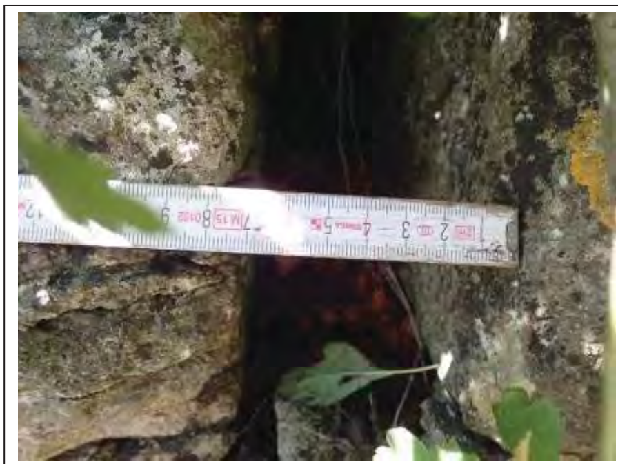
Photograph no 20: displacement at the coping perp noted to 70mm
