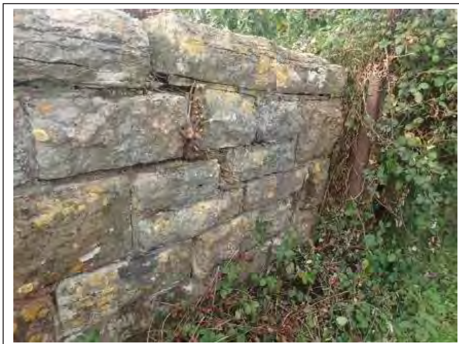
Photograph no 66: long-standing fracture and displacement noted at the U/S quoin of the C/e parapet
