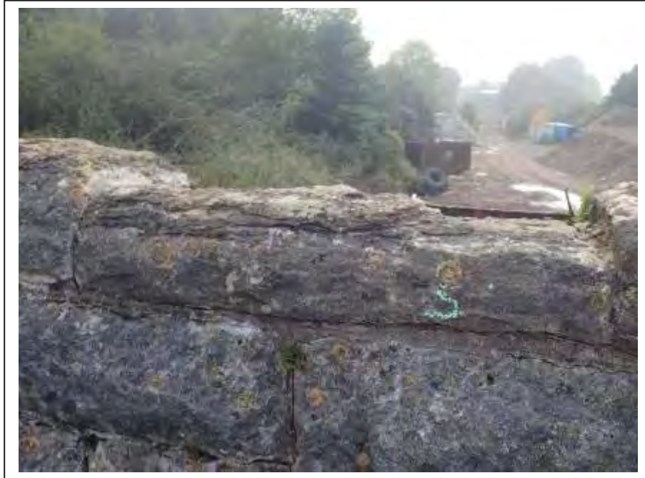
Photograph no 57: a coping upon the L/e parapet is spalled up to 80mm.
