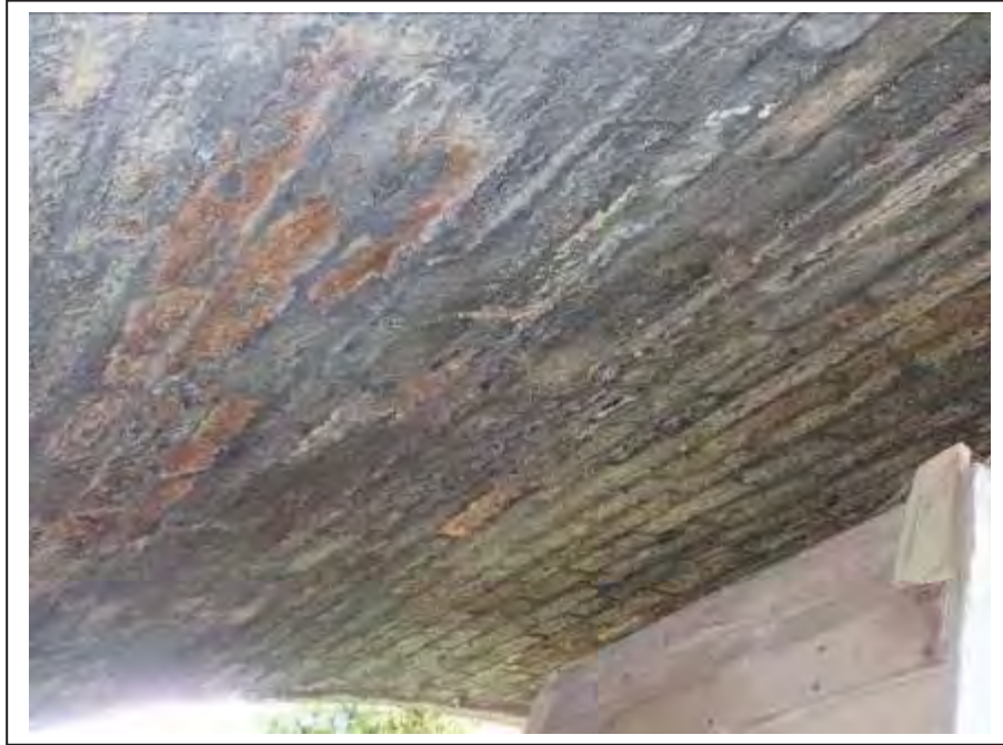
Photograph no 11: example of long-standing spalling action within the soffit
