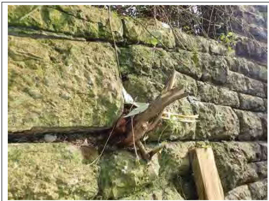
Photograph no 42: root ingress located approx 1.3m from the top of the U/S, C/e wingwall
