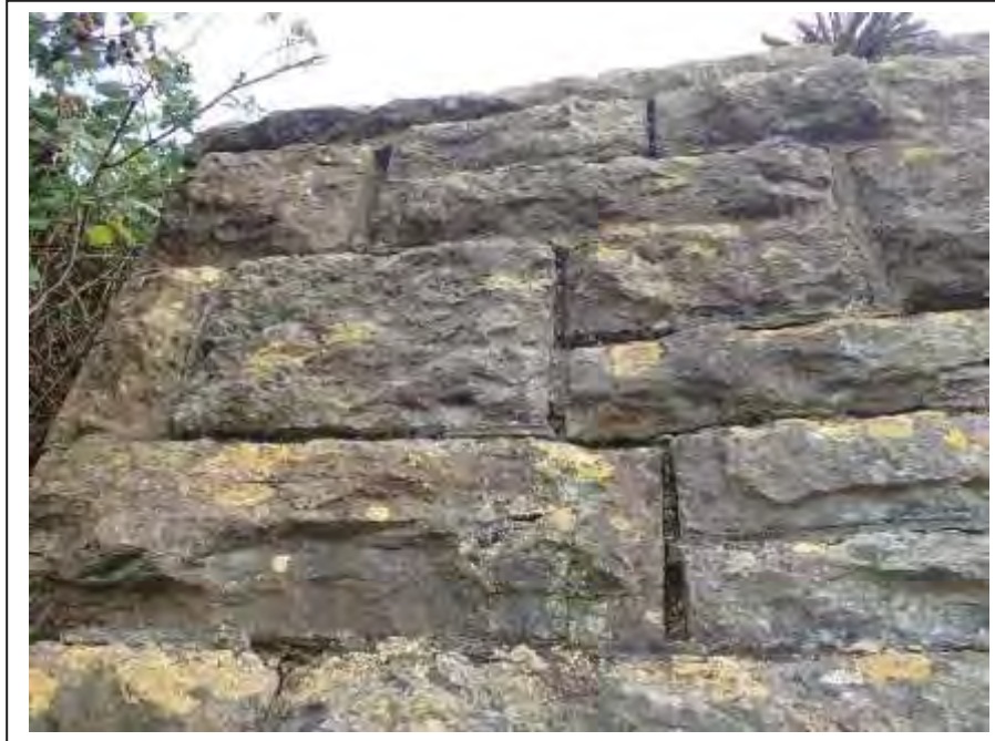
Photograph no 77: example of loose stonework located within 2.2m of the U/S quoin of the C/e parapet External face shown
