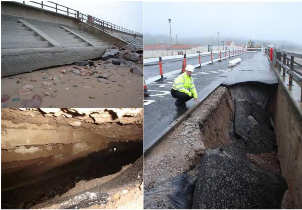
Figure 3.1 Failure of a concrete seawall, due to undermining and washout of backfill in Aberdeenshire, Scotland
